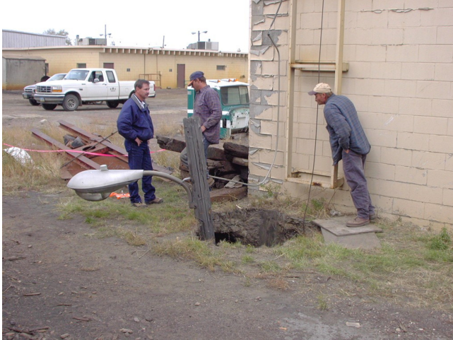
2001 Lehigh Emergency, sinkhole beneath commercial building.
