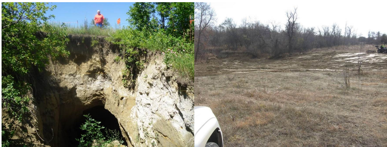
Before and after photos of sinkhole filling at Dave & Cathy Zimmerman property, Richardton, ND
