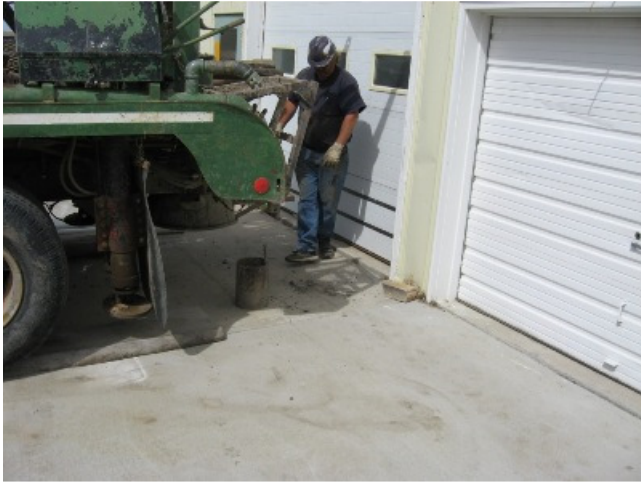
2008 Williston (David Njos) Emergency, drilling & grouting underneath a commercial building with voids directly underneath the floor.
