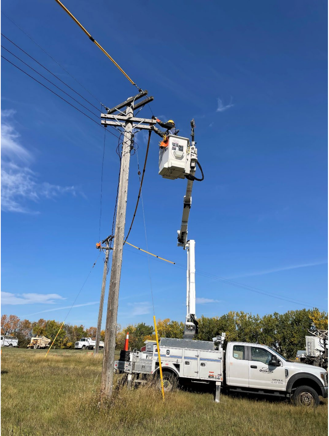
Figure 8: The power company covered the lines to allow safe drilling near these powerlines. Drilling confirmed these poles are undermined.
