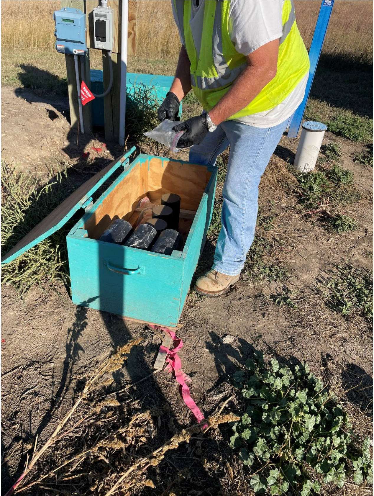
Figure 5: The material tester is storing grout samples for field curing. Once cured, they will be tested for strength.
