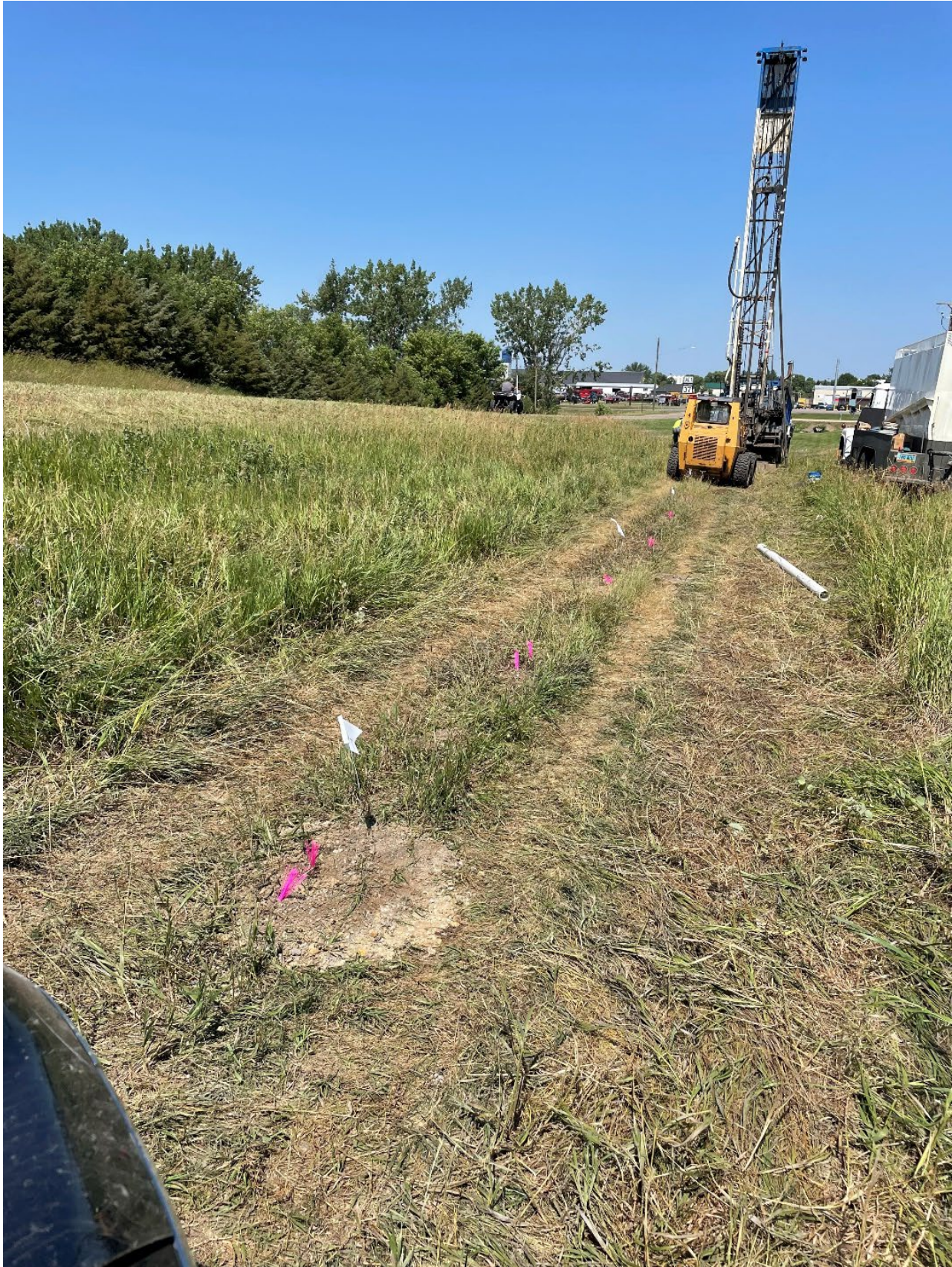
Figure 2: The drilling rig is moving north in the east right of way of McLean County Highway 15 as part of the 2022 Exploratory Drilling AML Project. The pink markers indicate a hole was cased.
