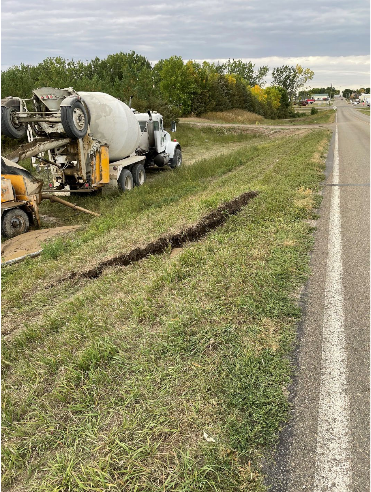
Figure 6: Surface lifting often occurs when a mine void is filled with grout. The grout will find the path of least resistance.
