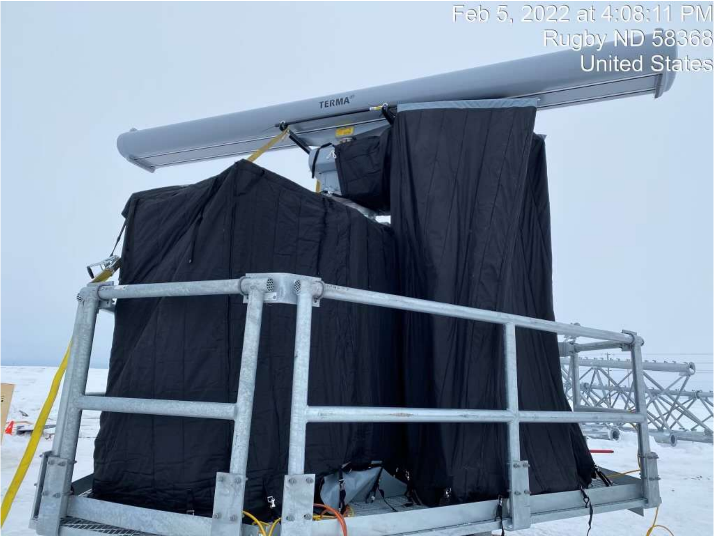
Rugby ADLS radar unit with enclosure on ground.
