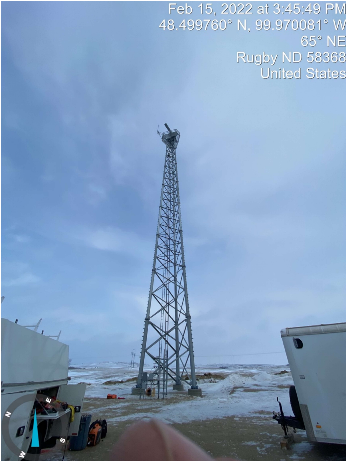
Rugby ADLS lattice tower with installed radar unit.
