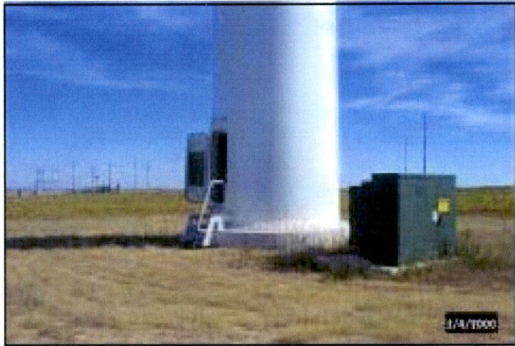
Pad Transformer at Base of Turbine
