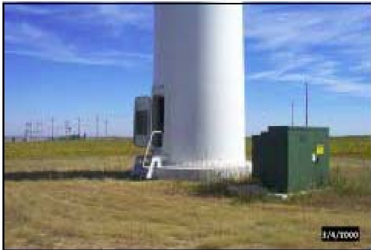
Pad Transformer at Base of Turbine
