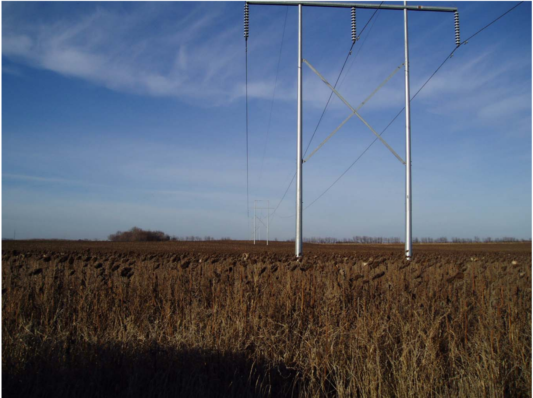
Figure 10. Existing Environment Rugby Wind Farm : 230 kV Transmission Line Pierce County, ND
