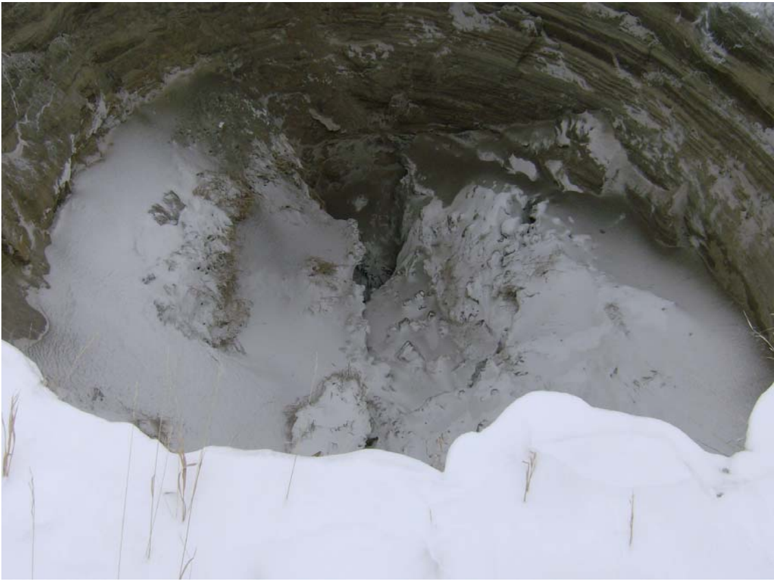
SN 358+30 Sink hole looking into hole
