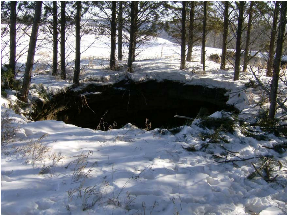
SN 362+50 looking SE, Sinkhole near ROW centerline in pine plantation 2009-01-29
