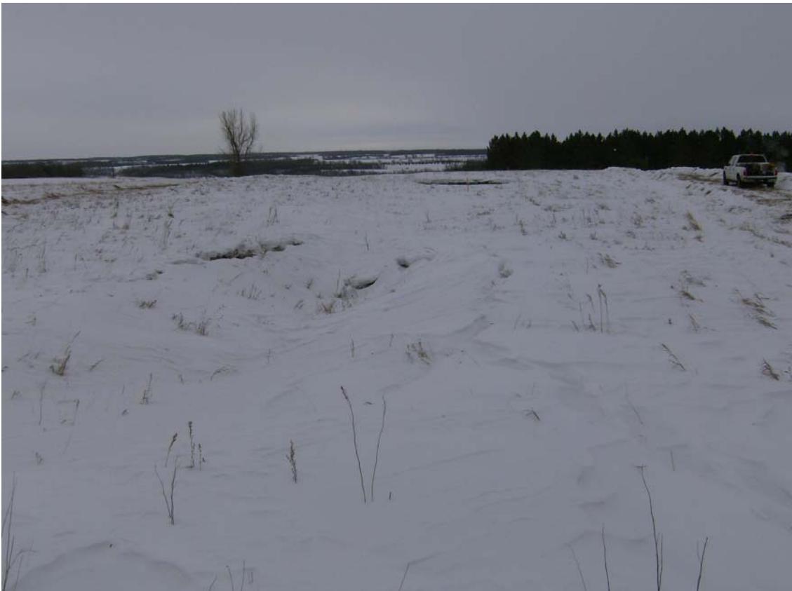
SN 356+50 Subsidence over ditch line looking south
