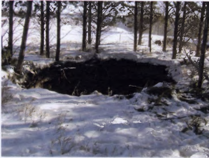
Sinkhole near ROW centerline in pine plantation. View is to the southeast
