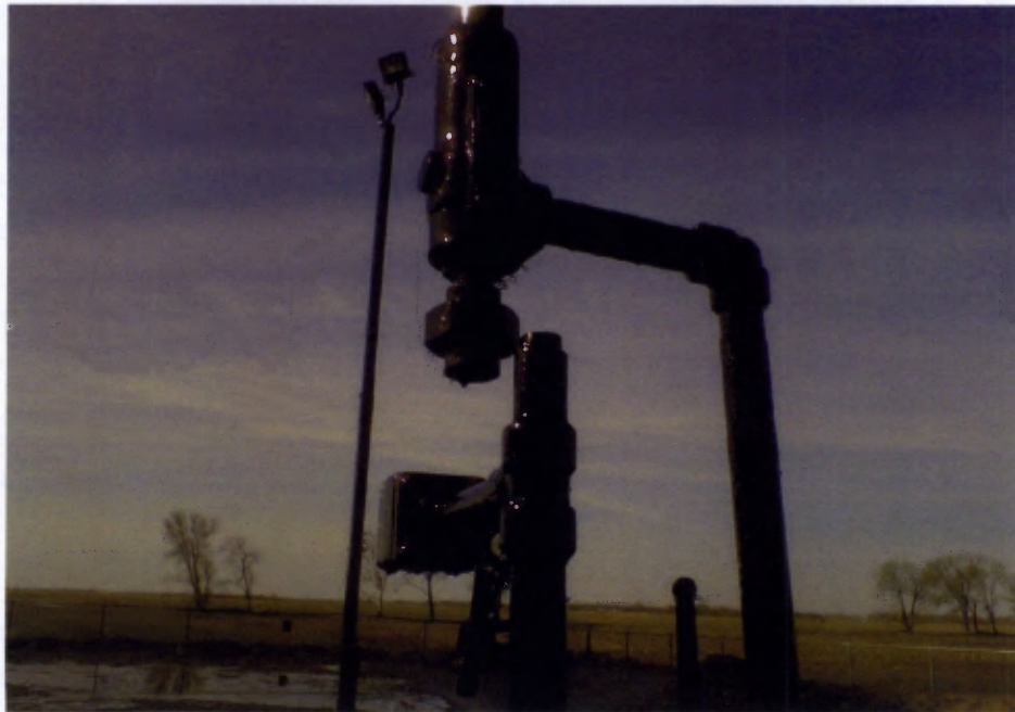
Figure 2 Failed Assembly as Found
