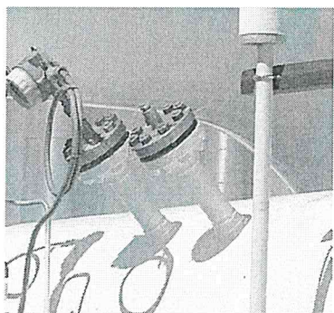
2 Thermo wells – Before
