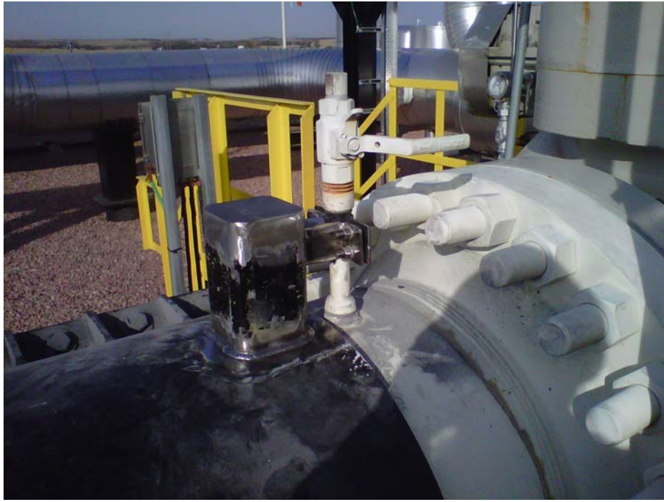
Unit Suction Line Vent Bracing
