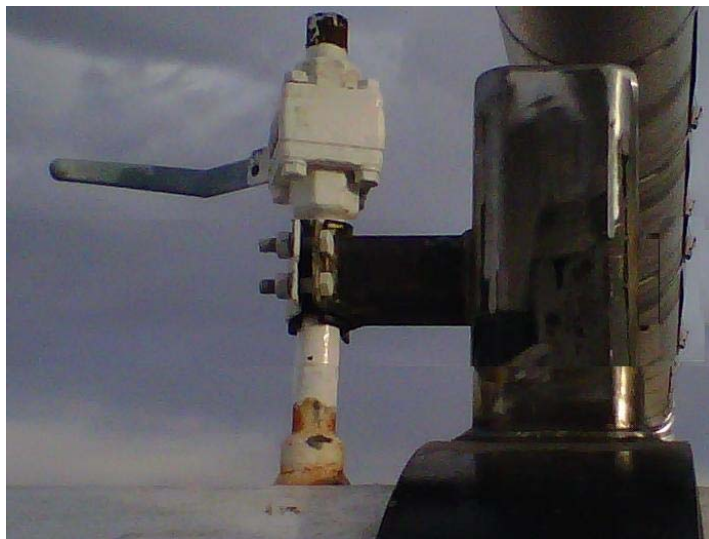
VFD Unit High Point Vent Bracing
