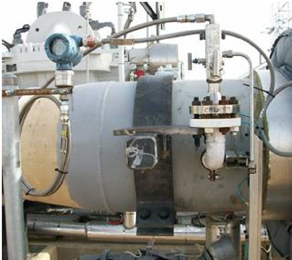
Pressure Transmitter Nozzle Brace
