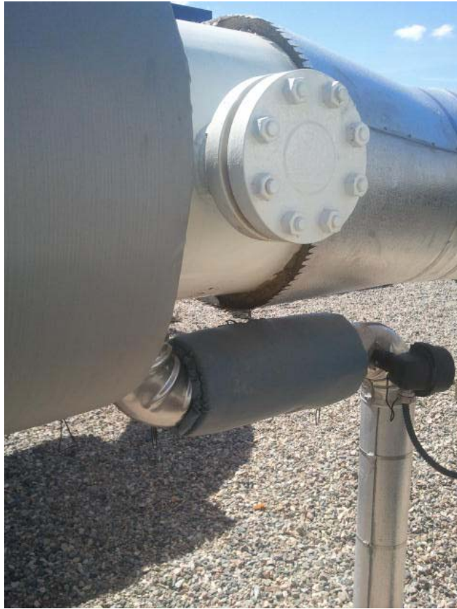
Unit Discharge Drain Line
