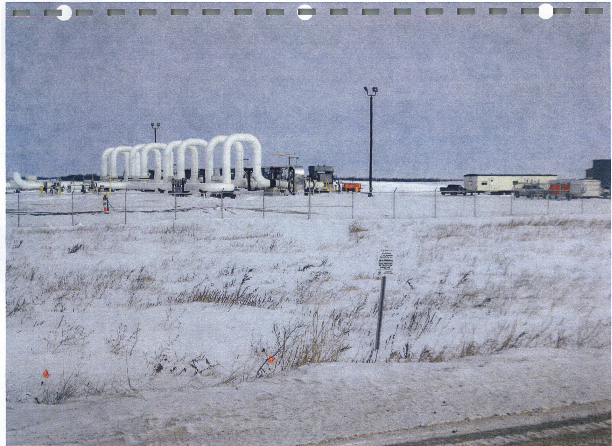
Picture # 58 Pump station 3rd one 11th St SE
