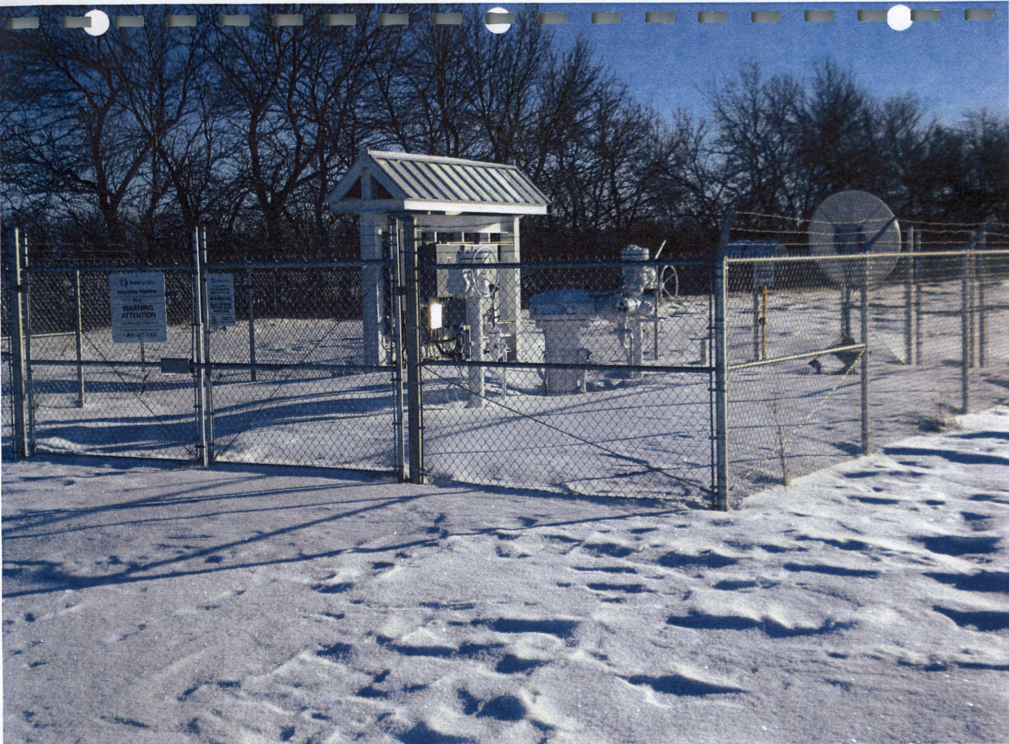
Picture #21 Automatic pressure emergency station mile #15 (2nd one)
