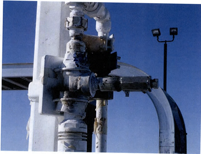
Previous PSV Test Port
