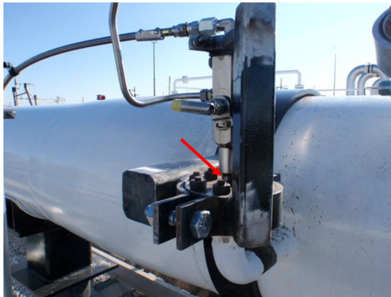
Figure 1. Typical PT-201 & PT-203 nozzle and manifold bracing. The red arrow points to the stress concentration area in the manifold "neck".
