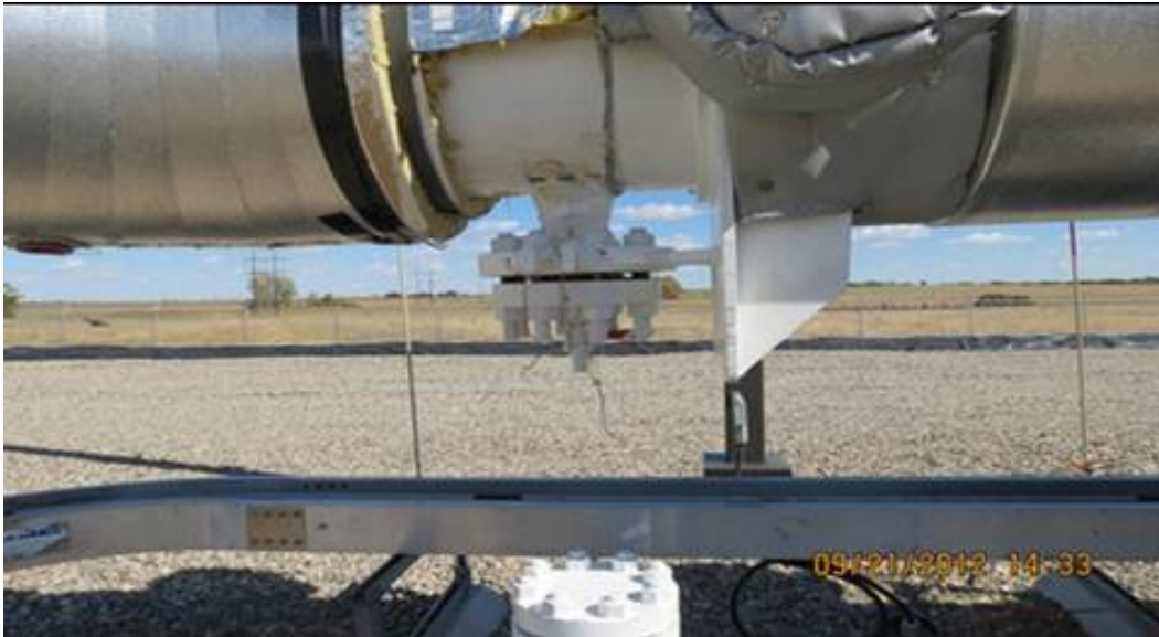
Figure 3: Fort Ransom abandoned station drain upstream from the PCV
