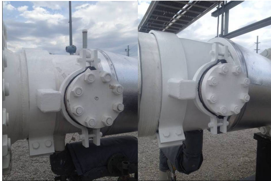
Figure 1: Braced pump #4 discharge MOV bypass nozzles at Severance fixed speed station: upstream from MOV (left) and downstream from MOV (right).
