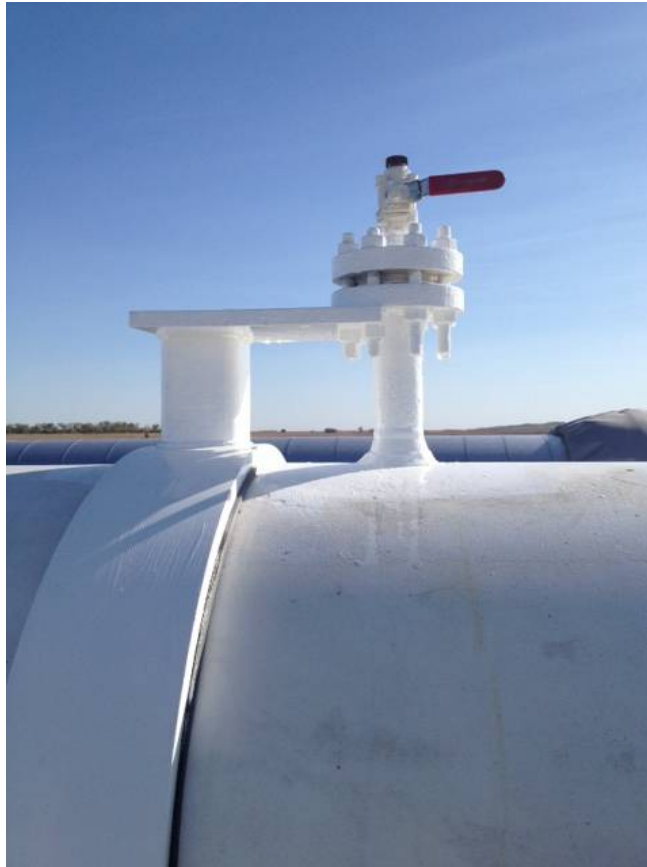
Figure 4: Braced pig launcher vent nozzle at Fort Ransom
