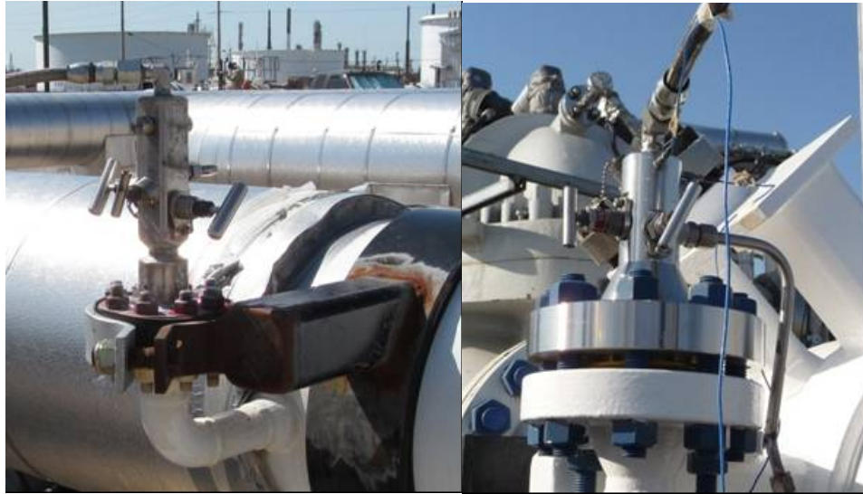
Figure 5: Hartford Delivery Terminal- existing (left) and replacement (right) PT manifolds
