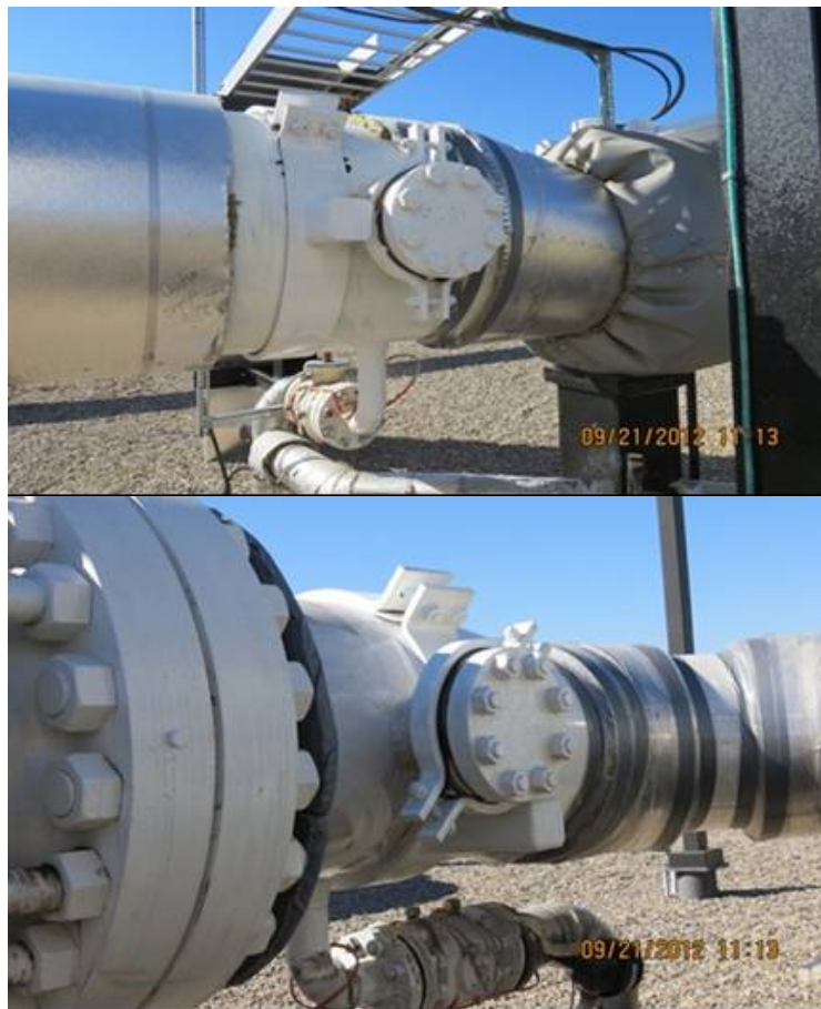
Figure 2: Braced pump #4 discharge MOV bypass nozzles at Fort Ransom fixed speed station: downstream from MOV (top) and upstream from MOV (bottom)
