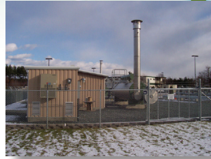
Metering and Regulating Station
