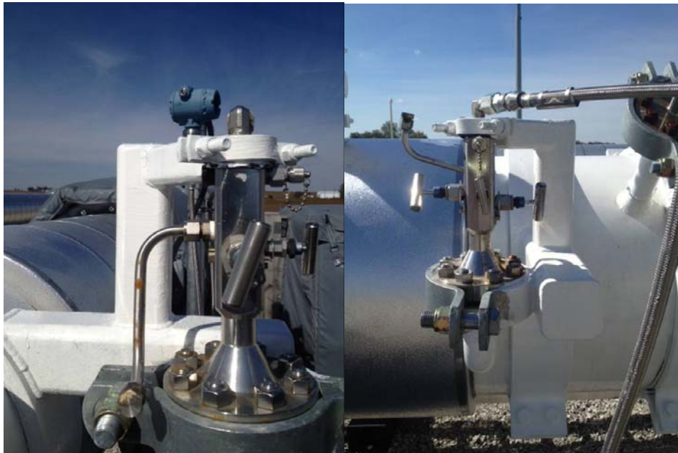
Figure 3: Braced PT201 (left) and PT203 (right) manifolds at Pierron VFD station
