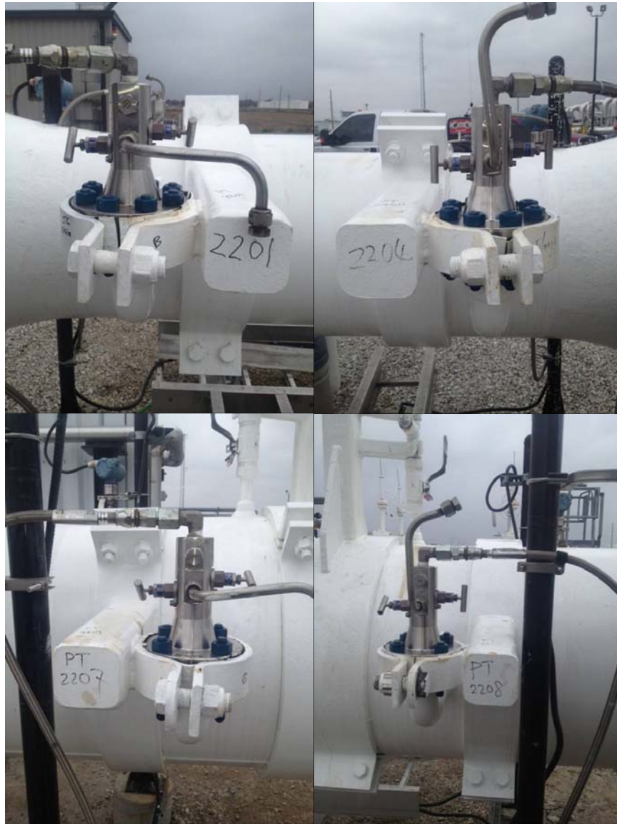
Figure 4: New PT2201, PT2204, PT2207 and PT2208 manifolds at Hartford Delivery Terminal
