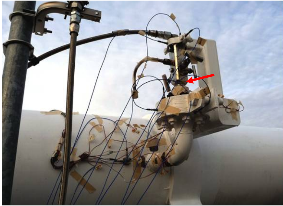
Figure 2: Braced PT201 manifold at Steele City VFD station
