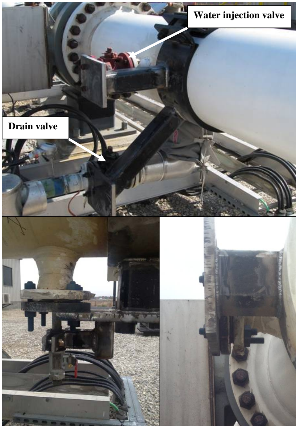
Figure 5: Hartford Delivery Terminal – drain and water injection branch connections: original configuration (top), abandoned drain (bottom left) and abandoned water injection (bottom right)
