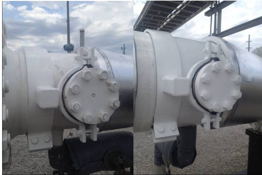
Figure 1: Examples of braced pump #4 discharge MOV bypass nozzles at the fixed speed stations: upstream from MOV (left) and downstream from MOV (right).
