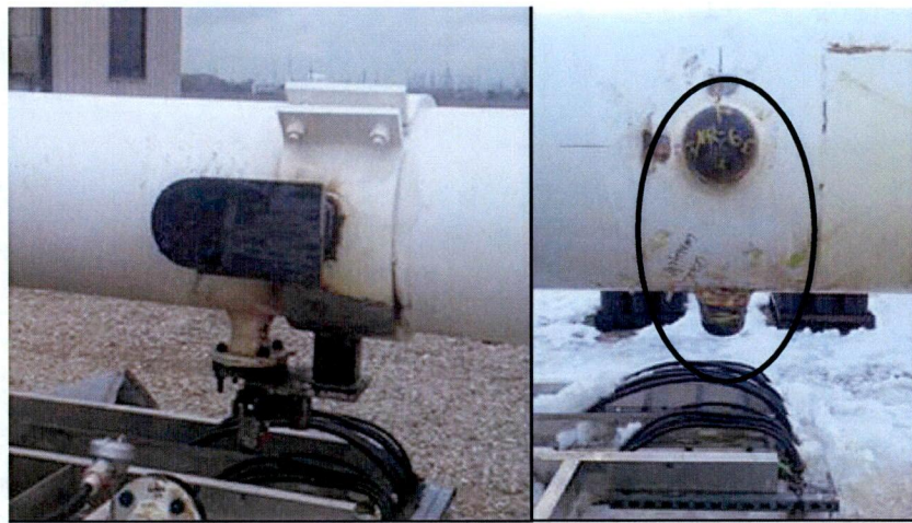
Figure 6: Drain and water injection nozzles downstream from the PCV: original configuration (left) and removed and capped nozzles (right).
