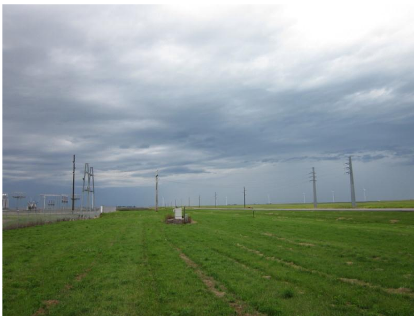
Photo 24. Direction: West. Transmission line connection at substation.
