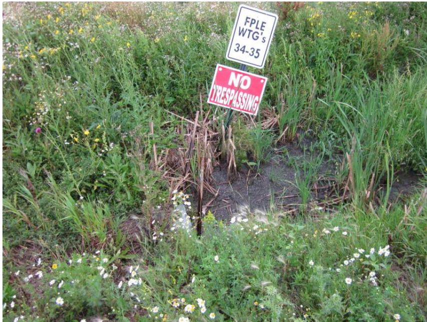
Photo 32. Sign at entrance to access road for towers LD-34 and LD-35 was being washed out by nearby culvert.
