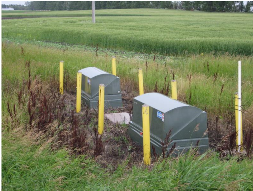
Photo 16. Direction: Northwest. Two junction boxes (F3-JB36 and F2-JB24) at intersection straight east of tower OT-18. The site was in good condition with no signs of settlement or erosion around the boxes or bollards.
