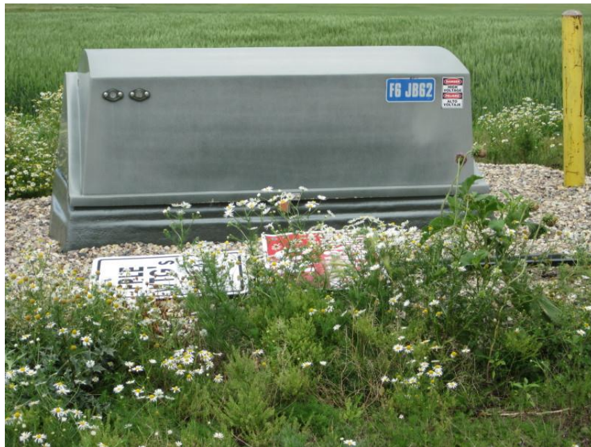
Photo 46. Direction: North. A signpost had been broken off and was placed beside junction box F6-JB62.
