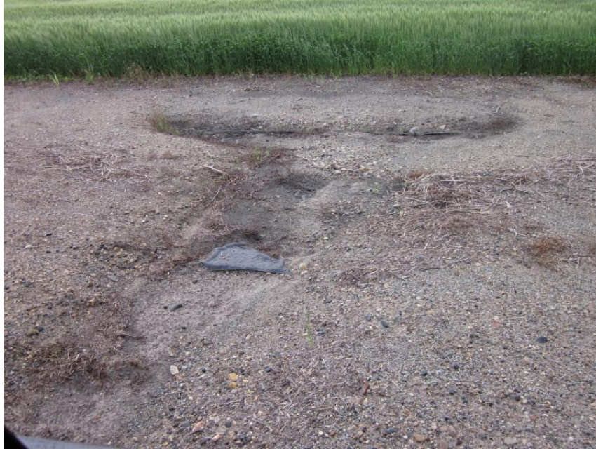
Photo 15. Direction: East. Erosion between towers OT-5 and OT-6 to the south of a Texas crossing, immediately to the east of tower OT-6. Geotech fabric was showing through gravel surface.
