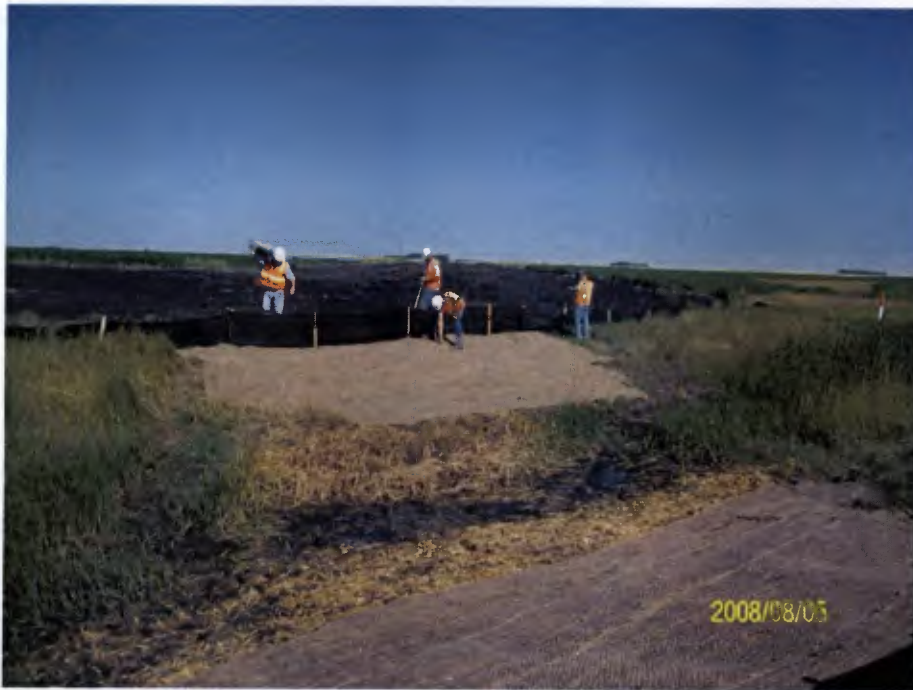
Environmental crew installing erosion controls following completion of waterbody crossing at MP 790.
