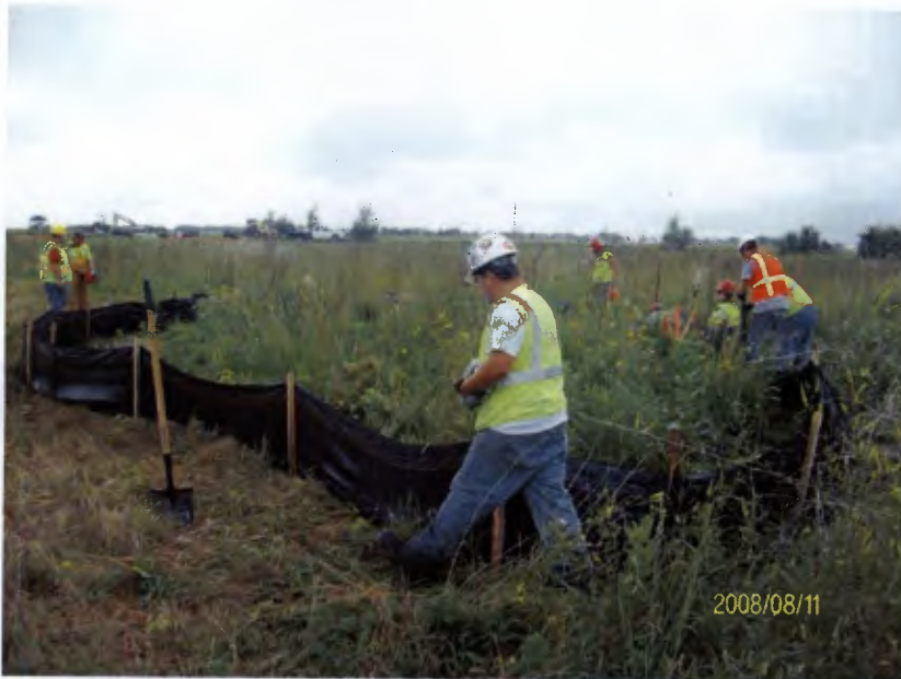
Containment of initial inadvertent return at the Pembina River
