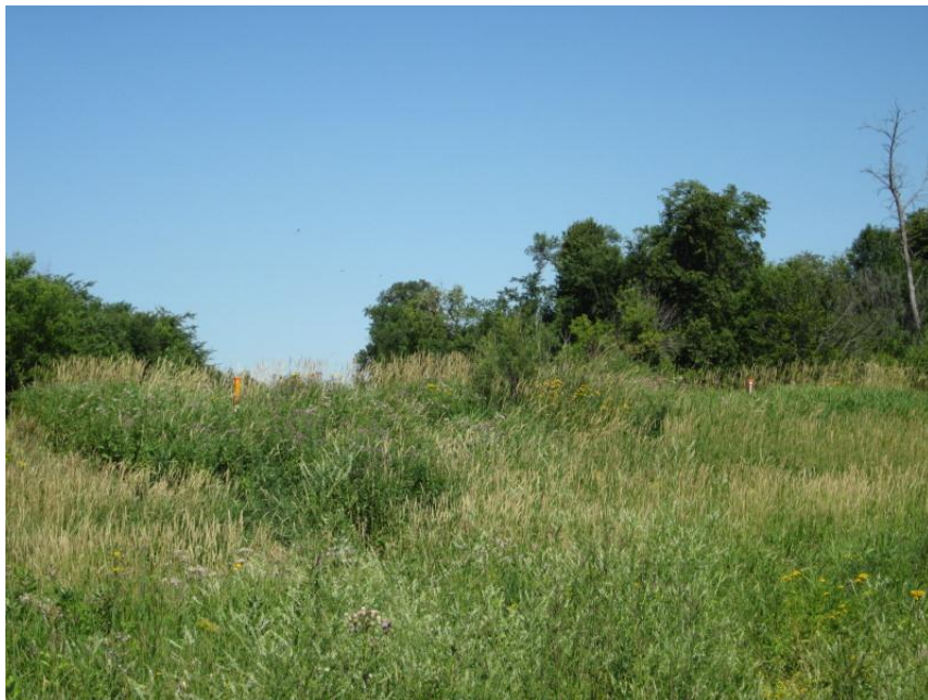
Photo 20. Direction: Northwest. Pembina River crossing. View of south bank, showing orange pipeline markers amidst the tall grasses, at approximately Mile 775.6. The river had been avoided by horizontally drilling underneath.
