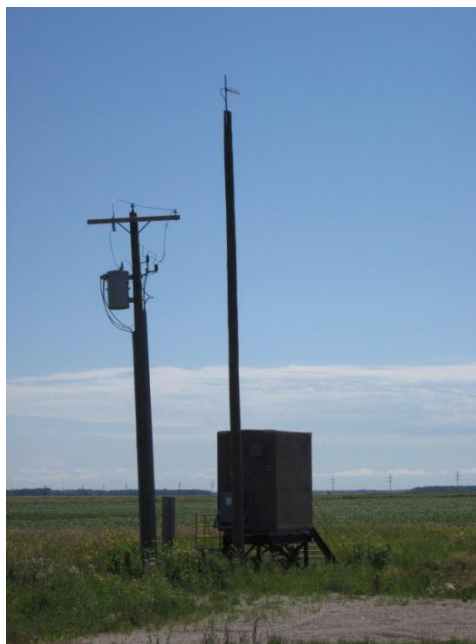
Photo 24. Direction: Southeast. Densitometer next to the valve system, which measures the density of the oil flowing through the pipeline. Information on the line served was not available at the time of the survey.
