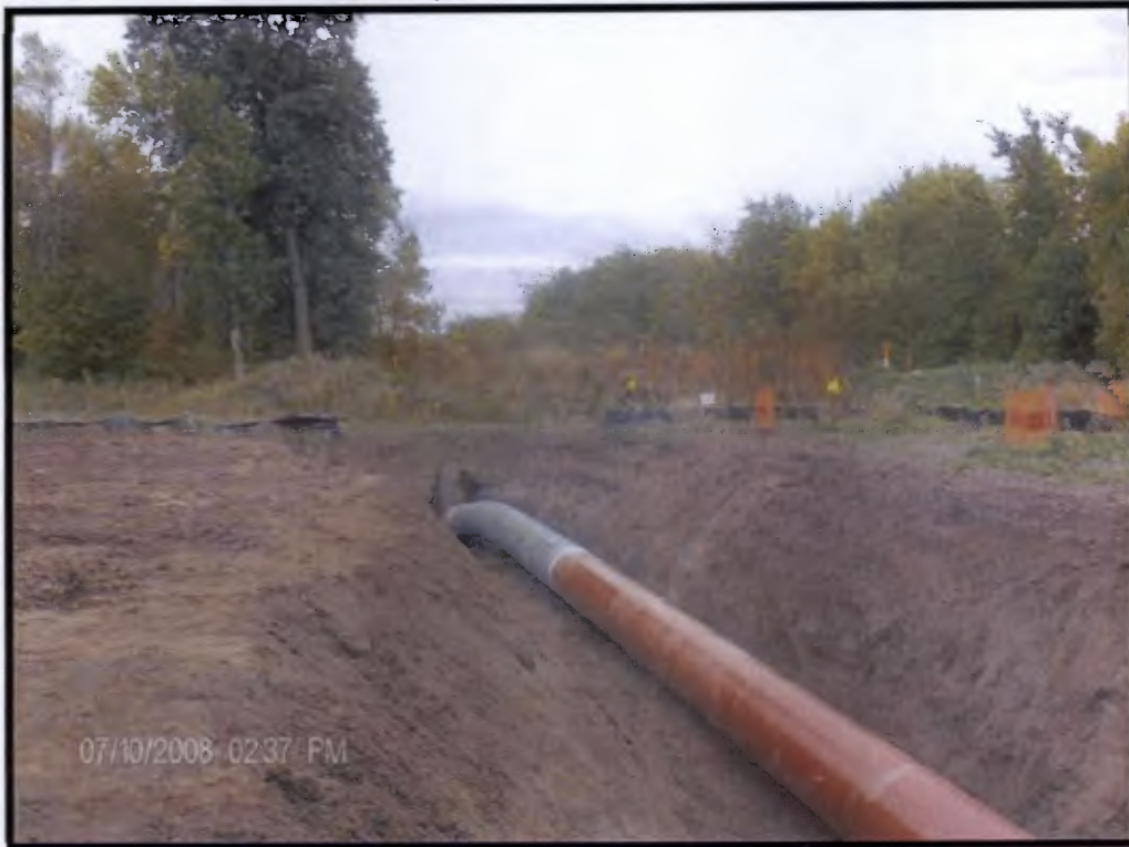
Connection of mainline pipe segment to HDD pipe segment under Tongue River
