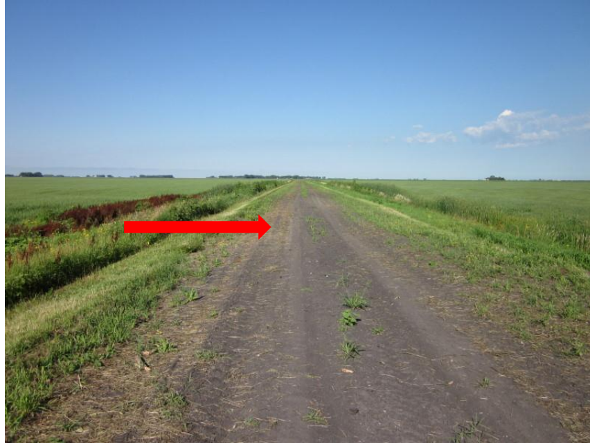
Photo 11. Direction: West. Southeast of Mile 799 at crossing of 91 st St NE. There was a slight depression in the road where the pipeline crossed (red arrow). The dip was not problematic and there was no erosion, but the location should be monitored. The vegetation in the ditch and the crops adjacent to this area appeared to have no impacts.
