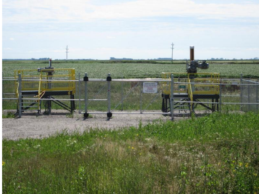
Photo 23. Direction: Southeast. Pipeline valve system to the northeast of the intersection of 147 th Ave NE and 107 th St NE (County Hwy 55), near Mile 777. The LSr valve is on the left and the Alberta Clipper valve is on the right.
