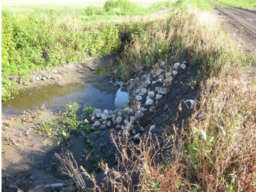
Photo 7. Direction: Northeast. Culvert installed at crossing of 161 st Ave NE, to the southeast of Mile 797. There were no signs of settling or erosion around the culvert. It appeared to be in good condition.
