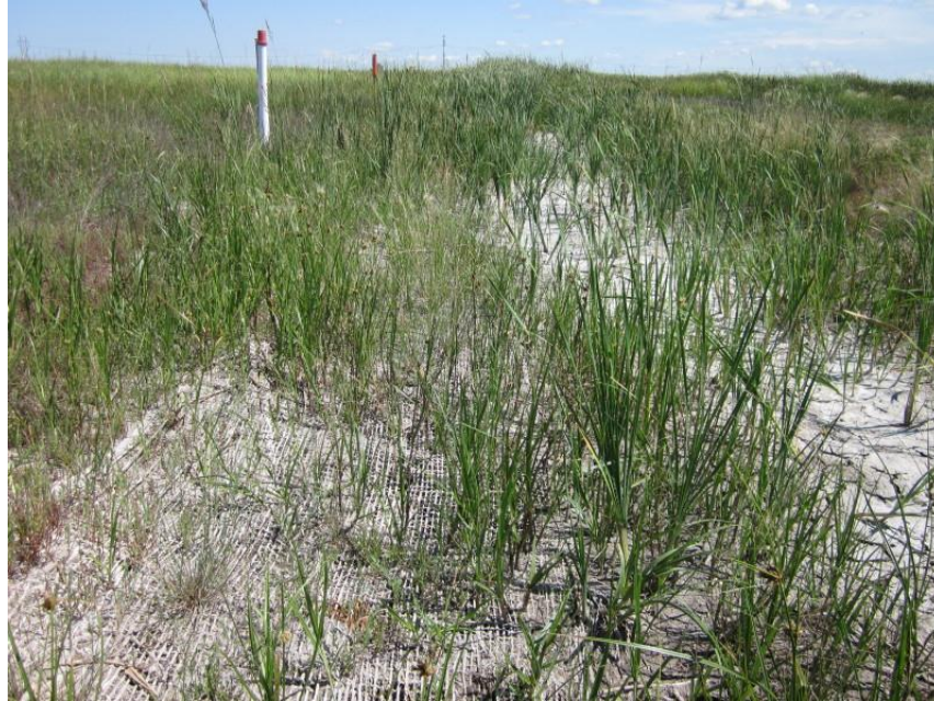
Photo 37. Direction: East. Ditch along minimum maintenance portion of 97 th St NE between Miles 790 and 791, within the wetlands surrounding Juhl National WMA. Pipeline route is marked by the posts on the left. Jute netting was in place in the ditch to stabilize soils and was functioning well. New vegetation was growing through the netting, including many native species such as prairie cordgrass ( Spartina pectinata ) and cattails ( Typha sp.) and the non-native but common grass quackgrass ( Agropyron repens ).
