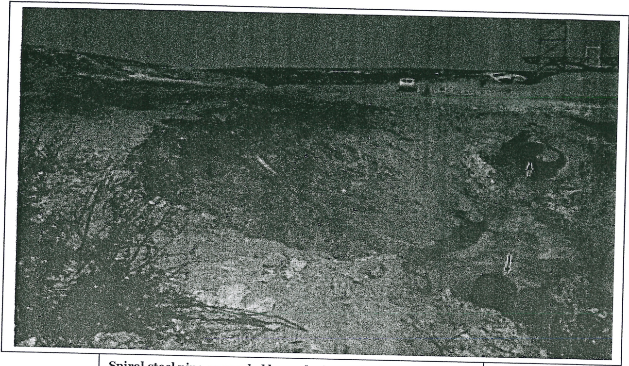
Spiral steel pipe unraveled by explosion at Carlsbad, NM
