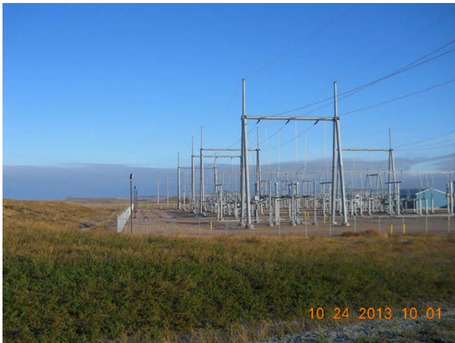
Photo 8 – Direction: North – Rhame Substation
