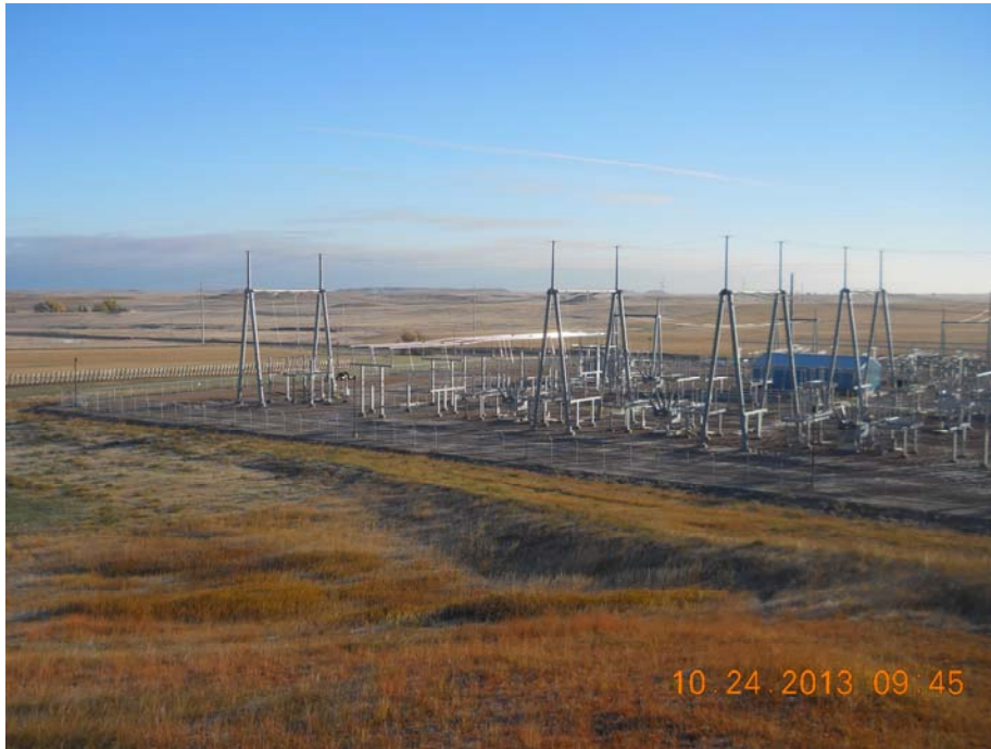
Photo 1 – Direction: Northeast – Rhame Substation
