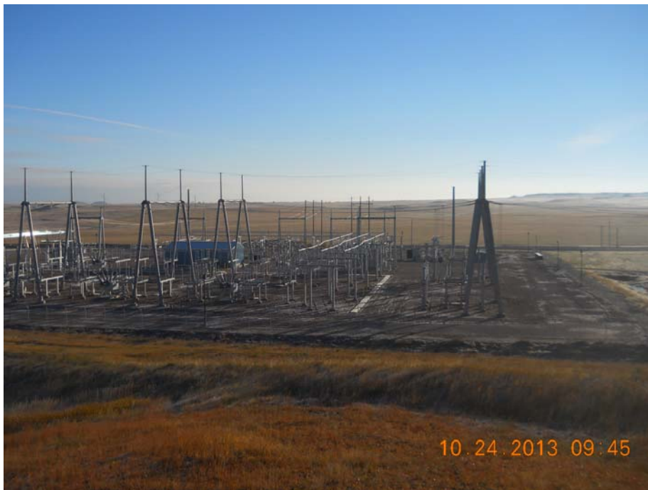
Photo 2 – Direction: East – Rhame Substation.
