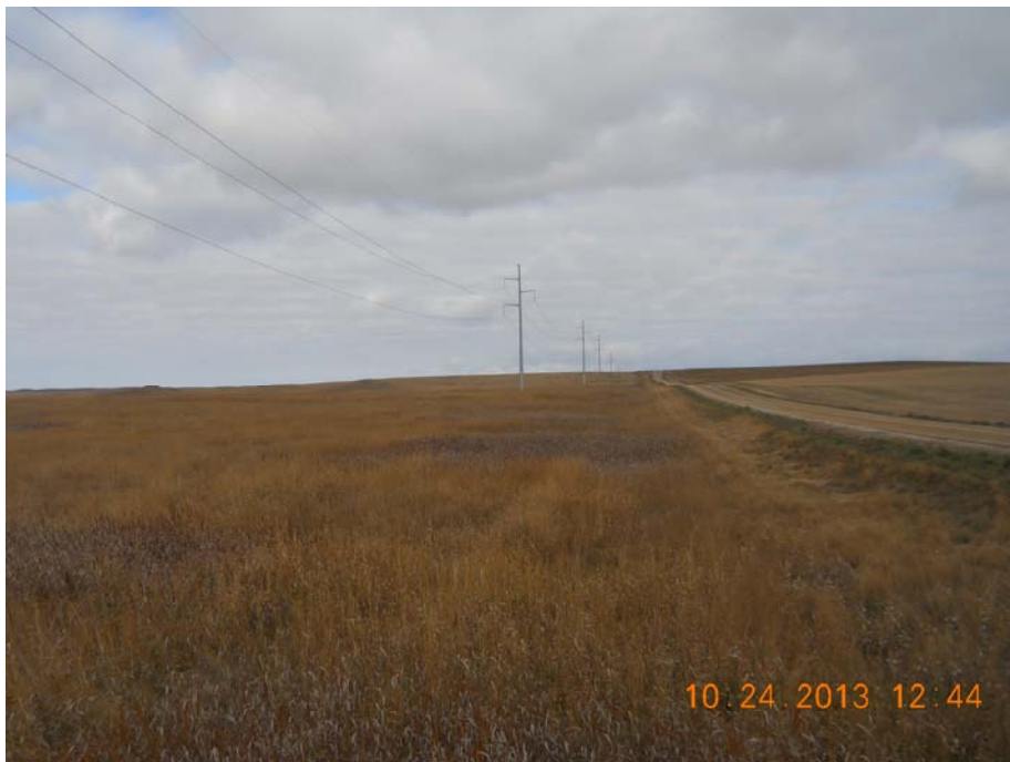
Photo 25 – Direction: North – Showing transmission line moving north along a county road.
