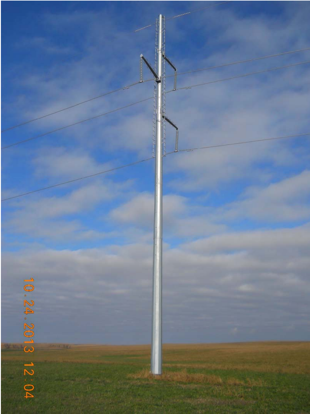
Photo 20 – Standard transmission line structure used for the Project.
