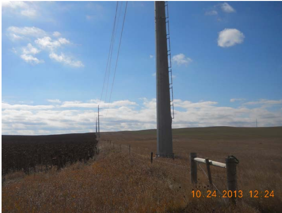
Photo 23 – Direction: South – Looking back on transmission line towards Rhame Substation. Notice integrity of fence and gate and the completed reclamation.
