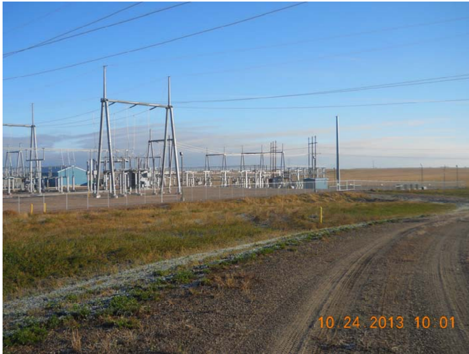
Photo 9 – Direction: Northeast – Rhame Substation and access road to the south.
