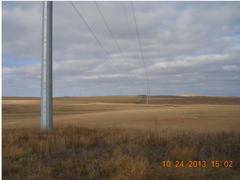
Photo 33 – Direction: North – Looking at span of transmission line across a drainage pathway. No adverse impacts to drainage pathway observed.
