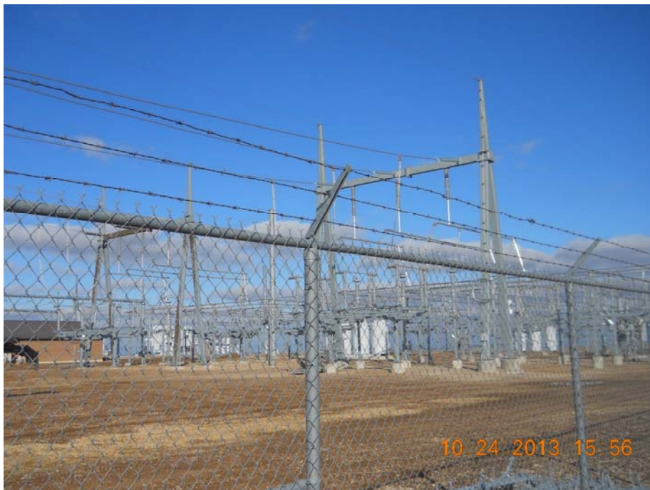
Photo 38 – Direction: Northeast – Takeoff structure inside the Belfield Substation.
