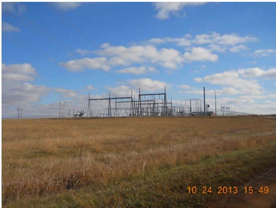
Photo 34 – Direction: South – Belfield Substation.
