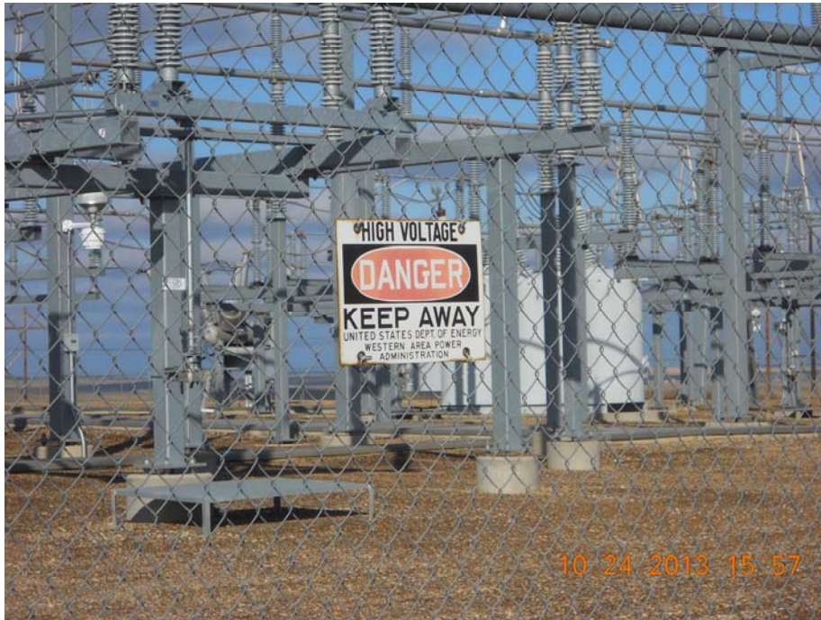
Photo 39 – Warning signs posted on Belfield Substation perimeter fence.
