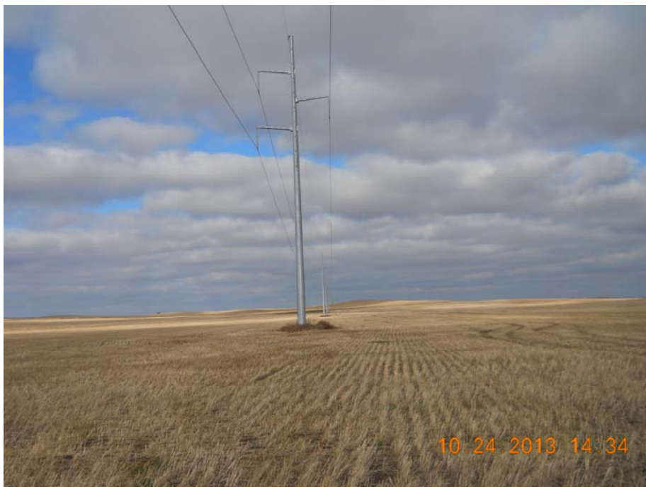
Photo 29 – Direction: North – Transmission line moving north. Notice minimal loss of cropland at the base of structures.
