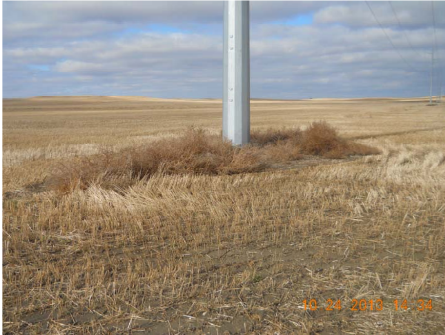
Photo 31 – Direction: West – Showing base of structure from Photo 30. Notice presence of weeds, controlled by continued farming around base of structure.
