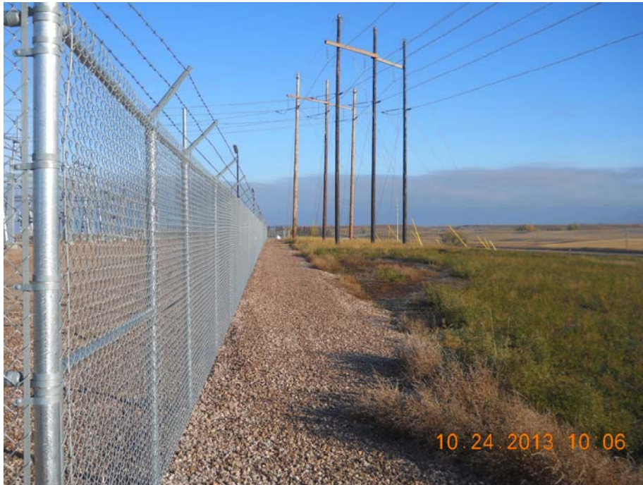
Photo 12 – Direction: North – Taken at southeast corner of Rhame substation. Showing well maintained gravel perimeter around fence. Also notice problem with vegetative cover on the right side of the photo, directly east of the Rhame Substation.
