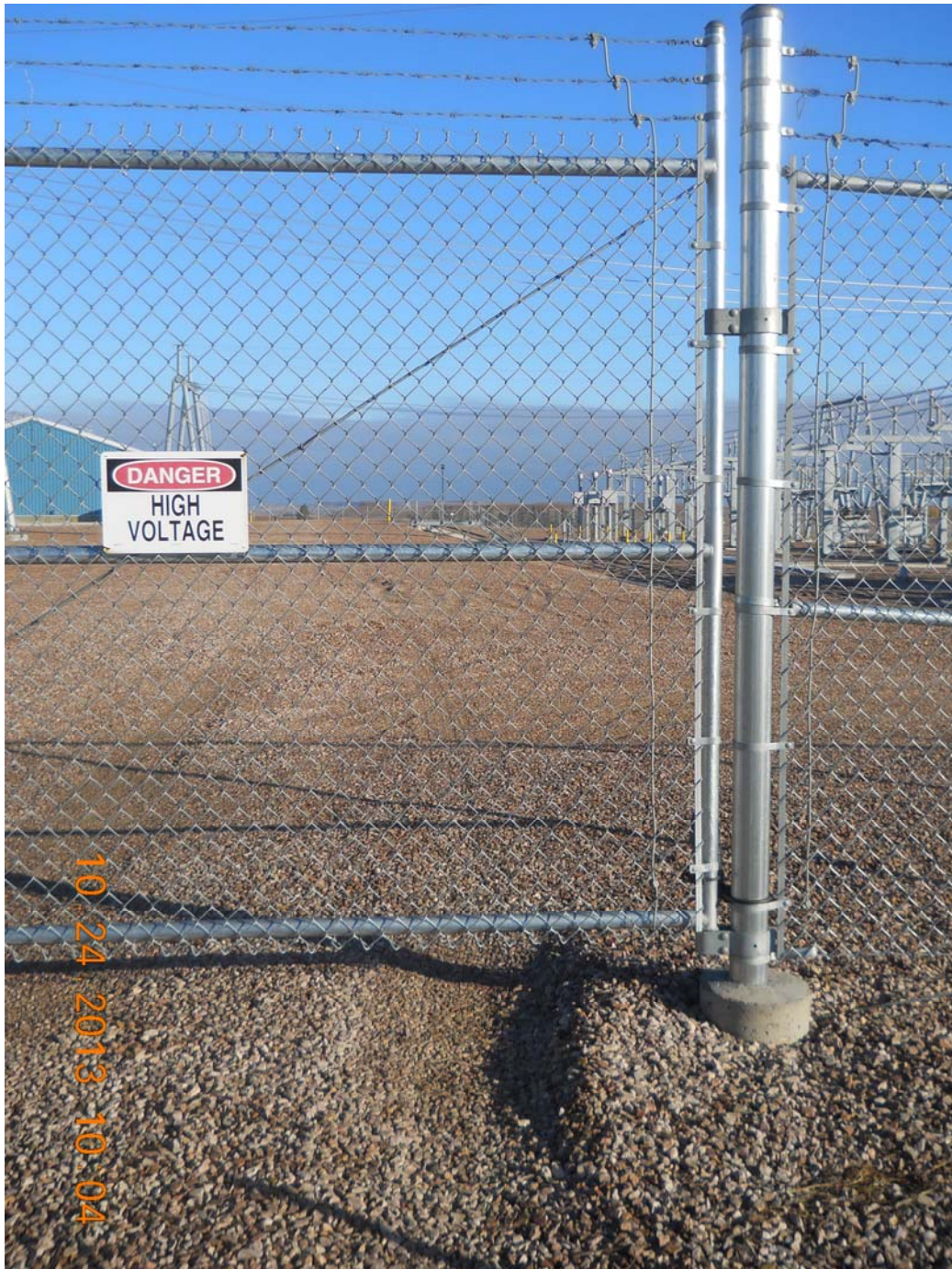
Photo 11 – Direction: North – Taken at Rhame Substation south access gate. Showing gap of approximately 12-14 inches at the bottom of the fence. Large enough for small wildlife to enter substation.
