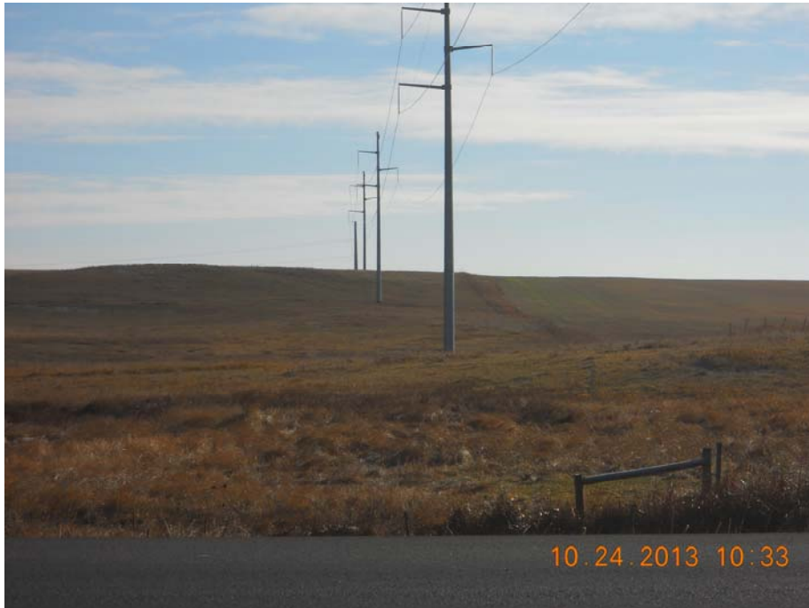
Photo 16 – Direction: East – Showing standard structures directly east of Rhame Road crossing north of Rhame Substation. Notice line turns north after hill in the distance.
