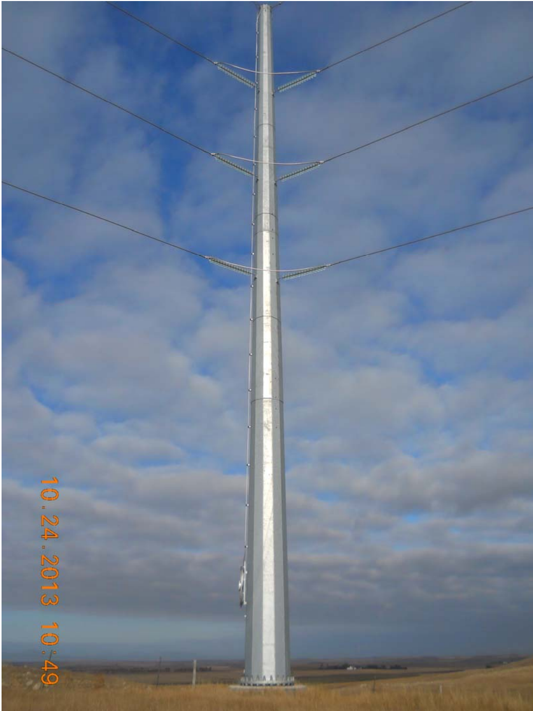
Photo 19 – Typical angle structure.
