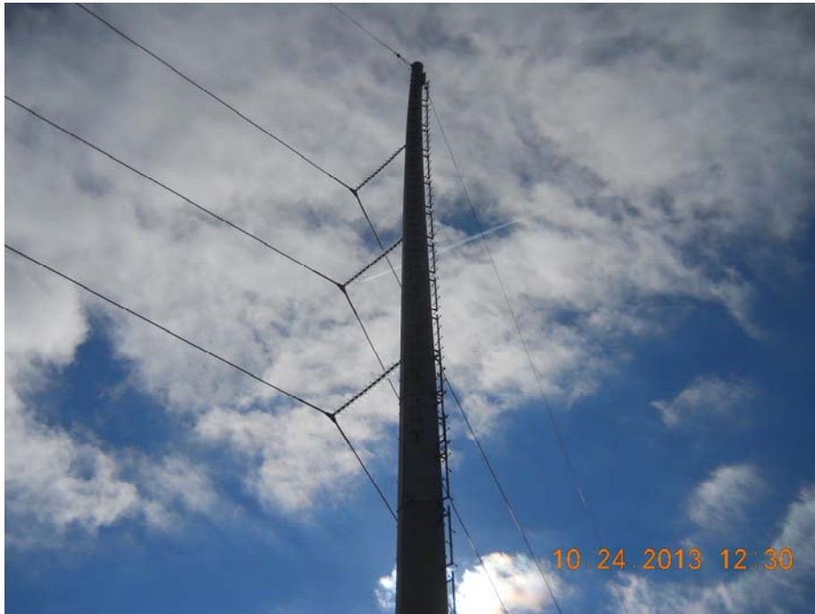
Photo 24 – Notice angle structure appears leaning at the top of the structure.
