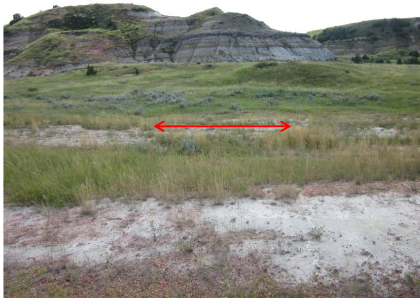
Photo 31. Direction: South/Southwest. Looking perpendicular to pipeline route as it paralleled an unnamed Forest Service Road diagonally through the center of Section 35, T148N, R102W. Re-vegetation of the right-of-way in this area was sparse and inadequate, with a significant amount of bare clay soils.
