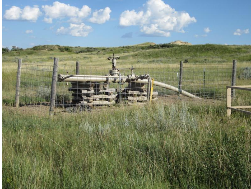
Photo 33. Direction: Southeast. Above-ground valve setting along pipeline route in the N ½ of the NW ¼ of Section 1, T147N, R102W.
