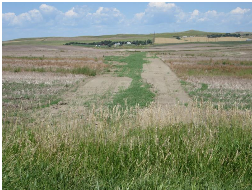
Photo 14. Direction: North. Pipeline right-of-way recently bladed to repair low areas upon landowner request. Photo taken from private east-west gravel road between Sections 7 and 18, T150N, R101W, which had been bored underneath, according to the as-built drawings. The stubble field was in the SE ¼ of Section 7.
