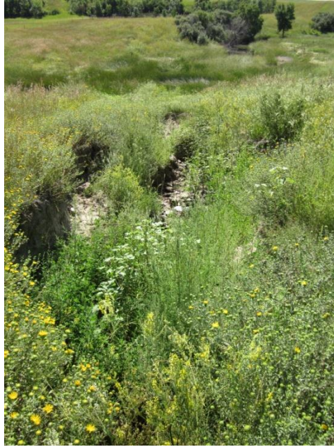
Photo 9. Direction: South. View of eroded trench from north to south looking towards Camp Creek (dark green vegetation visible in distance). As-built drawings indicated it had been open cut. The channel of Camp Creek itself appeared to be in good condition with no erosion problems and complete revegetation. Tree and shrub patches were avoided.
