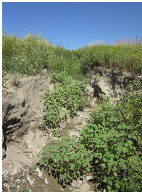
Photo 8. Direction: North. Eroded trench on north Bank of Camp Creek (NE ¼ of the SW ¼ of Section 6, T151N, R101W, at approximately pipeline distance 1463ft). The erosion was within the pipeline right-of-way and appeared to be due to settling and water erosion around the pipeline. At its deepest, the trench was four to five feet deep and had large rocks in the bottom.
