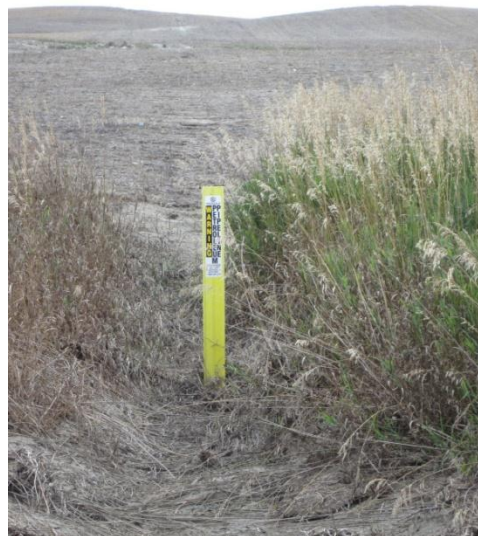
Photo 22. Direction: North. Another view of erosion in fields to north of 19 th St NW. There appeared to be a natural spring or a plugged culvert just to the east of the pipeline intersection along the road. There were very deep ruts in the road in that area. This was outside the pipeline right-of-way but the water accumulation was contributing to the erosion problems.
