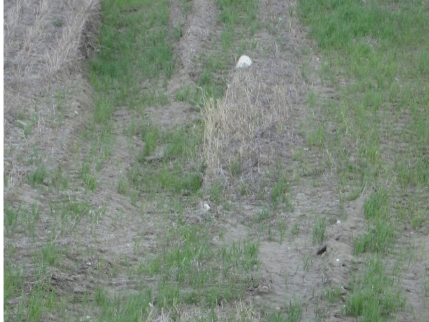
Photo 17. Direction: Northeast. Trenches/settling in pipeline right-of-way in stubble field to the north of County Route 15. There was a shallow coulee/drainageway in this portion of the field where water runs across the right-of-way during precipitation events and probably contributes to the settling in this location.
