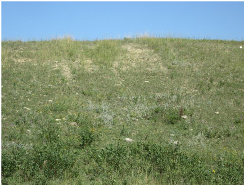
Photo 4. Direction: Northwest. Hill within pasture/rangeland on pipeline route in the NE ¼ of the NW ¼ of Section 30, T152N, R101W, leading into an unnamed drainage. There were minor areas of erosion and bare soils within the pipeline right-of-way on the upper slopes. The native vegetation of the surrounding pasture was spreading into the reclaimed route.
