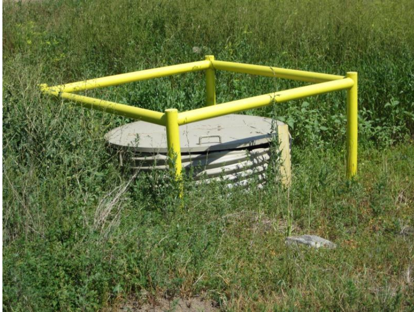
Photo 15. Direction: Northeast. Block valves for the pipeline along the gravel road between Sections 7 and 18. There was some settling around the valves and through the middle of the ditch, which was dense with yellow sweetclover ( Melilotus officinalis ).
