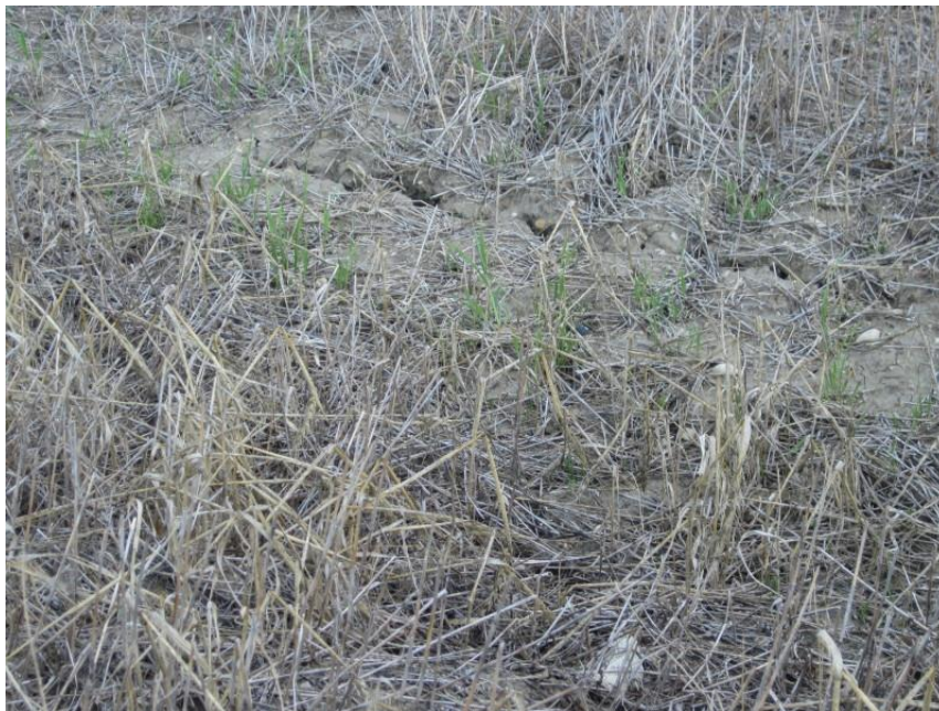
Photo 16. Direction: Northeast. Cracking in soil on pipeline right-of-way. This was on the edge of a stubble field to the north of County Route 15, which went east-west through the center of the SE ¼ of Section 18, T150N, R101W.
