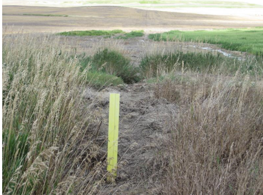
Photo 21. Direction: South. At intersection of pipeline with 19 th St NW, a sectionline trail which ran east-west between Sections 30 and 31, T149N, R101W. Markers were present which indicated the pipeline right-of-way. This road had been open cut, according to the as-built drawings. There was an extensive area of erosion about ¼ mile north and ½ mile south of this point in fallow fields. The road had deep ruts and erosion 12-18 inches deep and the fields had ruts 6-12 inches deep.
