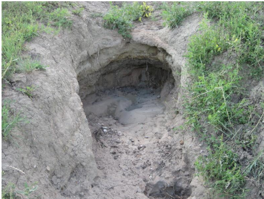
Photo 26. Direction: Northwest. Erosion from runoff in ditch of Forest Service Road 835 in the N ½ of Section 15, T148N, R102W, at the point where the pipeline crossed. Markers were in place on both sides of the road. The pipeline also intersected Spring Creek at this point. The as-built drawings were unclear and difficult to distinguish but appeared that Spring Creek and the road had been bored underneath.
