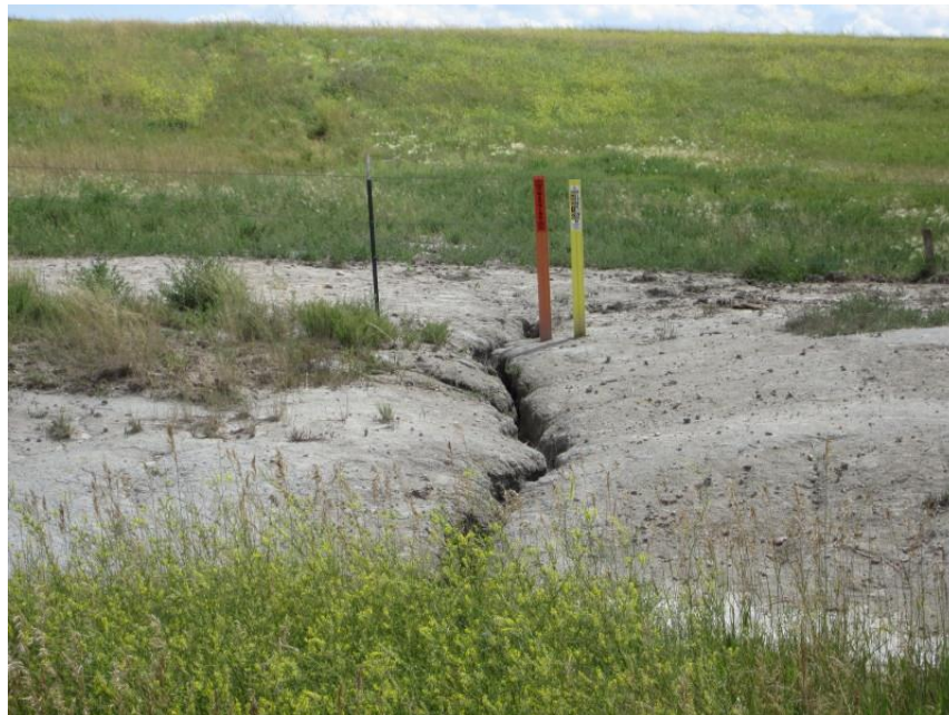
Photo 24. Direction: South. South ditch of State Highway 68 showing erosion of clay soils within pipeline right-of-way. The highway had apparently been bored underneath, so the erosion may not have been due to the pipeline. High amounts of spring runoff this year may have prompted the particularly deep erosion channels.
