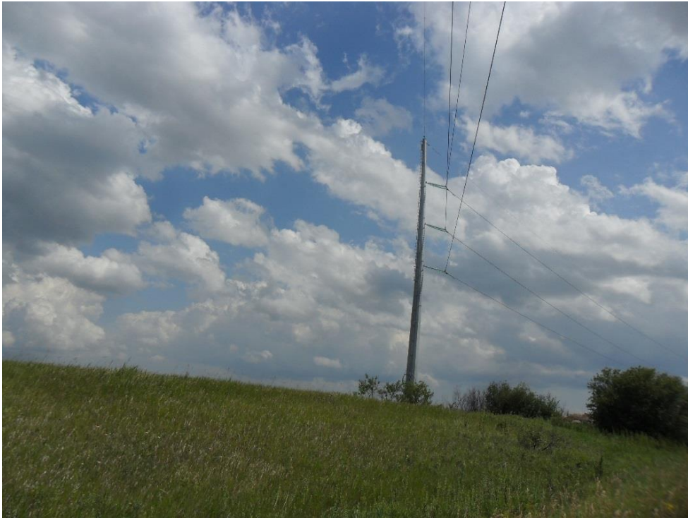
Photo 15 – Direction: Southeast - Angle structure near Tioga. Notice apparent lean.
