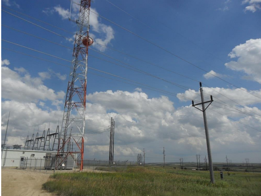
Photo 17 - Direction: Southeast – Tioga Substation
