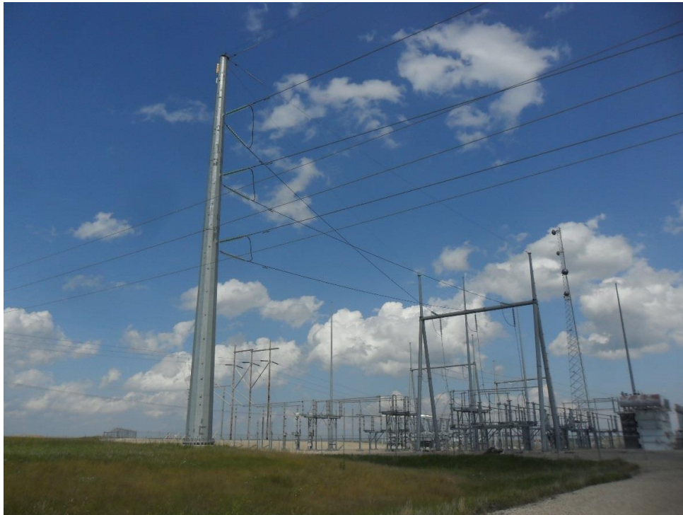
Photo 16 - Direction: Northeast – Entering Tioga substation
