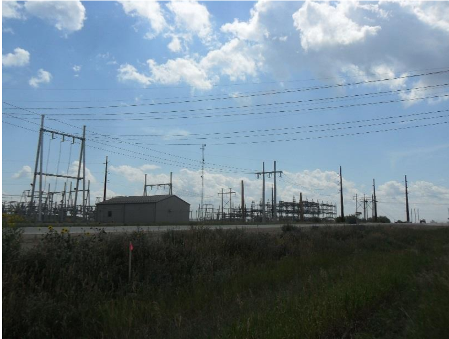
Photo 1 - Direction: Southeast – Williston Substation
