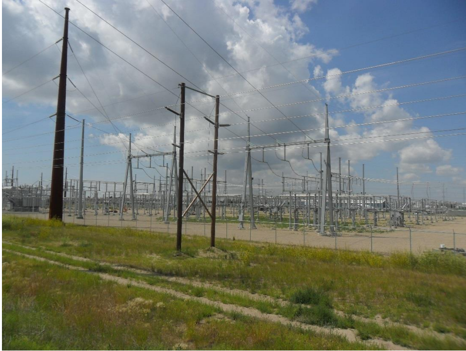
Photo 5 - Direction: Southwest – Williston Substation where transmission line enters
