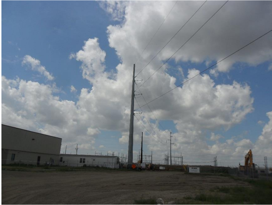
Photo 7 – Direction: West - Transmission line exiting Williston Substation
