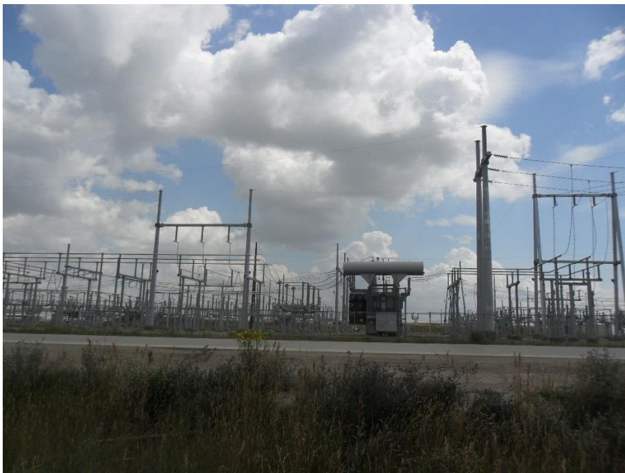
Photo 2 - Direction: East – Williston Substation
