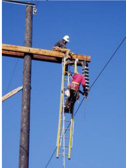
Figure 3-4. Clipping of Conductor to the Insulator
