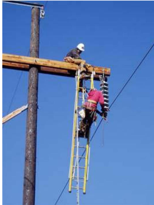
Figure 3-4. Clipping of Conductor to the Insulator
