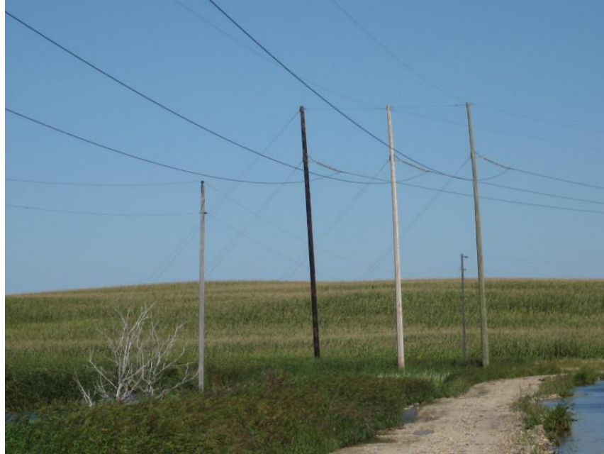
Photo 5. Direction: Northeast. Set of three monopoles at the east end of the reroute. The monopoles had guy wires attached and were also outside the flooded area.
