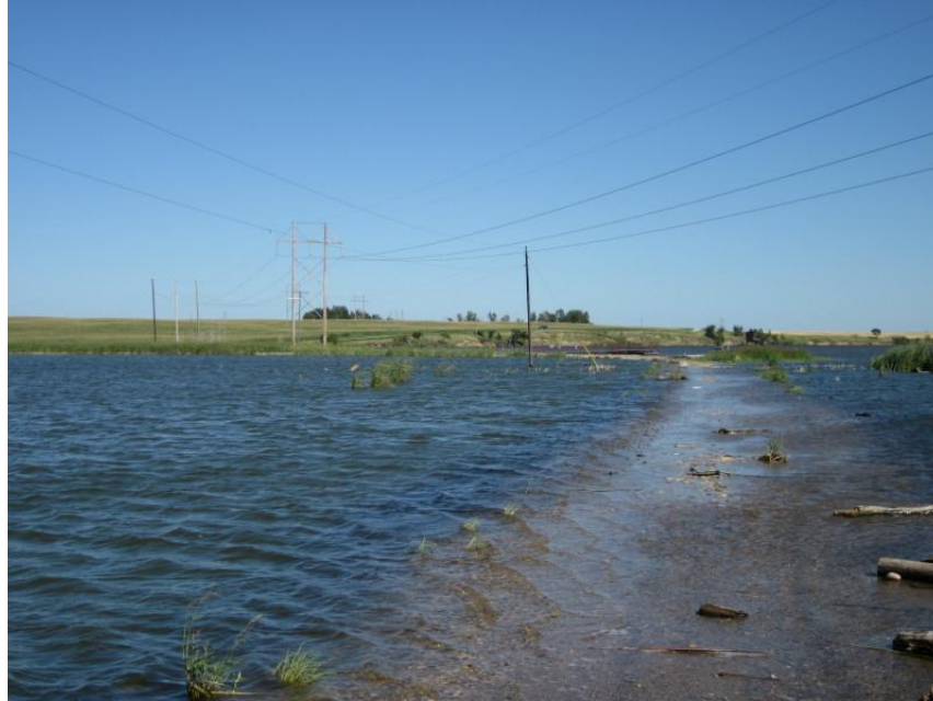
Photo 3. Direction: East/Northeast. Overview of east end of transmission line reroute. From the monopole structures in Photo 1, the reroute line crossed a gravel road (90 th St SE), attached to a wooden H-frame structure (distant left of photo), then attached to another set of three monopoles (distant far left), then connected back to the original route. Grass (Sand) Lake flooded the road at the time of the survey. The east end of the reroute was accessed by walking across the shallow water on the road.
