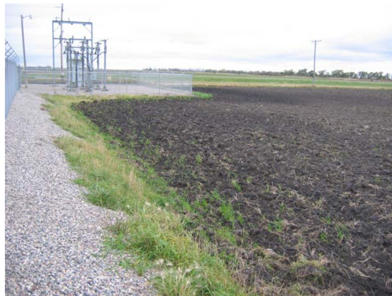
Crookston Station. View of northern edge of facility and location of the proposed control building.
