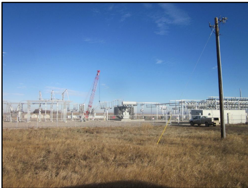
Photo 4. Direction: Northeast. Barnes Substation serving the Ashtabula I turbines, to the west of the O&M building and grounds. Note the crane in the distance to the north of the substation which was still being actively used for construction staging, storage, and maintenance purposes. The area around the substation had been reclaimed and the vegetation was established and in good condition.
