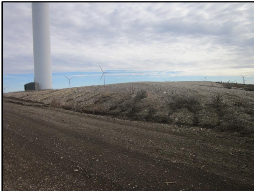
Photo 18. Direction: Southeast. The edges of the gravel pad of Turbine OT48 had eroded channels, which drained toward the edge of the access road, where a deep eroded channel had formed.
