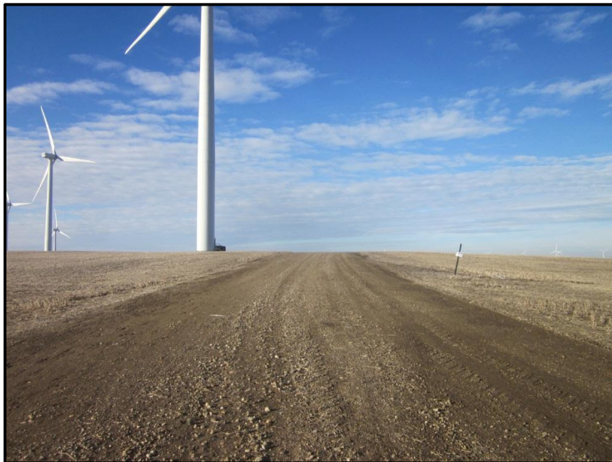
Photo 6. Direction: West. Access road entrance to Turbines 131-125 from its intersection with 125 th Ave SE. Proper safety and public access signage was in place, though the sign with the turbine names was missing. Cropland adjacent to road and turbines were in good condition and had been satisfactorily reclaimed. An archeological site on this hill had been destroyed by plowing and was deemed not necessary to avoid during Project construction.
