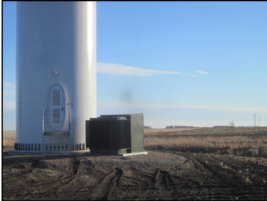
Photo 29. Direction: Southeast. Close-up of base of Turbine 23, showing example of a transformer with extra containment for oils in the pad mount. This is for extra protection in the case of a spill, since this turbine is near a wetland area (visible in the right background) which was under USFWS wetland easement.
