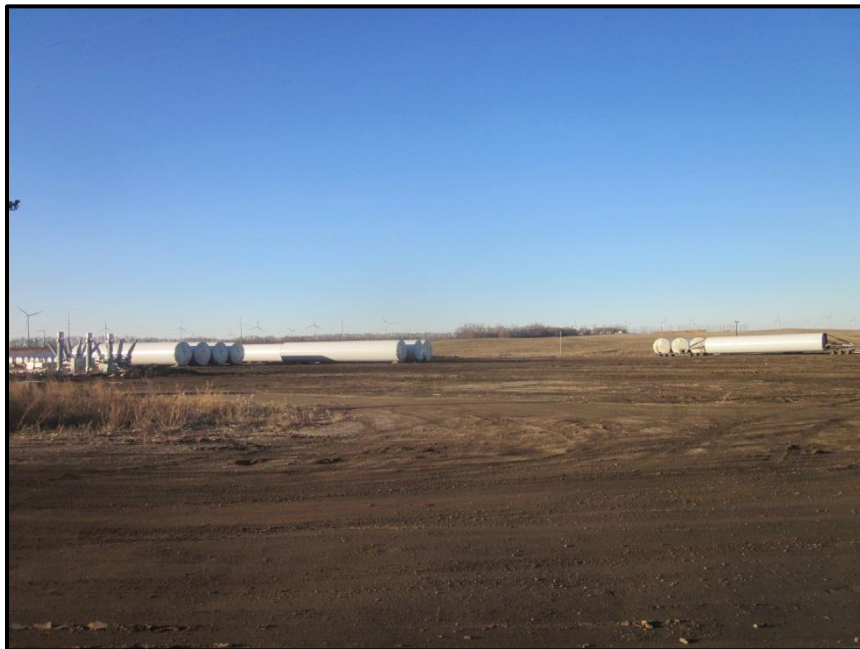
Photo 2. Direction: North. Central portion of O&M grounds used for construction staging where tower sections were being stored.
