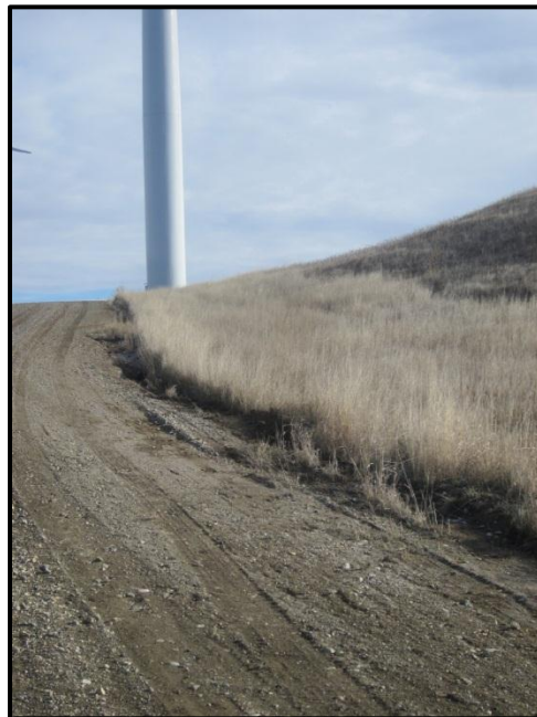
Photo 22. Direction: East. Looking back toward Turbine OT43. There were several spots on hills along this access road where erosion channels had formed on the edges; however as shown in this photo this problem was being addressed through routine maintenance by grading the road and filling in the channels. Also note the different coloration of the grasses seeded for reclamation along this portion of the road.
