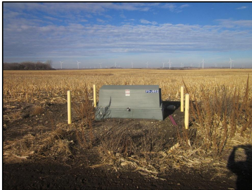
Photo 10. Direction: Northwest. Example of junction box conditions showing close-up of JB52 adjacent to access road. Cement bollards and gravel were in place around the box with no indication of erosion. Weeds appeared to have been sprayed on the gravel area, though there were a few annual weeds (tall brown vegetation) that had grown this past season. Safety warning signs were in place.
