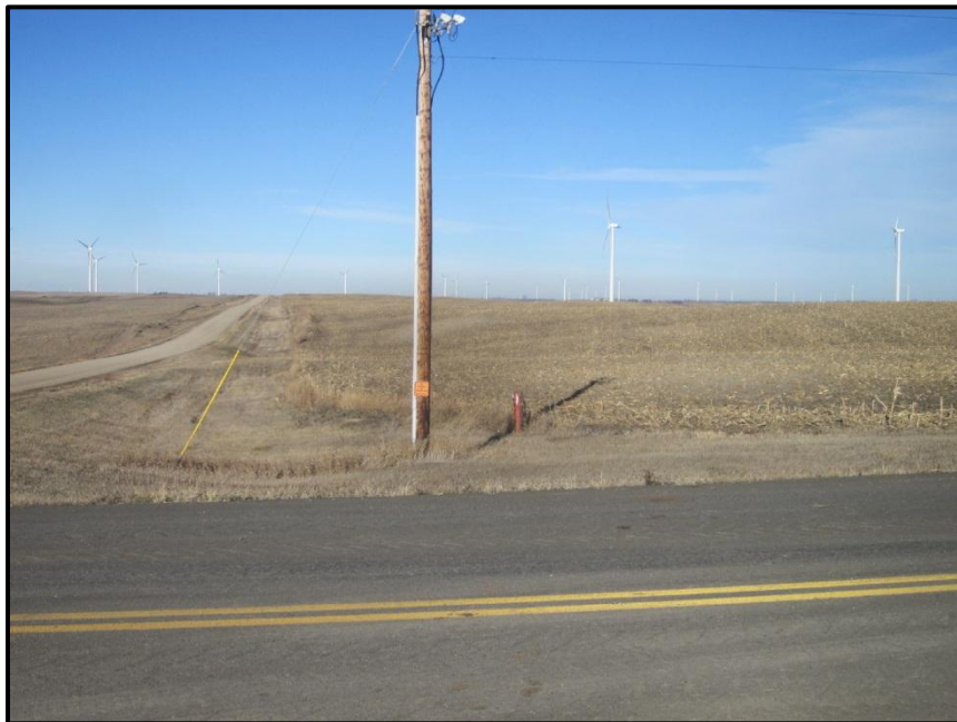
Photo 26. Direction: North. Collection line crossing of 18 th St SE/County Road 6, which had been bored. Note the red marker in the north ditch.
