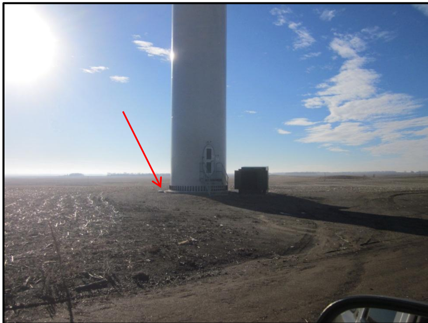
Photo 8. Direction: Southeast. Base of Turbine 129 showing example of typical conditions on the site. Cropland and gravel pad were in good condition. Safety signs were in place. Pad-mounted transformer is on right of tower base. This tower was one of several being controlled for mice infestations; note the small white trap to the left of the tower base (marked with red arrow).
