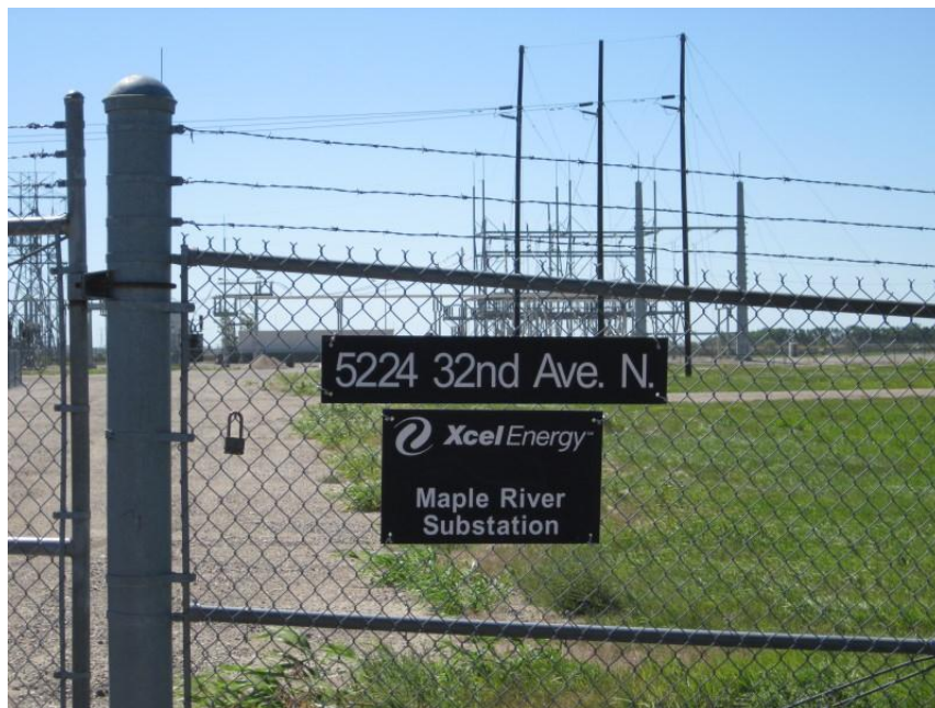
Photo 30. Direction: South. Entrance to Maple River Substation north of West Fargo. This was the east end of the 230 kV transmission line.
