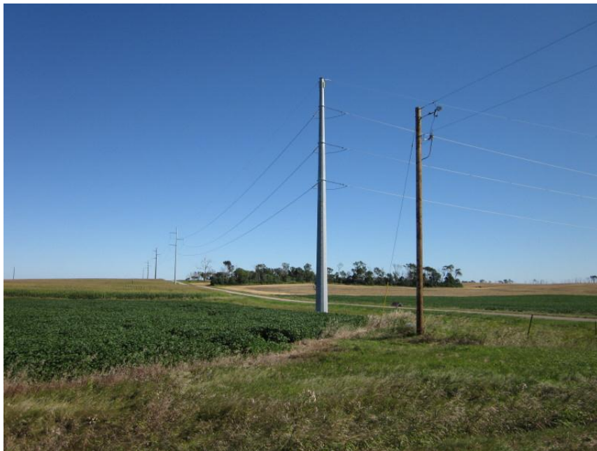
Photo 12. Direction: Northeast. Corner post at intersection of 143 rd Ave and 23 rd St. The line paralleled the west side of 143 rd Ave to the north of this point (left-center of photo), then crossed 143 rd Ave going east to parallel the north side of 23 rd St.
