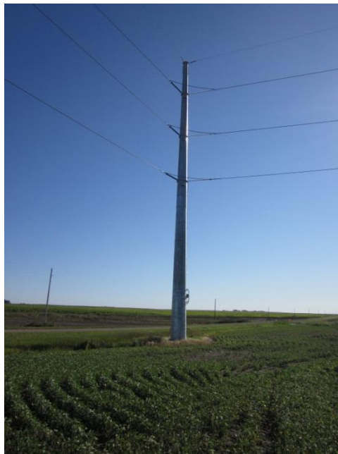
Photo 6. Direction: Northeast. Corner pole where transmission line turned from east to south at the intersection of 14 th St and 129 th Ave east of Pillsbury.
