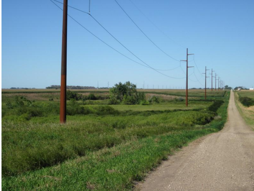
Photo 15. Direction: West. Example of wider spacing between poles to span the large wetland on the south side of the road (23 rd St between 147 th Ave and 148 th Ave).
