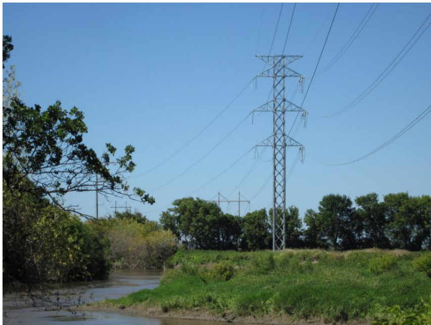
Photo 26. Direction: West. Crossing of the Sheyenne River northwest of West Fargo. At this point both the 230 kV line and the 345 kV line run together on the same structure (pole in foreground). Note there has been bank erosion on the Sheyenne due to spring flooding.
