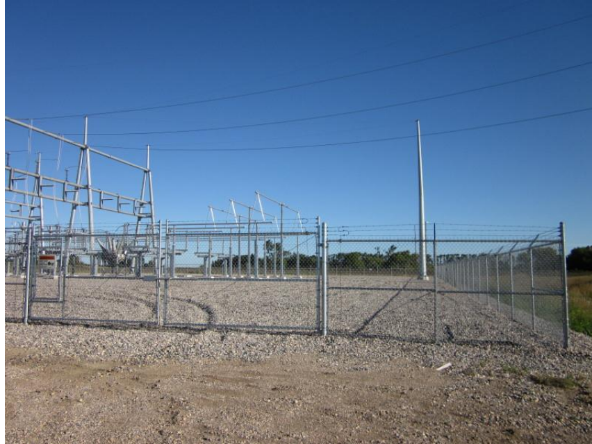
Photo 1. Direction: North. Entrance to the new Pillsbury Substation at the west end of the transmission line, about two miles west of the town of Pillsbury in the SW ¼ of Section 7, Township 143N, Range 56W, Barnes County, North Dakota.
