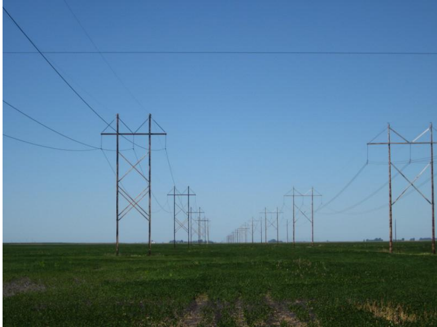
Photo 21. Direction: West. One mile in distance is where the line turned from north-south along 162 nd Ave to east-west, about one-fourth of a mile north of, but parallel to, 32 nd St. At the corner described, the use of monopoles shifted to the use of H-frame structures. Note the 345 kV line parallel to the 230 kV line to the north (on right in photo).
