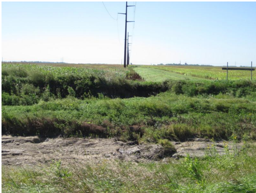
Photo 20. Direction: South. Transmission line crossing of the channelized Rush River along 162 nd Ave to the south of its intersection with 30 th St. The line spanned the channel and avoided disturbance of the waterway.
