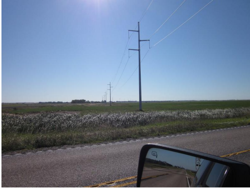
Photo 11. Direction: Southeast. Intersection of Highway 38 and route of transmission line, to the south of the town of Page. The line continued to parallel a railroad. There were bird deterrents in both directions on this portion of the line.
