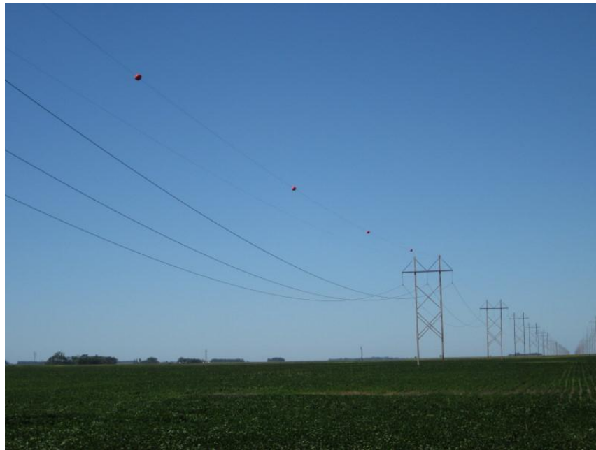
Photo 24. Direction: West. Intersection of transmission line with 81 st St, just to the north of 52 nd Ave, northwest of the city of West Fargo. The large orange balls on the line were presumably there for aircraft safety purposes.
