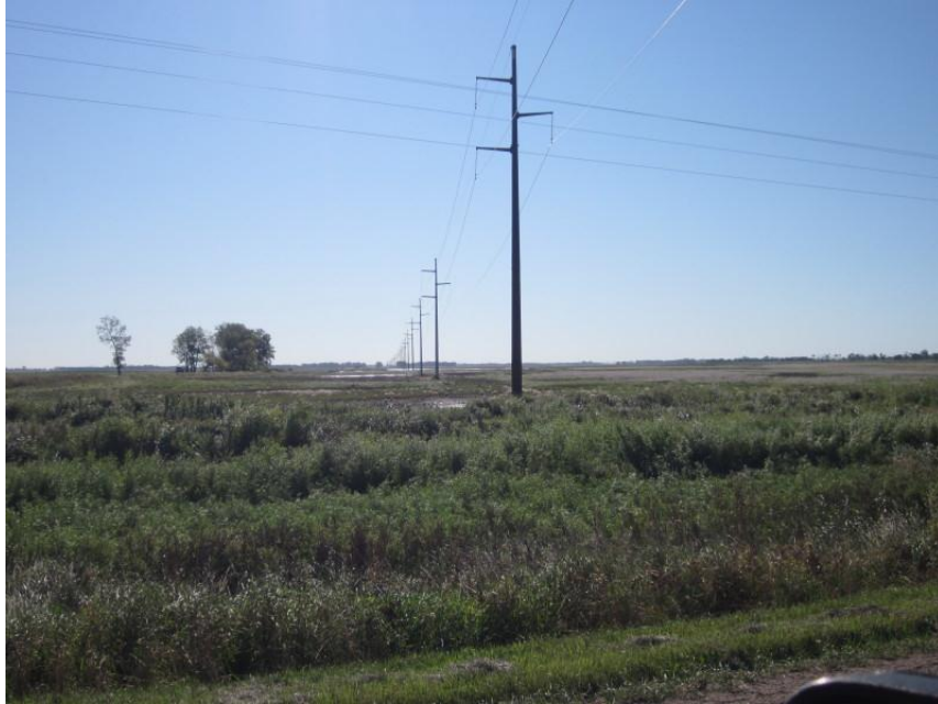
Photo 9. Direction: Southeast. Intersection of 133 rd Ave and route of transmission line, looking to the southeast, where the line paralleled a railroad to the southeast of Pillsbury.
