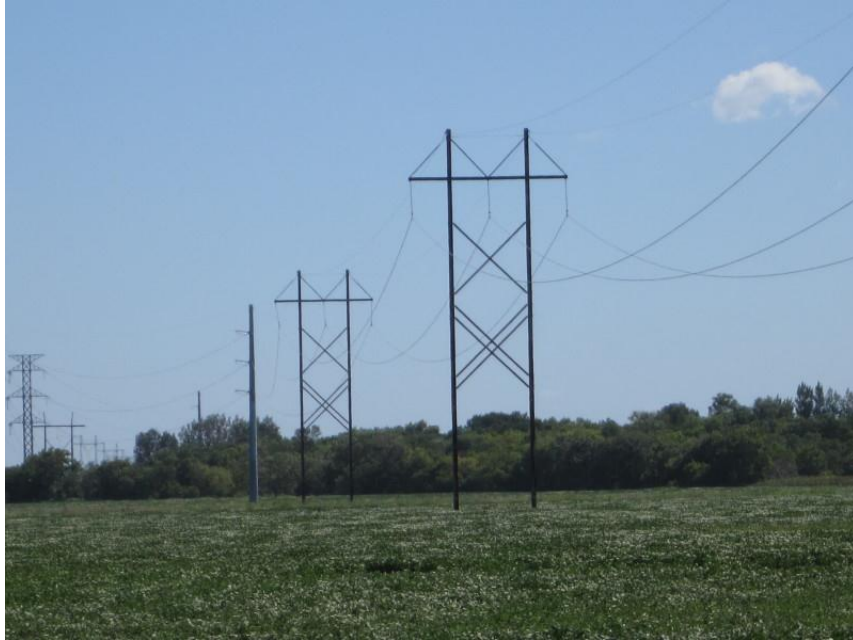
Photo 25. Direction: East. Intersection of transmission line with 81 st St, just to the north of 52 nd Ave, northwest of the city of West Fargo. Note the switch from H-frame structures to monopoles about ½ mile before the crossing of the Sheyenne River, which is indicated by the dense trees in the distance.
