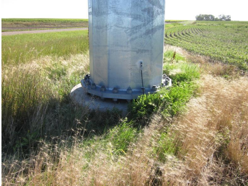
Photo 7. Close-up of pole in Photo 6 showing concrete footing of base, which is how all corner poles were constructed.
