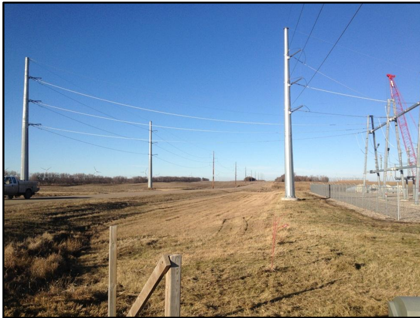
Photo 12. Direction: North. South end of the transmission line at the Ashtabula Wind Energy Center substation.
