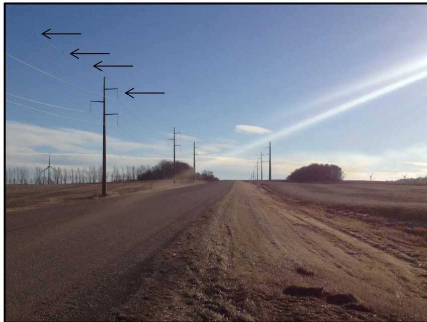
Photo 10. Direction: South. View of the transmission line crossing 123 rd Ave. SE along 19 th St. SE. There were flight diverters along this portion of the route (indicated by black arrows).
