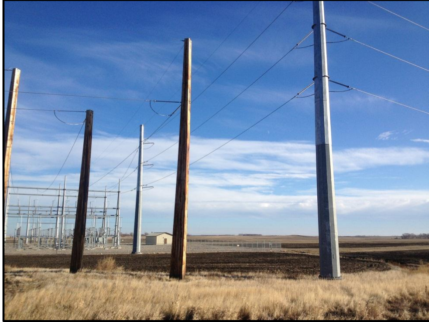
Photo 1. Direction: Southeast/East. North end of the transmission line (steel poles) at the Pillsbury substation.
