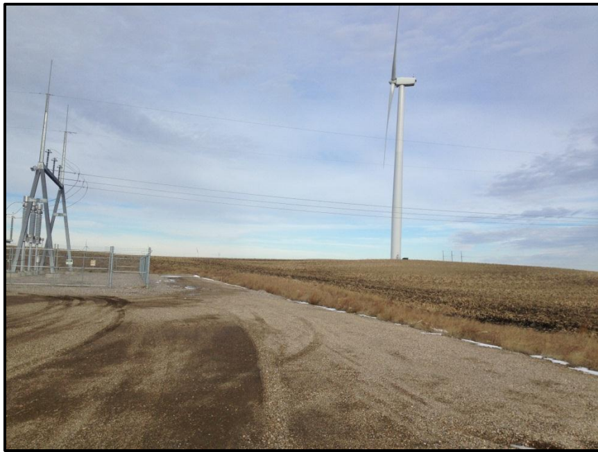
Photo 10. Direction: North. View of the transmission line as it interconnects with the Luverne substation.
