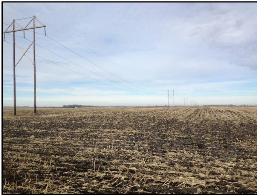
Photo 6. Direction: Northwest. View shows typical span and structure design of the transmission line. No impacts to agricultural land or crop production were noted.
