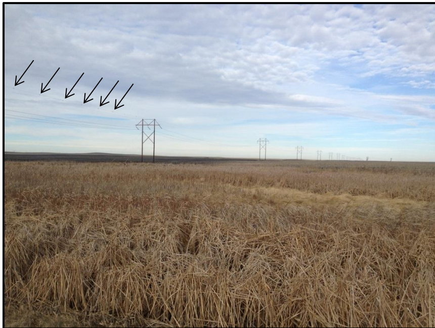
Photo 4. Direction: North/Northwest. View of the transmission line spanning a wetland area; no sedimentation or disturbance to the wetland was noted. Bird diverters were evident, although only faintly visible in this photo (shown by black arrows).
