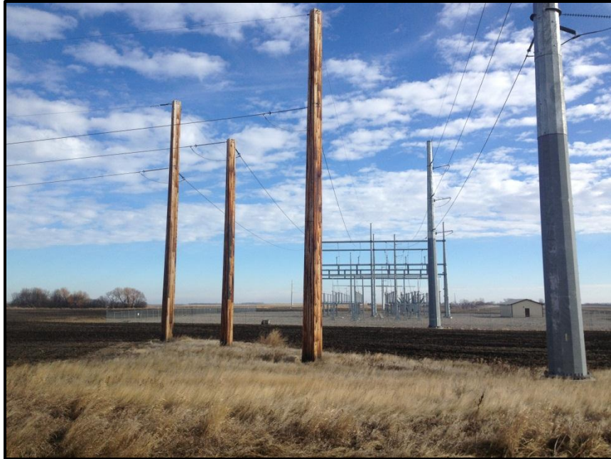
Photo 1. Direction: East. View of the beginning of the transmission line (wooden poles) at the Pillsbury substation.
