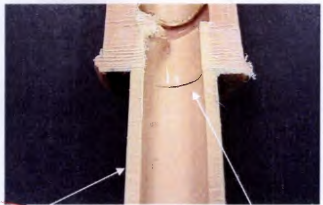
Service line interior stress fracture Photo #14
