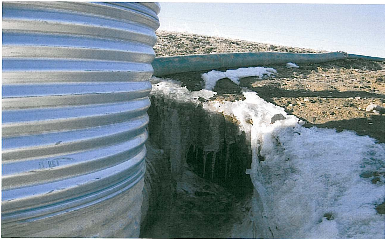
Photo #1- Piping feature on upstream slope of embankment.
