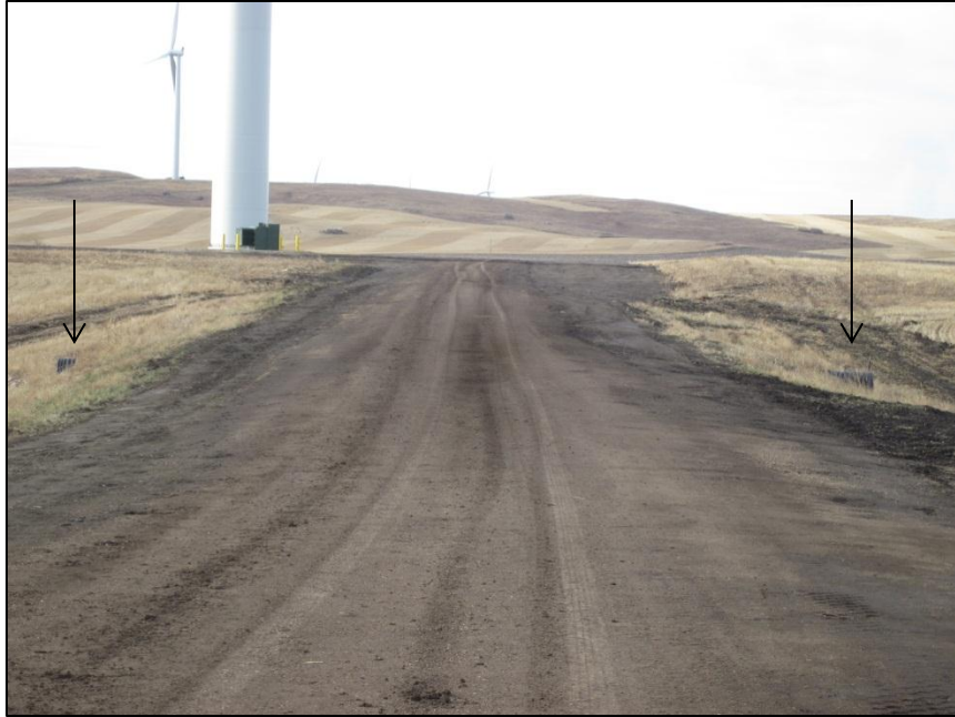
Photo 5. Direction: South. Access road to Structure 28. Note culverts in place along roadway (black arrows).
