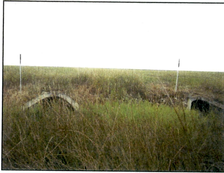
Figure 2. A representative view of WET 2 to the north of U.S. Highway 2. Note the two concrete culverts in the foreground.
