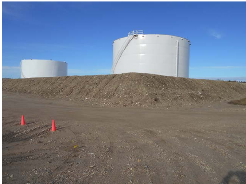
Photo 2 – Direction: North– Oil Tank Battery (Bridger Facility) served by Hawthorn Pipeline located just south of Highway 2, Stanley, ND
