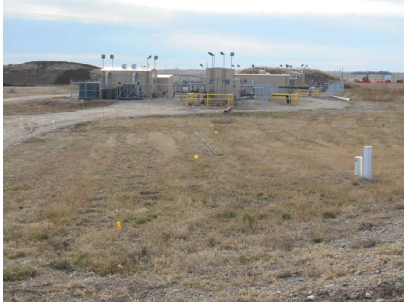
Photo 1 – Direction: South – Stanley Pipeline/ Valve Stations
