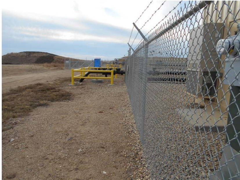
Photo 3 – Direction: South – Showing perimeter fence surrounding valve stations. Valve station gates were also locked to prevent admittance to improper personnel. Notice: Yellow bollards surrounding above ground pipe connections at valve stations.
