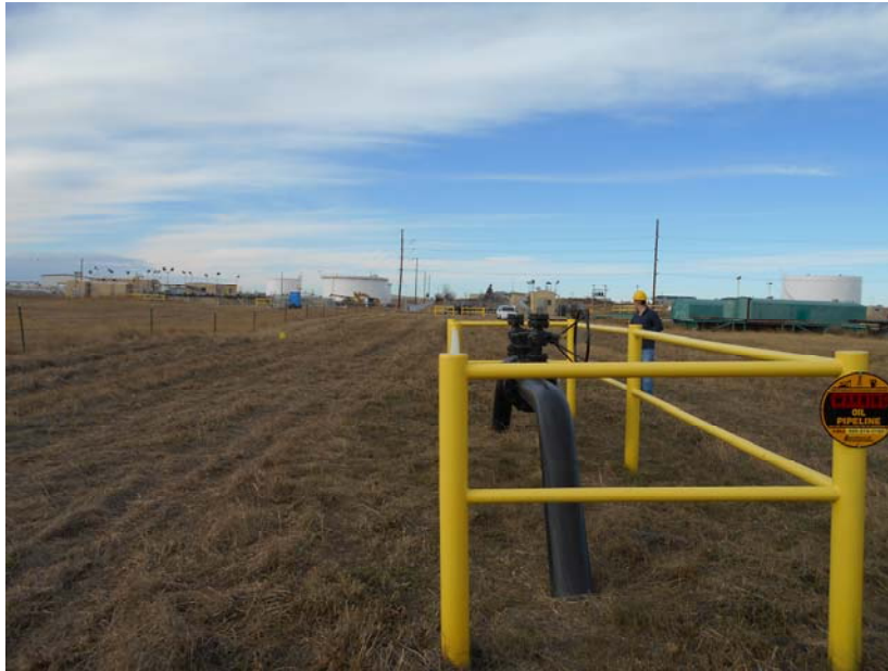
Photo 9 – Direction: West– West valve station before crossing Little Knife River.
