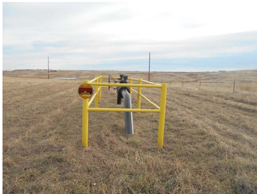
Photo 8 – Direction: East– West valve station before crossing Little Knife River.
