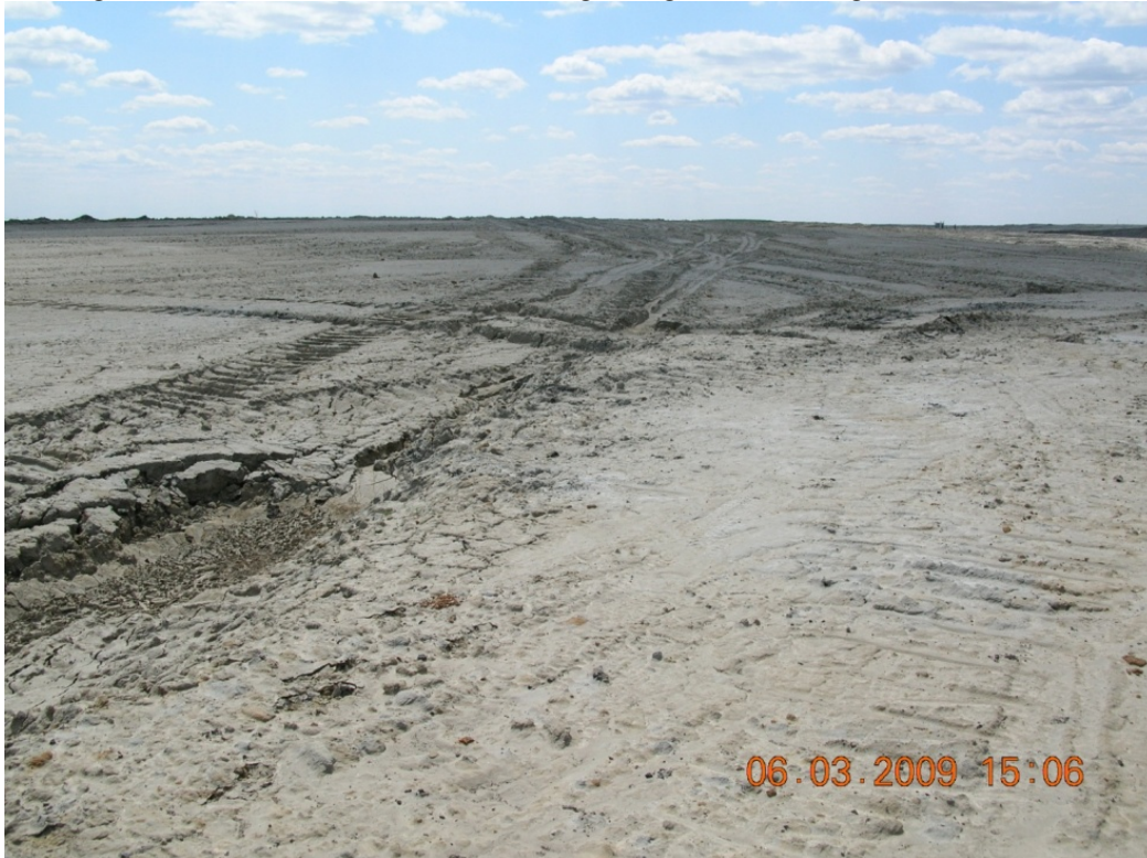
Looking west at ruts and differential settling along the north edge of GA W28A.
