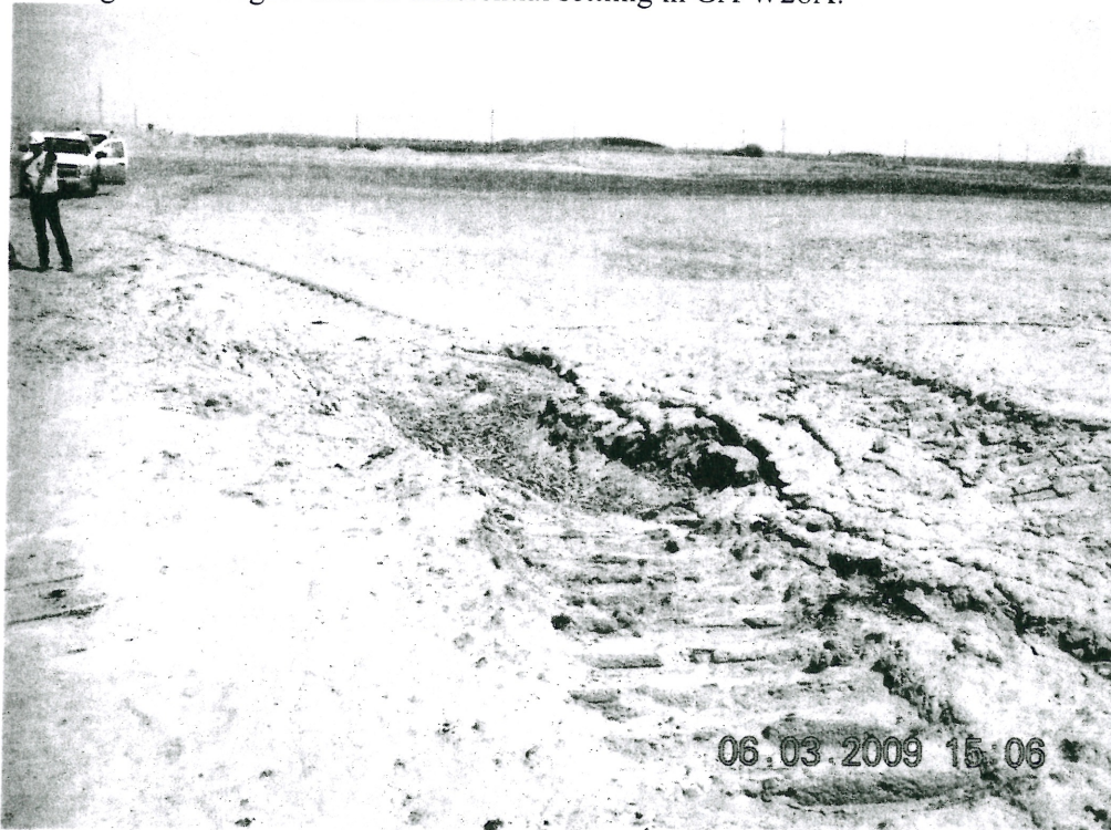
Looking east at largest area of differential settling in GA W28A.
