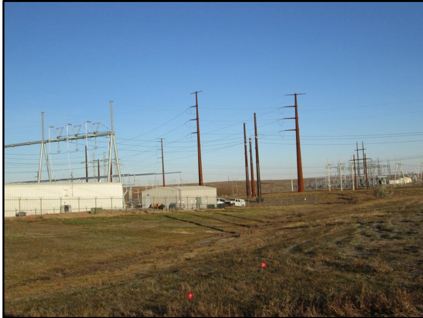
Photo 1. Direction: North/Northwest. View of the transmission line (monopole structures) on the east end of the route at the Square Butte substation.
