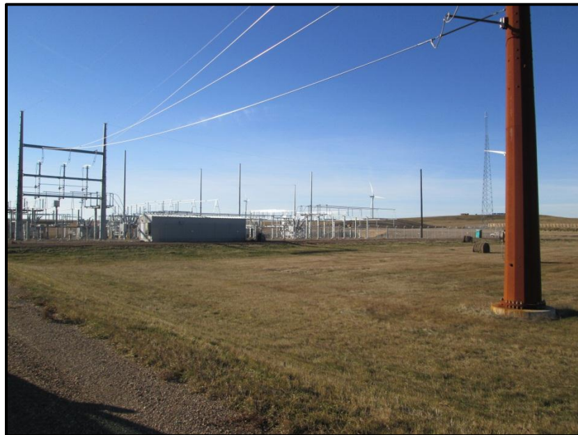
Photo 8. Direction: South/Southwest. View of the transmission line at the Bison Substation on the west end of the route.
