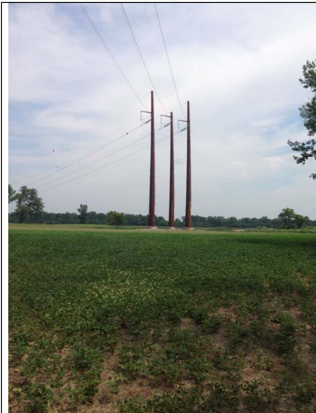
Photo 1: Pole 69 on the west side of the Missouri River. Shield markers have been installed, and can be seen in this photo.
