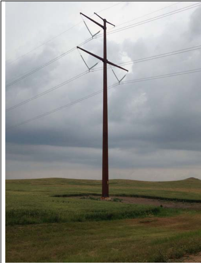
Photo 5: Typical photo of a pole constructed in agriculture land. Pole 86.
