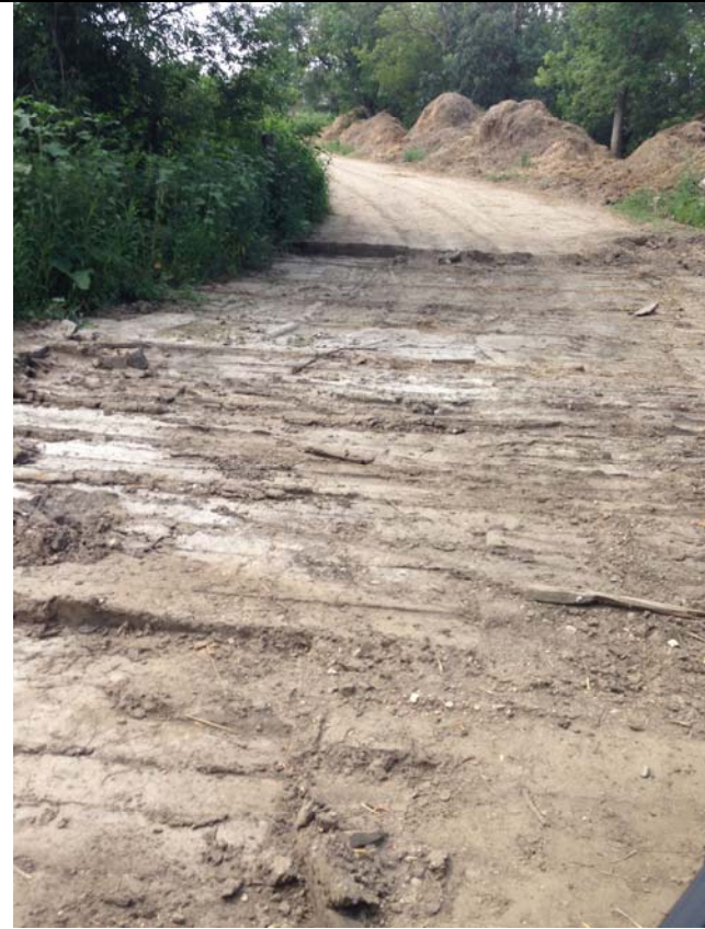
Photo 3: Adjacent to pole 68, showing rutting from recently removed construction matting within a wetland. This area will require further restoration.
