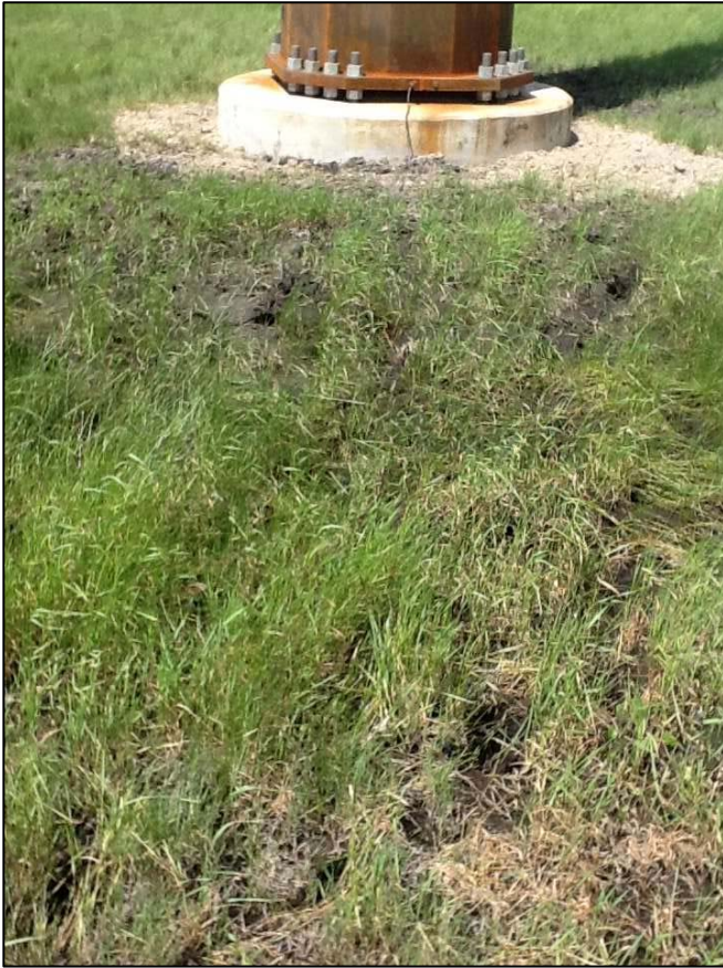
Photo 3: Example construction rutting (Pole 1272)
