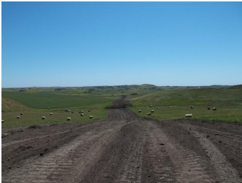
Photo 128. Direction: South. This photo shows the right-of-way for the Bridger Pipeline. At the time of our site visit the right-of-way needed final restoration.
