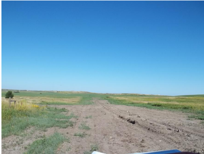
Photo 83. Direction: Northwest. This photo shows the right-of-way for the Bridger Pipeline. At the time of our site visit the right-of-way needed final restoration.
