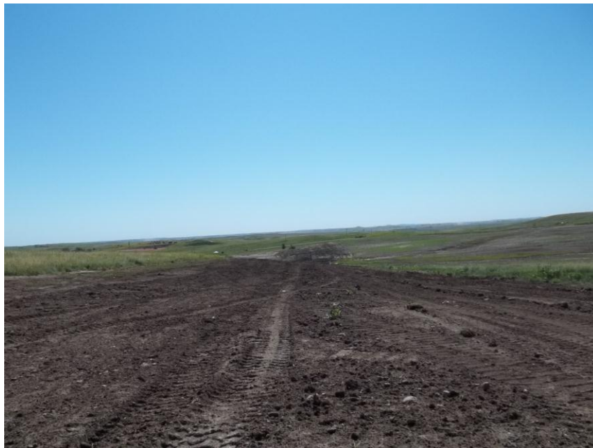
Photo 108. Direction: South. This photo shows the right-of-way for the Bridger Pipeline. At the time of our site visit the right-of-way needed final restoration.
