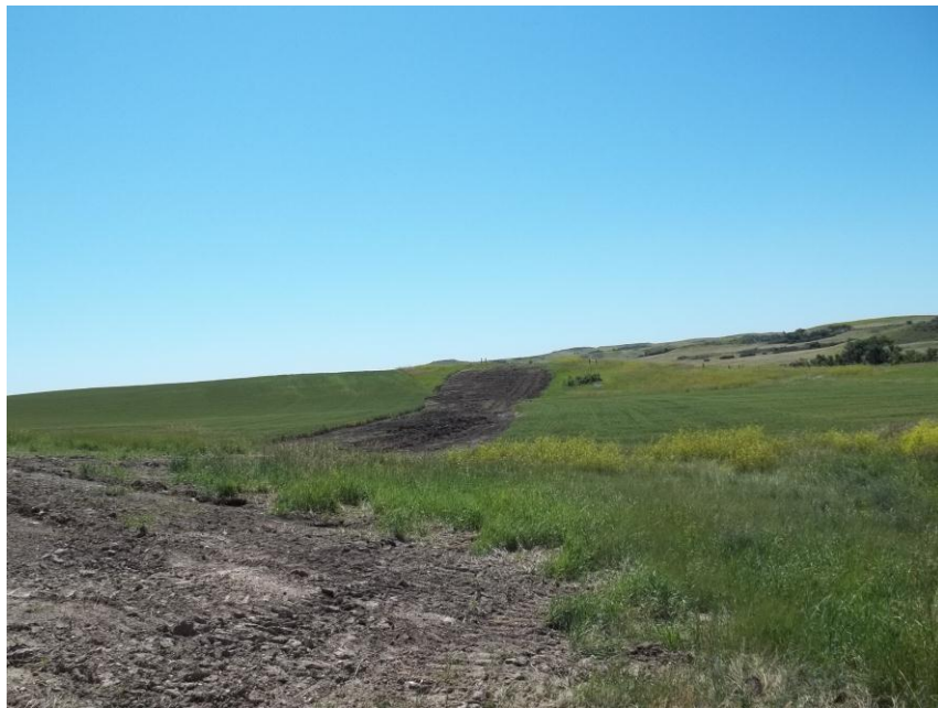
Photo 122. Direction: South. This photo shows the right-of-way for the Bridger Pipeline. At the time of our site visit the right-of-way needed final restoration.
