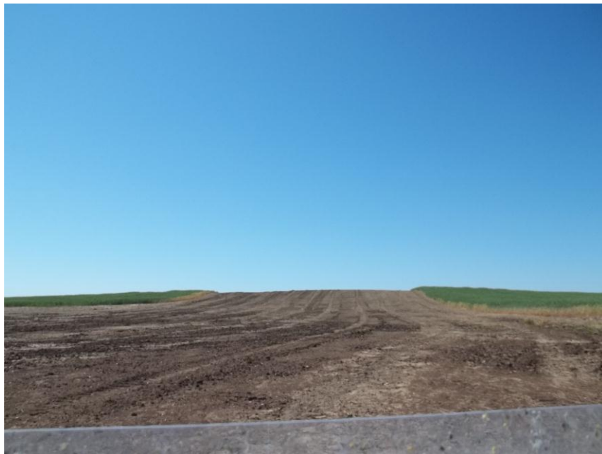
Photo 104. Direction: South. This photo shows the right-of-way for the Bridger Pipeline. At the time of our site visit the right-of-way needed final restoration.
