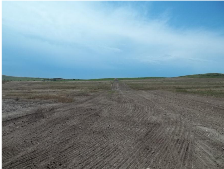
Photo 25. Direction: South. This photo shows the right-of-way for the Bridger Pipeline. At the time of our site visit the right-of-way needed final restoration.
