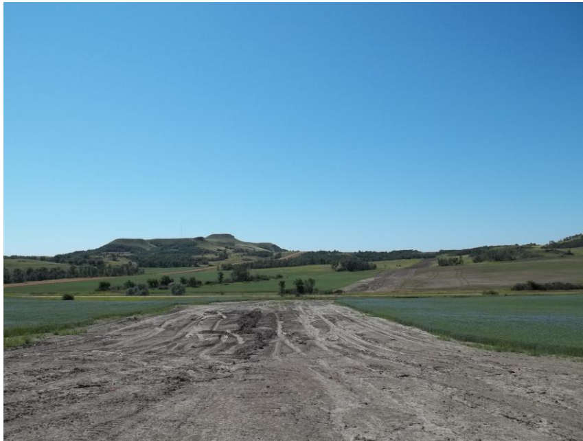
Photo 100. Direction: South. This photo shows the right-of-way for the Bridger Pipeline. At the time of our site visit the right-of-way needed final restoration.
