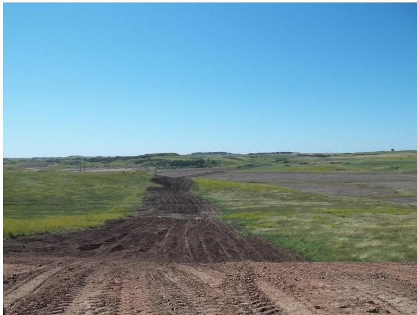
Photo 112. Direction: South. This photo shows the right-of-way for the Bridger Pipeline. At the time of our site visit the right-of-way needed final restoration.
