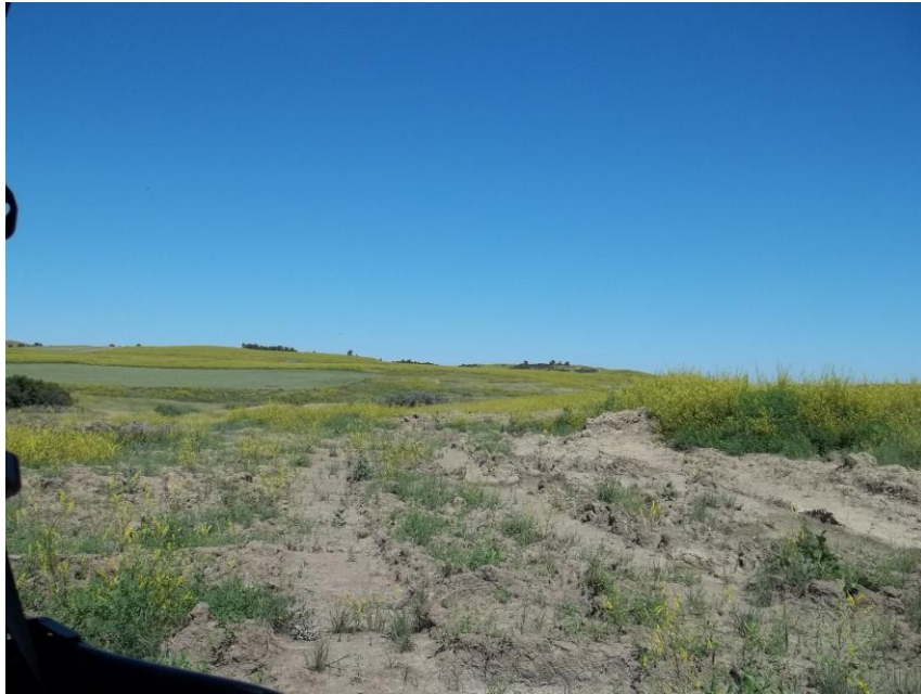
Photo 131. Direction: Northeast. This photo shows the right-of-way for the Bridger Pipeline. At the time of our site visit the right-of-way needed final restoration.
