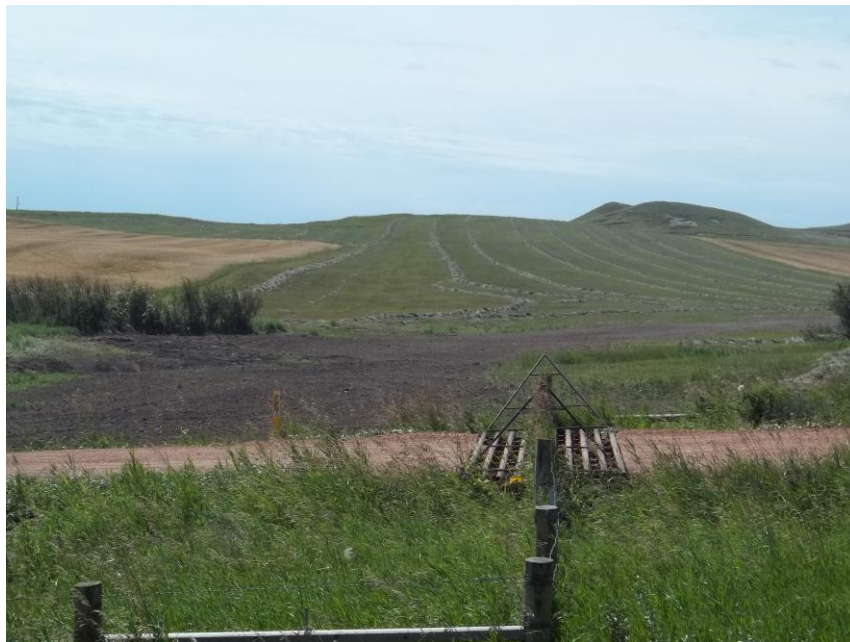
Photo 34. Direction: South. This photo shows the right-of-way for the Bridger Pipeline. At the time of our site visit the right-of-way needed final restoration.
