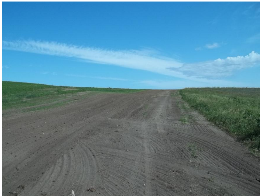
Photo 18. Direction: North. This photo shows the right-of-way for the Bridger Pipeline. At the time of our site visit the right-of-way needed final restoration.
