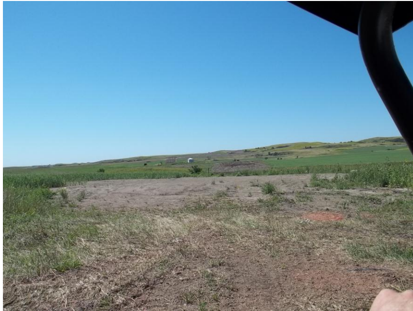
Photo 107. Direction: South. This photo shows the right-of-way for the Bridger Pipeline. At the time of our site visit the right-of-way needed final restoration.
