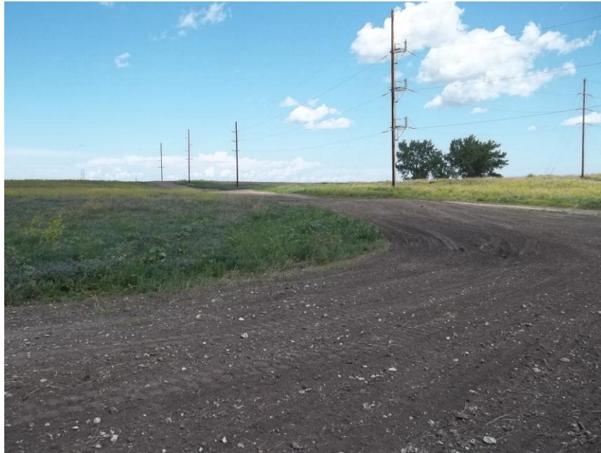
Photo 39. Direction: North. This photo shows the right-of-way for the Bridger Pipeline. At the time of our site visit the right-of-way needed final restoration.
