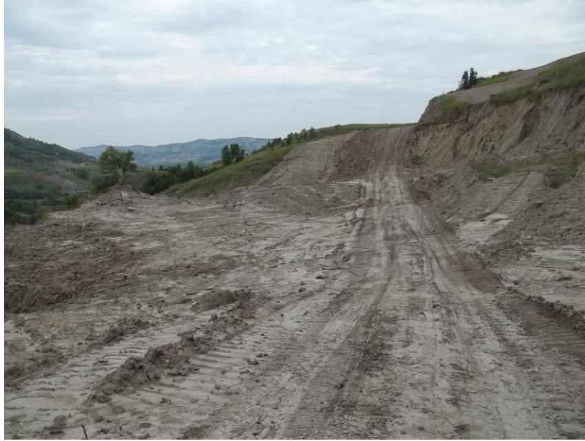
Photo 63. Direction: North. This photo shows the right-of-way for the Bridger Pipeline. At the time of our site visit the right-of-way needed final restoration.
