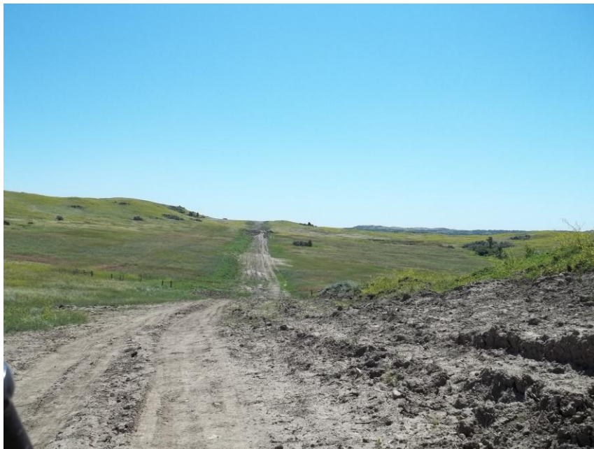
Photo 132. Direction: South. This photo shows the right-of-way for the Bridger Pipeline. At the time of our site visit the right-of-way needed final restoration.
