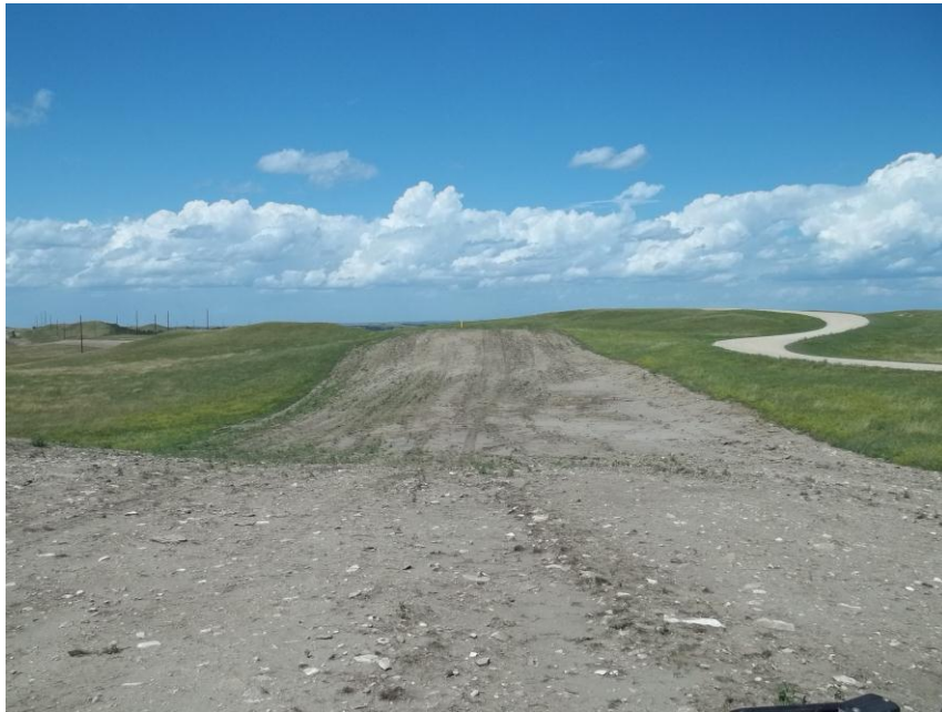
Photo 50. Direction: North. This photo shows the right-of-way for the Bridger Pipeline. At the time of our site visit the right-of-way needed final restoration.
