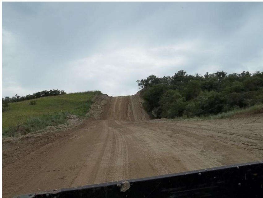
Photo 62. Direction: Southeast. This photo shows the right-of-way for the Bridger Pipeline. At the time of our site visit the right-of-way needed final restoration.
