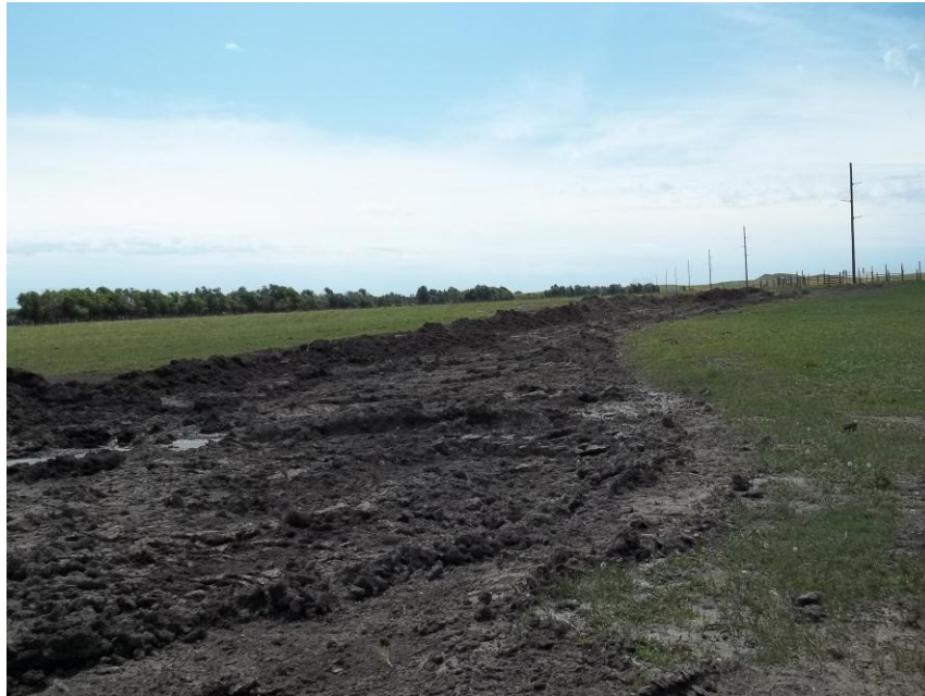
Photo 35. Direction: South. This photo shows the right-of-way for the Bridger Pipeline. At the time of our site visit the area shown needed topsoil spread for a total segment length of approximately 1,500 feet and final restoration.
