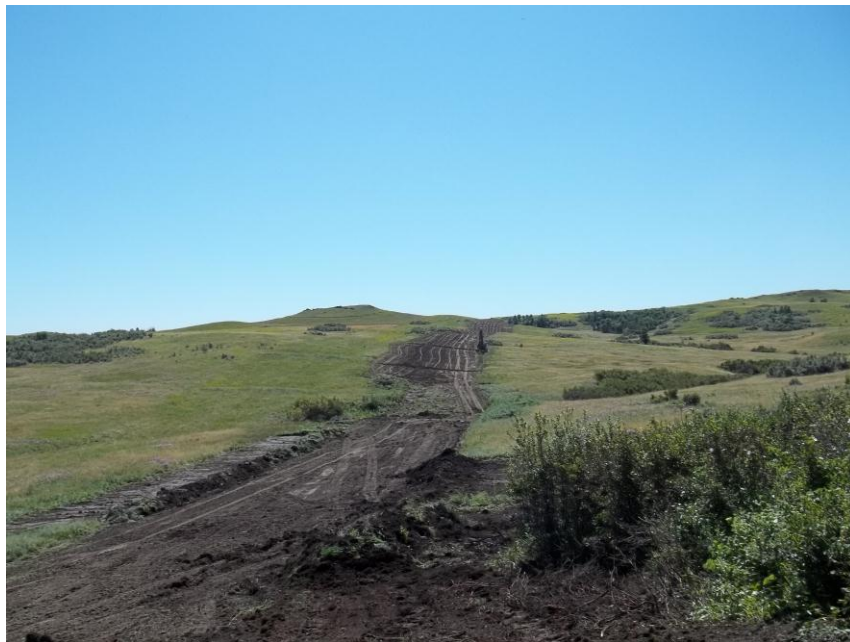
Photo 126. Direction: South. This photo shows the right-of-way for the Bridger Pipeline. At the time of our site visit the right-of-way needed final restoration.
