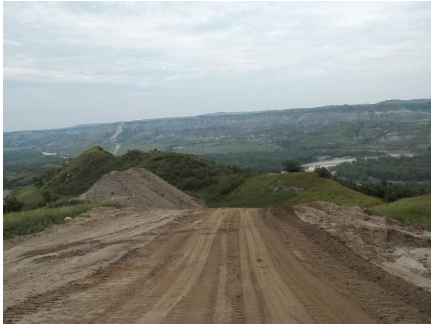
Photo 61. Direction: Northwest. This photo shows the right-of-way for the Bridger Pipeline. At the time of our site visit the right-of-way needed final restoration.
