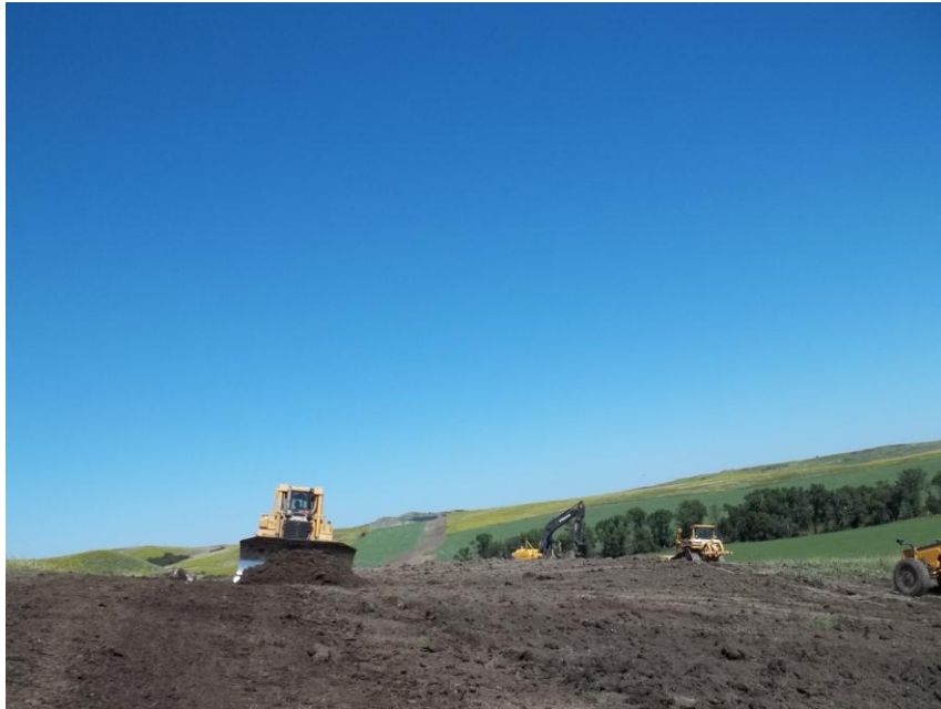
Photo 127. Direction: North. This photo shows the right-of-way for the Bridger Pipeline. At the time of our site visit the right-of-way needed final restoration.
