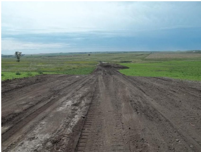
Photo 20. Direction: South. This photo shows the right-of-way for the Bridger Pipeline. At the time of our site visit the right-of-way needed final restoration.
