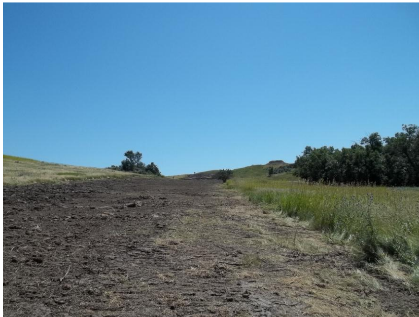
Photo 138. Direction: South. This photo shows the right-of-way for the Bridger Pipeline. At the time of our site visit the right-of-way needed final restoration.
