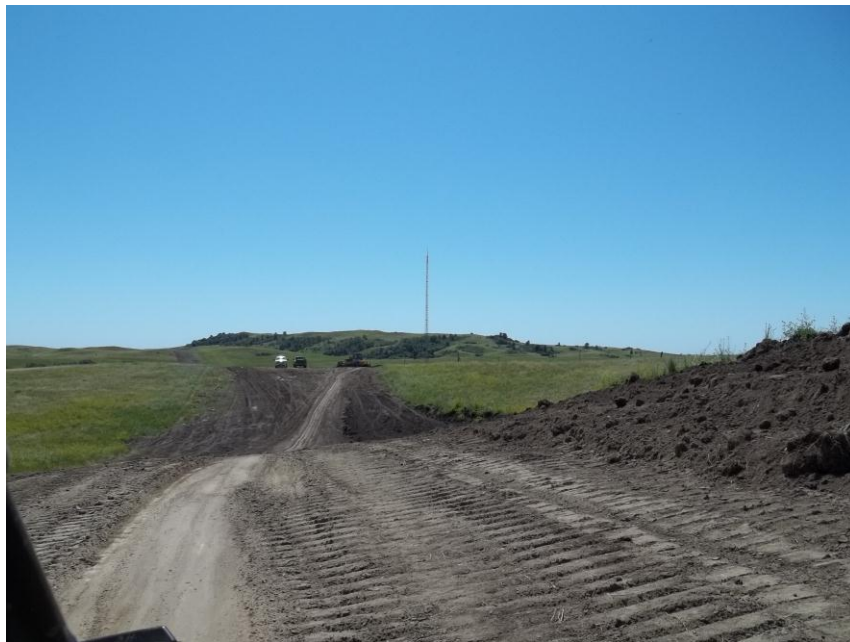
Photo 140. Direction: Southwest. This photo shows the right-of-way for the Bridger Pipeline. At the time of our site visit the right-of-way needed final restoration.
