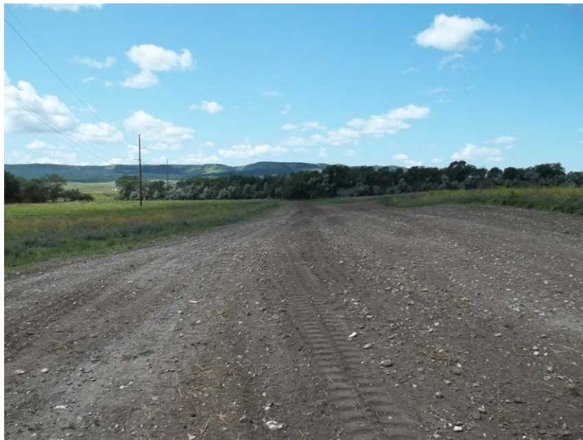
Photo 38. Direction: West. This photo shows the right-of-way for the Bridger Pipeline. At the time of our site visit the right-of-way needed final restoration.
