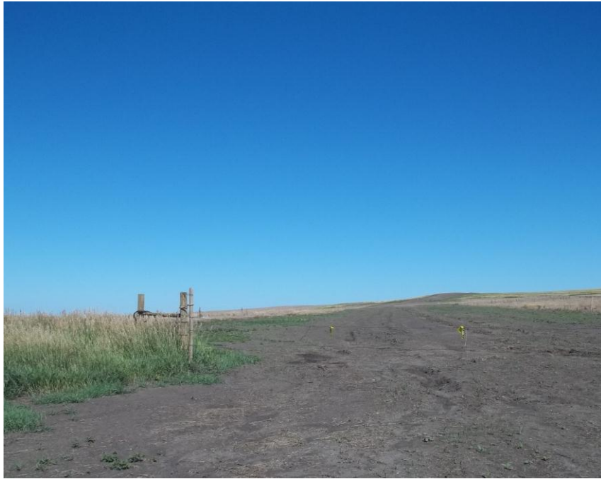
Photo 89. Direction: North. This photo shows the right-of-way for the Bridger Pipeline. At the time of our site visit the right-of-way needed final restoration.
