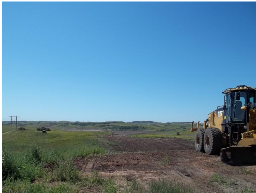
Photo 110. Direction: South. This photo shows the right-of-way for the Bridger Pipeline. At the time of our site visit the right-of-way needed final restoration
