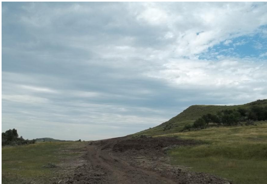
Photo 78. Direction: North. This photo shows the right-of-way for the Bridger Pipeline. At the time of our site visit the right-of-way needed final restoration.
