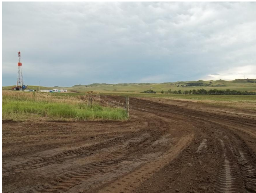
Photo 14. Direction: Southwest. This photo shows the right-of-way for the Bridger Pipeline. At the time of our site visit the right-of-way needed final restoration.
