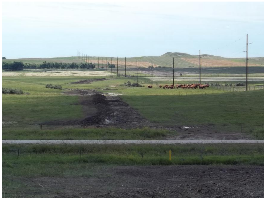
Photo 36. Direction: South. This photo shows the right-of-way for the Bridger Pipeline. At the time of our site visit the area shown needed topsoil spread and final restoration.
