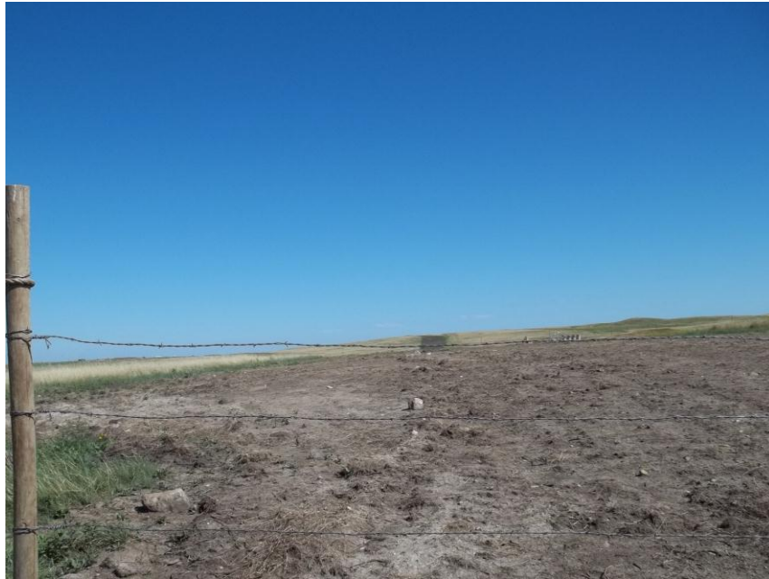
Photo 87. Direction: North. This photo shows the right-of-way for the Bridger Pipeline. At the time of our site visit the right-of-way needed final restoration.
