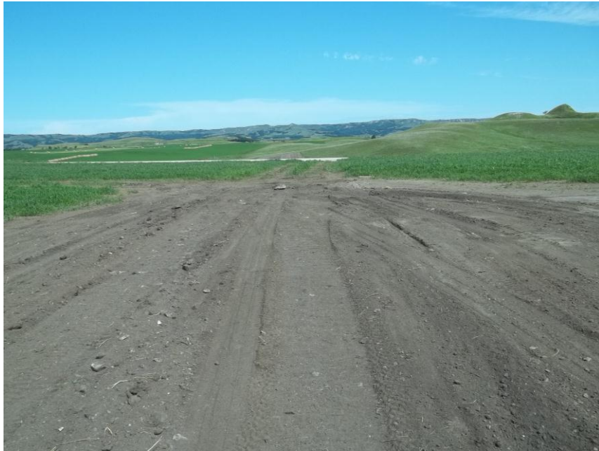
Photo 21. Direction: North. This photo shows the right-of-way for the Bridger Pipeline. At the time of our site visit the right-of-way needed final restoration.
