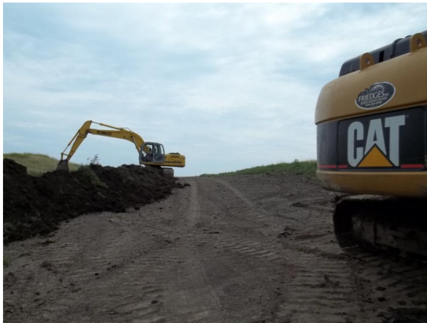
Photo 60. Direction: Northwest. This photo shows the right-of-way for the Bridger Pipeline. At the time of our site visit the right-of-way needed final restoration.
