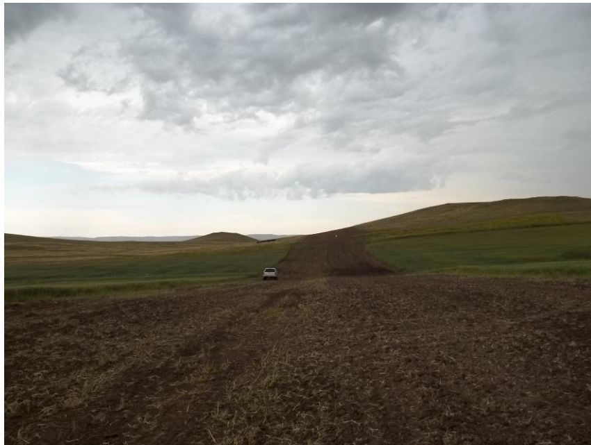
Photo 10. Direction: North. This photo shows the right-of-way for the Bridger Pipeline. At the time of our site visit the right-of-way needed final restoration.
