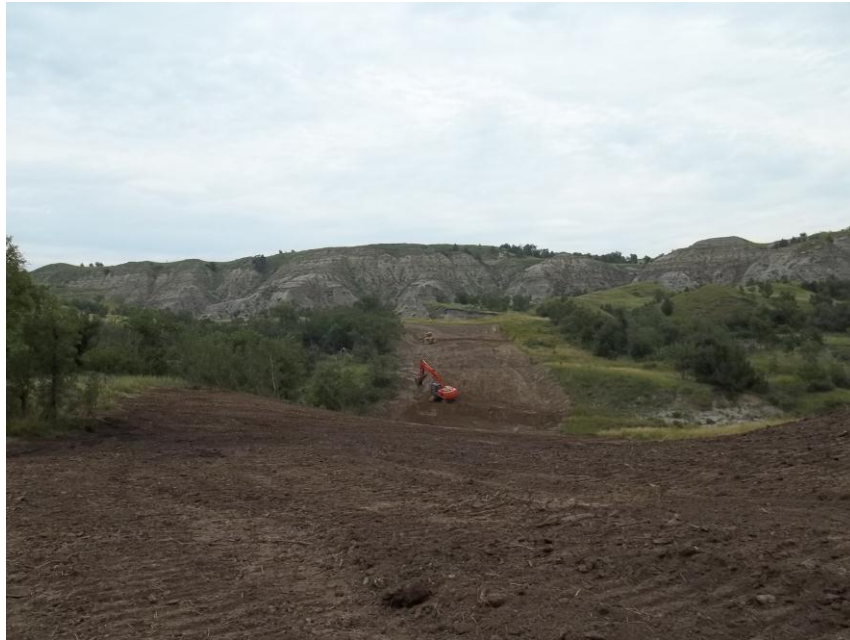
Photo 57. Direction: Northwest. This photo shows the right-of-way for the Bridger Pipeline. At the time of our site visit the right-of-way needed final restoration.
