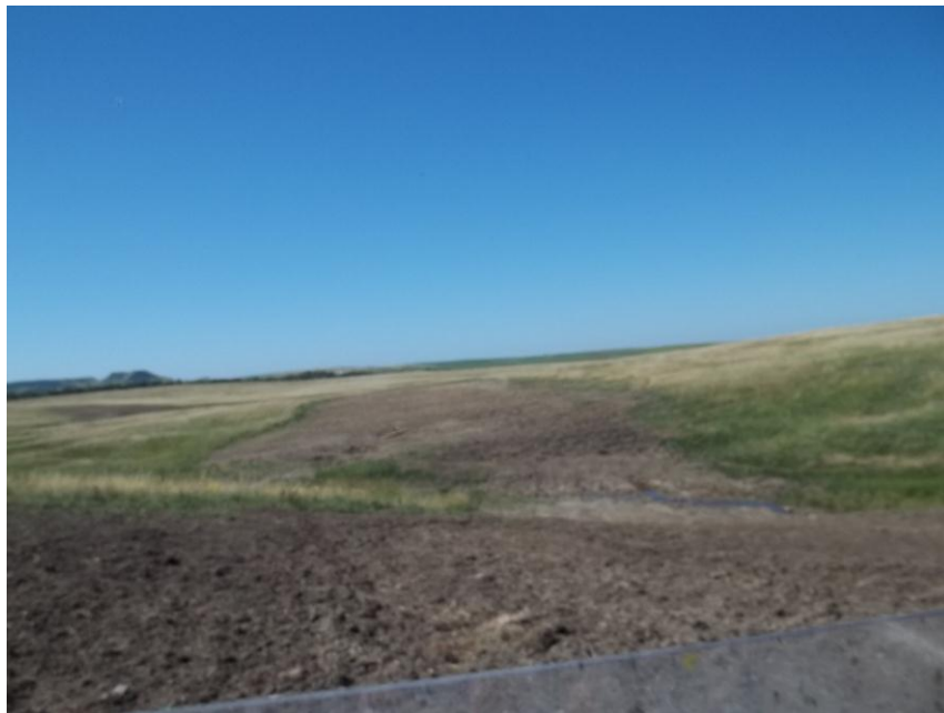
Photo 92. Direction: South. This photo shows the right-of-way for the Bridger Pipeline. At the time of our site visit the right-of-way needed final restoration.
