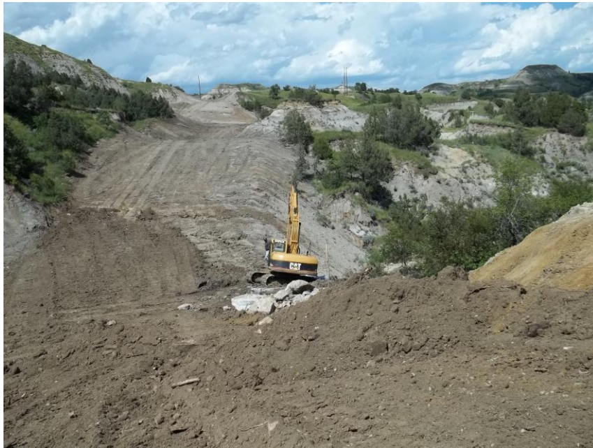
Photo 56. Direction: North. This photo shows the right-of-way for the Bridger Pipeline. At the time of our site visit the right-of-way needed final restoration.
