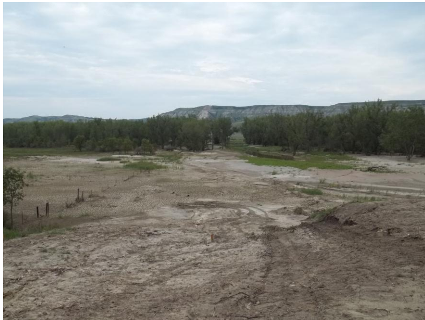
Photo 64. Direction: North. This photo shows the right-of-way for the Bridger Pipeline. At the time of our site visit the area shown had wet soil conditions and needed final restoration.
