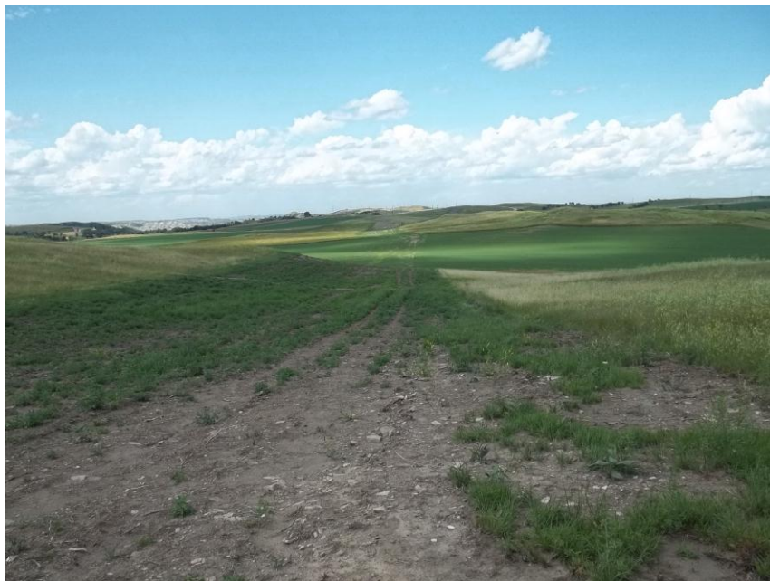
Photo 48. Direction: North. This photo shows the right-of-way for the Bridger Pipeline. At the time of our site visit the right-of-way needed final restoration.
