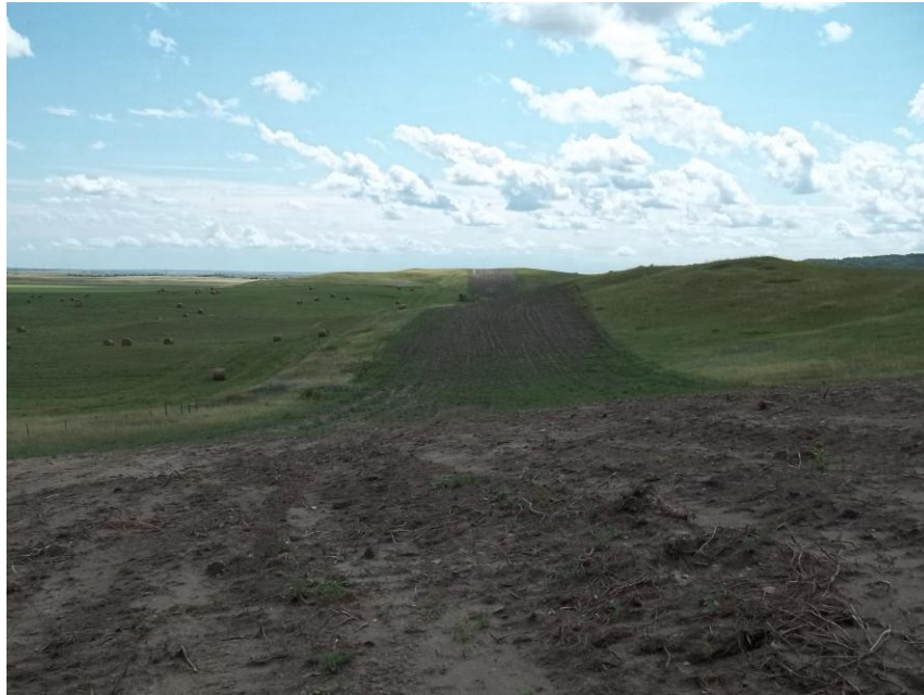
Photo 47. Direction: South. This photo shows the right-of-way for the Bridger Pipeline. At the time of our site visit the right-of-way needed final restoration.
