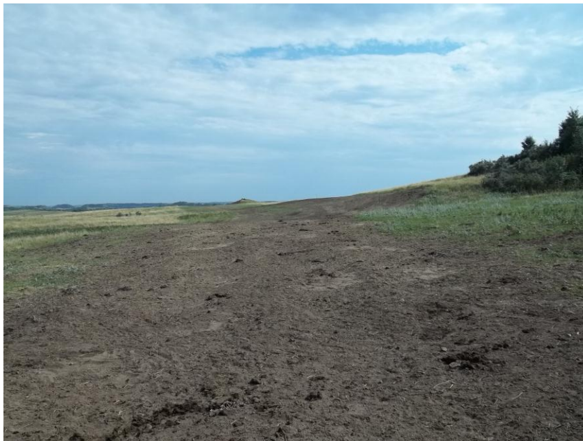
Photo 76. Direction: South. This photo shows the right-of-way for the Bridger Pipeline. At the time of our site visit the right-of-way needed final restoration.
