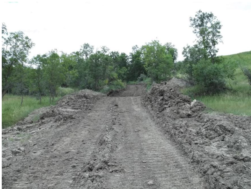
Photo 79. Direction: South. This photo shows the right-of-way for the Bridger Pipeline. At the time of our site visit the area shown needed topsoil spread and final restoration.
