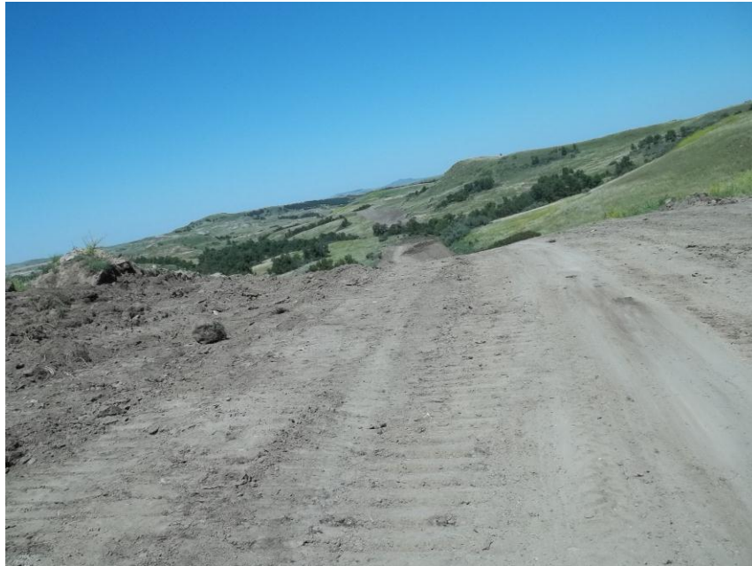
Photo 141. Direction: Northeast. This photo shows the right-of-way for the Bridger Pipeline. At the time of our site visit the right-of-way needed topsoil spread and final restoration.
