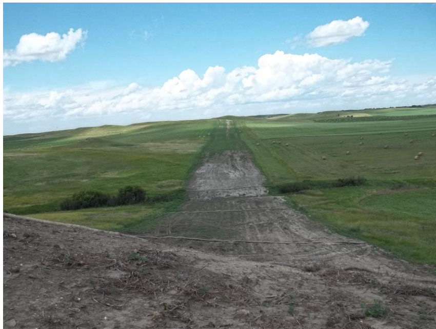
Photo 46. Direction: North. This photo shows the right-of-way for the Bridger Pipeline. At the time of our site visit the right-of-way needed final restoration.
