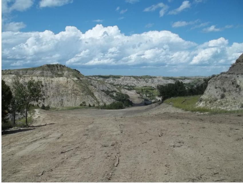
Photo 55. Direction: North. This photo shows the right-of-way for the Bridger Pipeline. At the time of our site visit the right-of-way needed final restoration.
