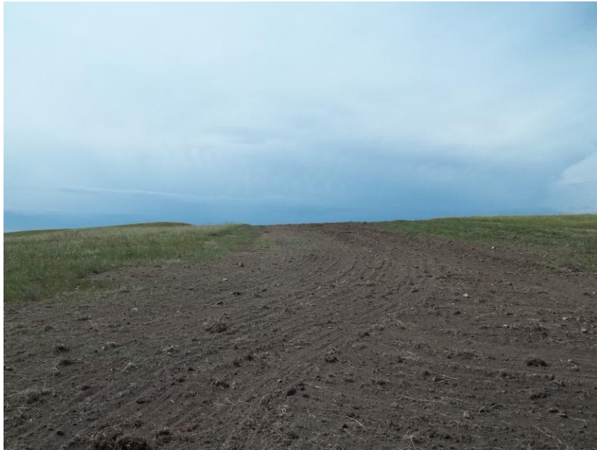
Photo 19. Direction: South. This photo shows the right-of-way for the Bridger Pipeline. At the time of our site visit the right-of-way needed final restoration.
