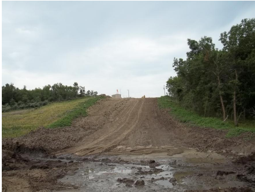
Photo 59. Direction: Southeast. This photo shows the right-of-way for the Bridger Pipeline. At the time of our site visit the area shown was wet and needed final restoration.
