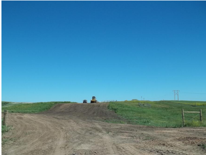
Photo 113. Direction: North. This photo shows the right-of-way for the Bridger Pipeline. At the time of our site visit the right-of-way needed final restoration.
