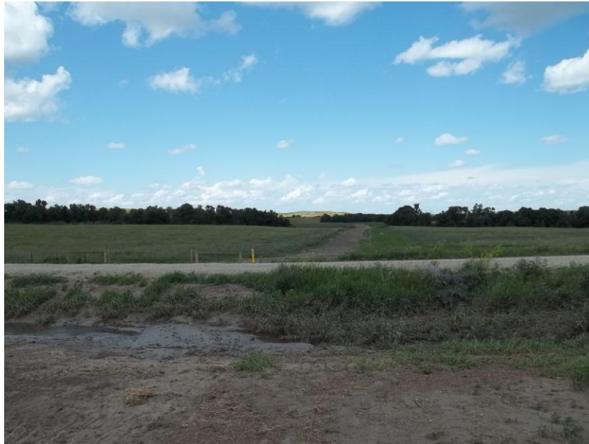
Photo 41. Direction: North. This photo shows the right-of-way for the Bridger Pipeline. At the time of our site visit the right-of-way needed final restoration.
