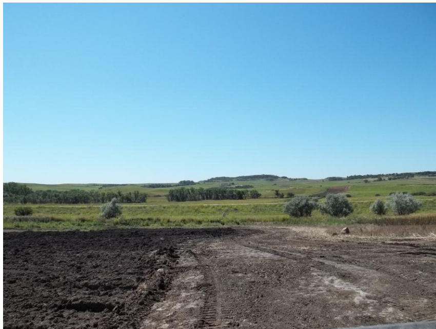
Photo 114. Direction: South. This photo shows the right-of-way for the Bridger Pipeline. At the time of our site visit the right-of-way needed final restoration.
