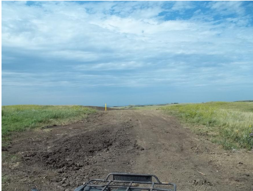
Photo 77. Direction: North. This photo shows the right-of-way for the Bridger Pipeline. At the time of our site visit the right-of-way needed final restoration.
