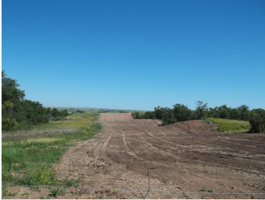
Photo 105. Direction: North. This photo shows the right-of-way for the Bridger Pipeline. At the time of our site visit the right-of-way needed final restoration.
