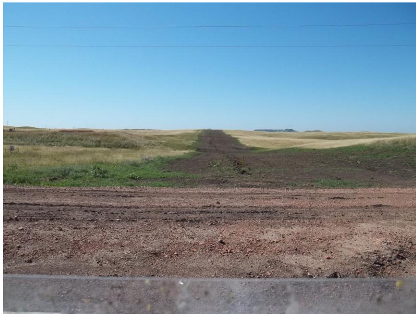
Photo 84. Direction: South. This photo shows the right-of-way for the Bridger Pipeline. At the time of our site visit the right-of-way needed final restoration.
