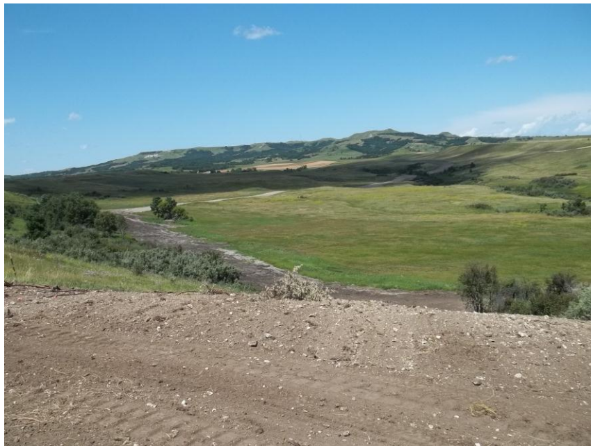
Photo 40. Direction: Northwest. This photo shows the right-of-way for the Bridger Pipeline. At the time of our site visit the area shown needed topsoil spread and final restoration.
