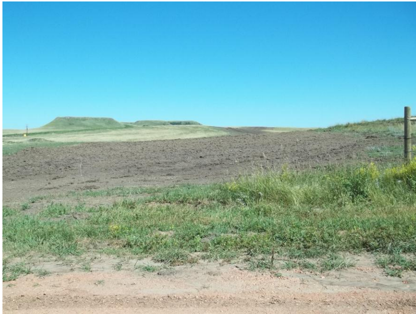
Photo 106. Direction: North. This photo shows the right-of-way for the Bridger Pipeline. At the time of our site visit the right-of-way needed final restoration.
