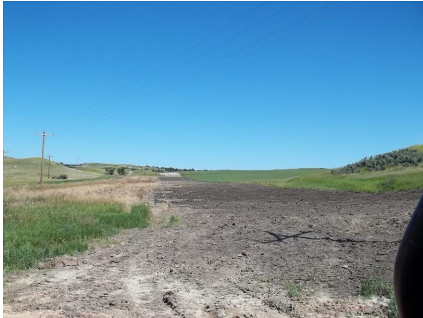
Photo 123. Direction: North. This photo shows the right-of-way for the Bridger Pipeline. At the time of our site visit the right-of-way needed final restoration.
