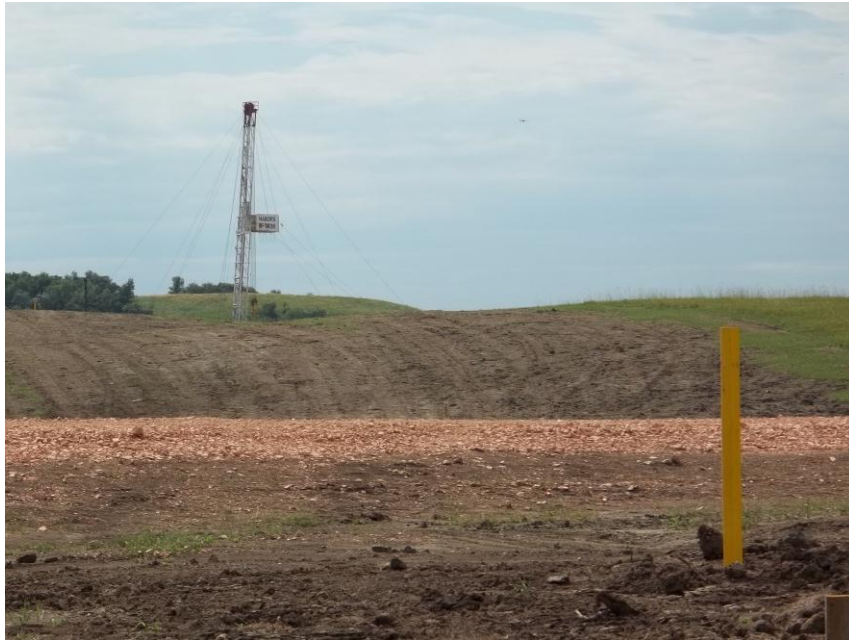
Photo 73. Direction: South. This photo shows the right-of-way for the Bridger Pipeline. At the time of our site visit the right-of-way needed final restoration.
