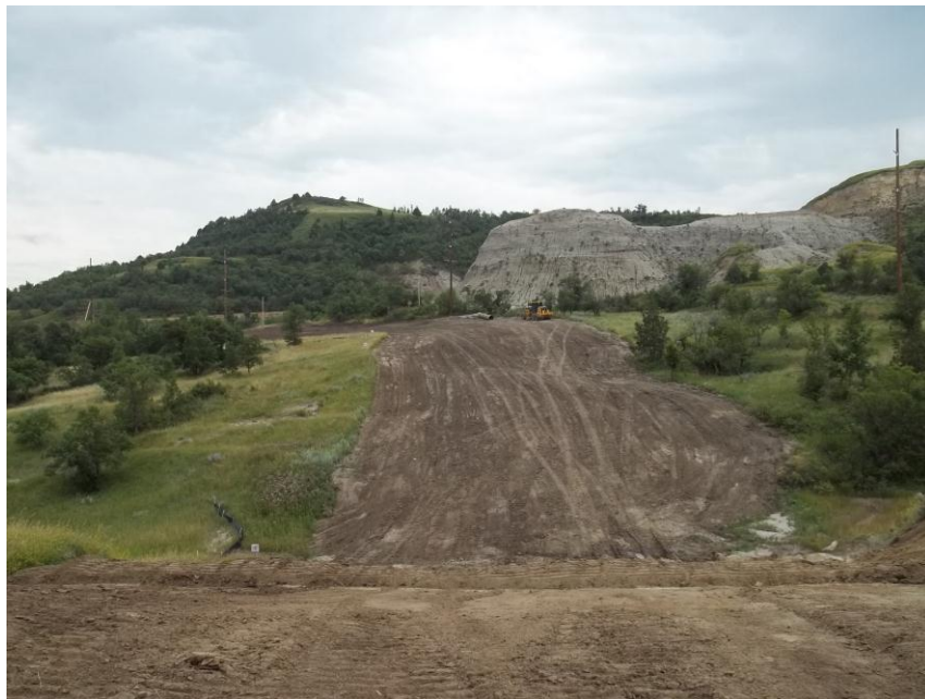
Photo 58. Direction: Southeast. This photo shows the right-of-way for the Bridger Pipeline. At the time of our site visit the right-of-way needed final restoration.
