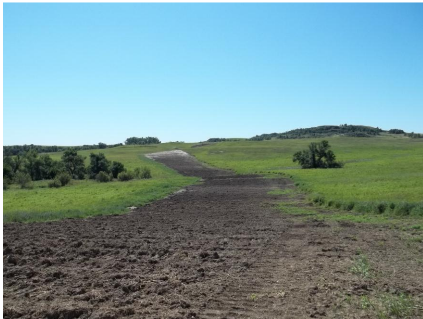
Photo 116. Direction: South. This photo shows the right-of-way for the Bridger Pipeline. At the time of our site visit the right-of-way needed final restoration.
