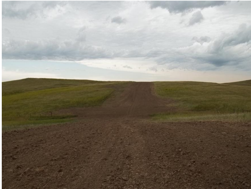
Photo 13. Direction: North. This photo shows the right-of-way for the Bridger Pipeline. At the time of our site visit the right-of-way needed final restoration.
