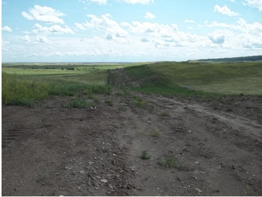
Photo 49. Direction: South. This photo shows the right-of-way for the Bridger Pipeline. At the time of our site visit the right-of-way needed final restoration.
