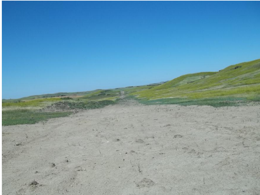
Photo 135. Direction: North. This photo shows the right-of-way for the Bridger Pipeline. At the time of our site visit the right-of-way needed final restoration.
