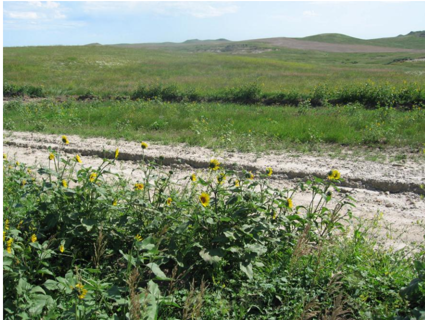
Photo 5. Direction: Northeast. This photo shows the right-of-way for the Bridger Pipeline. At the time of our site visit there was a one foot deep trench above the pipeline and the right-of-way needed final restoration.
