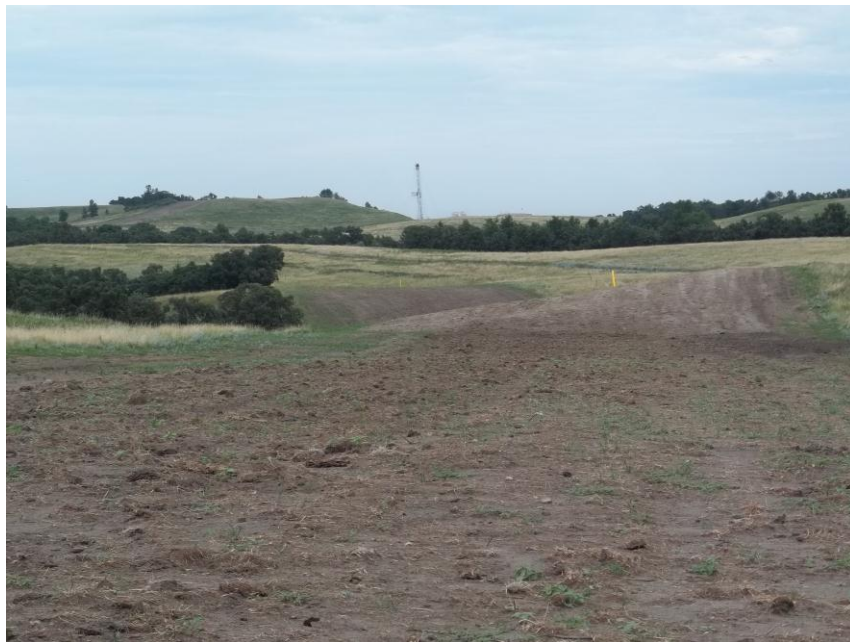
Photo 70. Direction: North. This photo shows the right-of-way for the Bridger Pipeline. At the time of our site visit the right-of-way needed final restoration.
