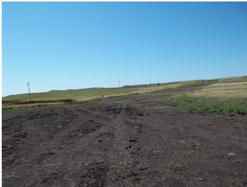
Photo 88. Direction: South. This photo shows the right-of-way for the Bridger Pipeline. At the time of our site visit the right-of-way needed final restoration.
