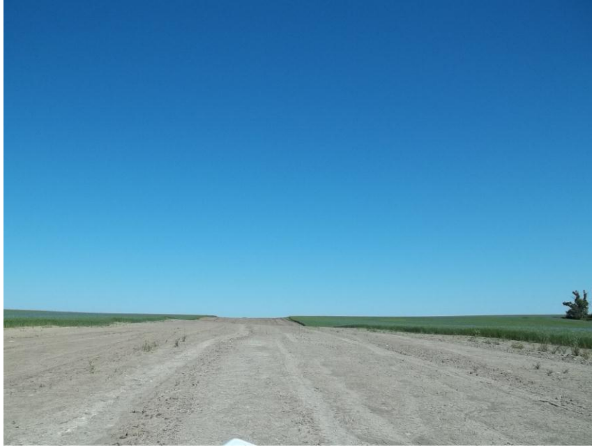
Photo 101. Direction: North. This photo shows the right-of-way for the Bridger Pipeline. At the time of our site visit the right-of-way needed final restoration.
