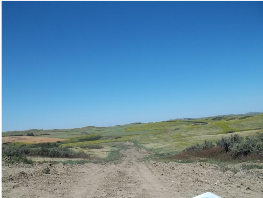
Photo 133. Direction: North. This photo shows the right-of-way for the Bridger Pipeline. At the time of our site visit the right-of-way needed final restoration.
