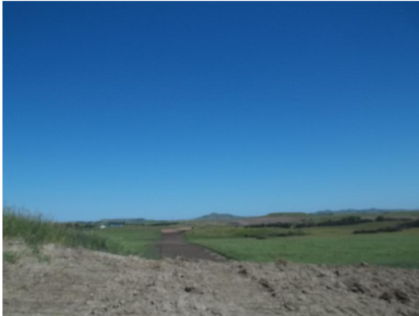
Photo 117. Direction: North. This photo shows the right-of-way for the Bridger Pipeline. At the time of our site visit the right-of-way needed final restoration.
