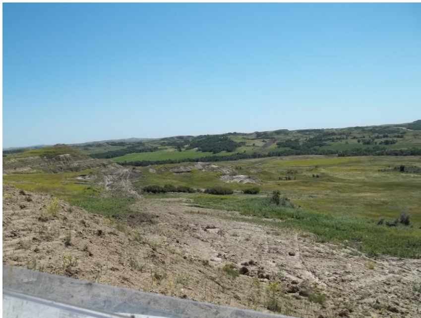
Photo 134. Direction: South. This photo shows the right-of-way for the Bridger Pipeline. At the time of our site visit the right-of-way needed final restoration.
