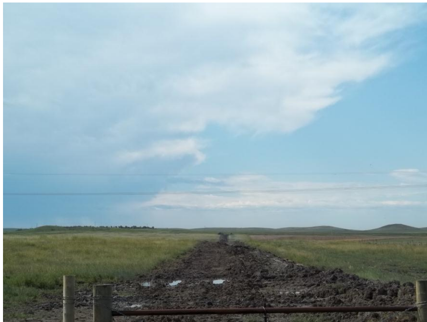
Photo 16. Direction: South. This photo shows the right-of-way for the Bridger Pipeline. At the time of our site visit the area shown had wet soil conditions, needed topsoil spread, and final restoration.
