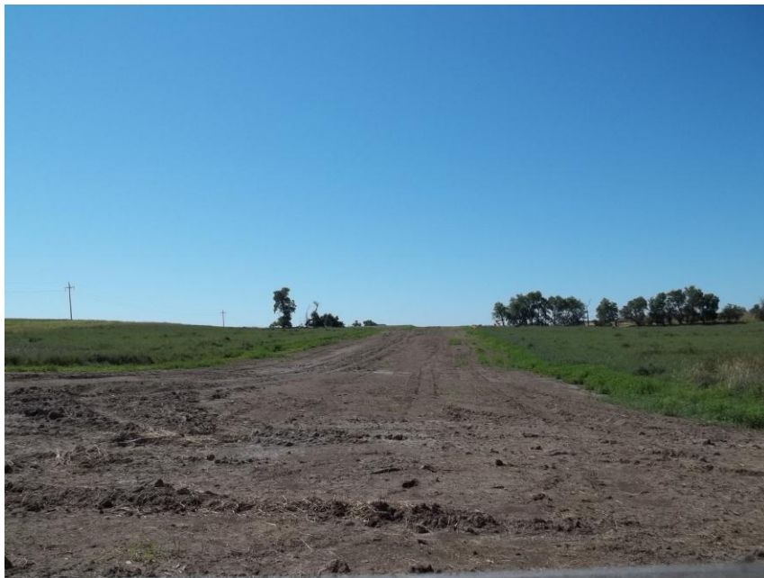
Photo 94. Direction: South. This photo shows the right-of-way for the Bridger Pipeline. At the time of our site visit the right-of-way needed final restoration.
