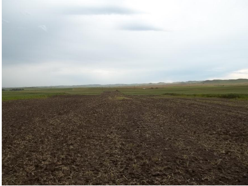
Photo 9. Direction: South. This photo shows the right-of-way for the Bridger Pipeline. At the time of our site visit the right-of-way needed final restoration.
