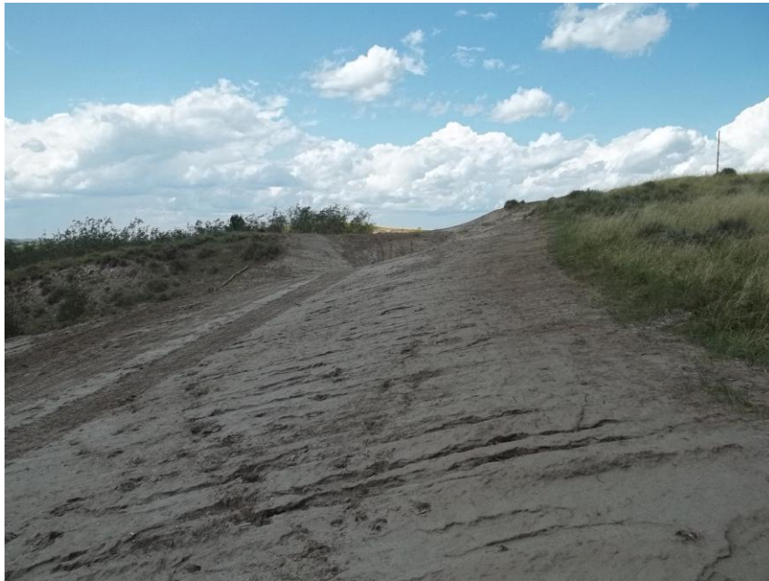
Photo 52. Direction: North. This photo shows the right-of-way for the Bridger Pipeline. At the time of our site visit the right-of-way needed final restoration.
