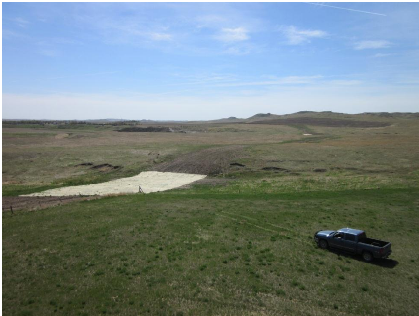
Photo 34. Direction: Southeast. Pipeline right-of-way. Grass mats had been placed for erosion control at the request of landowner.
