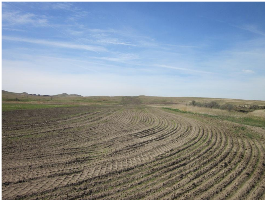
Photo 28. Direction: South. Pipeline right-of-way. This area had recently been planted by the landowner.
