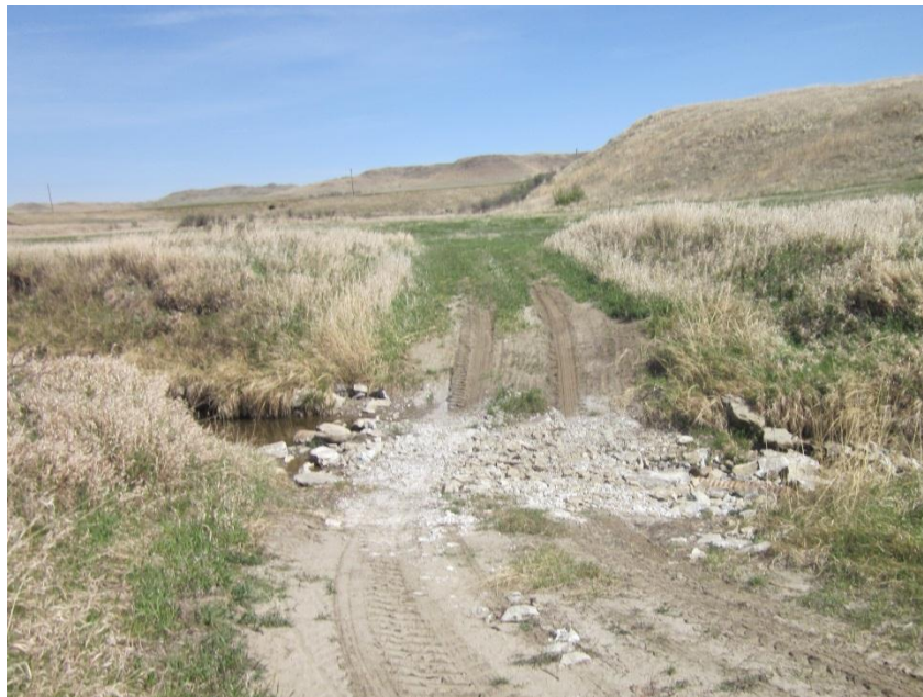
Photo 24. Direction: South. Access road for Bridger's pipeline where it crosses the Knife River. A culvert was used to preserve the waterway's natural flow patterns; no erosion or sedimentation was noted.
