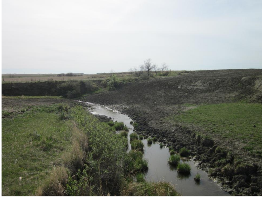
Photo 13. Direction: Southwest. Pipeline right-of-way. No erosion or sedimentation to the waterway was evident as a result of construction, but erosion controls were not in place at the time of the inspection. Steps to vegetate the slope should be done immediately to prevent erosion to the waterway
