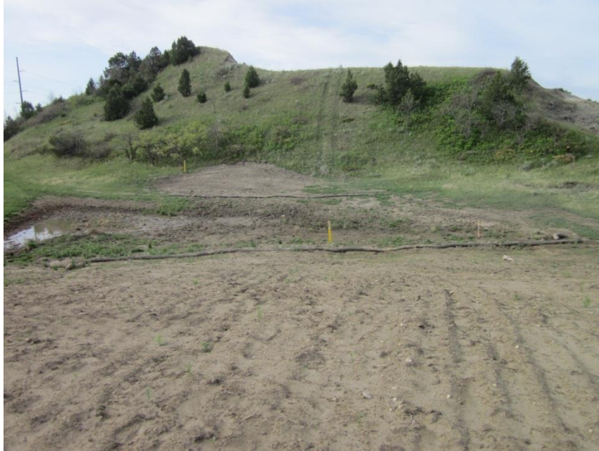
Photo 67. Direction: South. North of where Bridger’s pipeline bores under a badland butte. Note erosion control structures in place around wetland.
