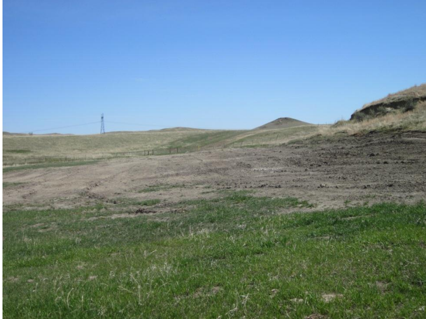
Photo 37. Direction: Northeast. Pipeline right-of-way. A seep in the side of the hill caused erosion problems during construction, but restoration appeared to have ameliorated any permanent construction impacts.
