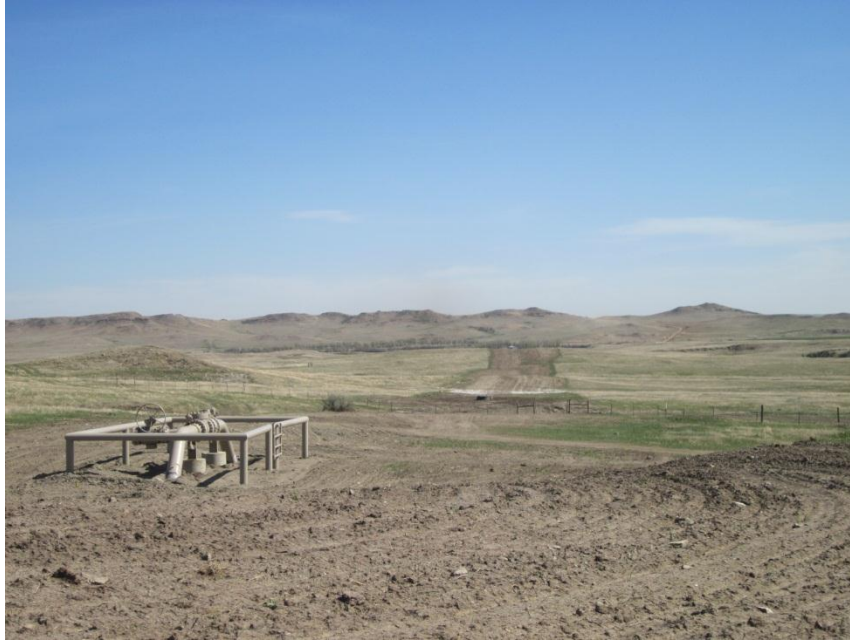
Photo 21. Direction: Southeast. Pipeline right-of-way at the 12 th St. valve setting. Reseeding had occurred, but vegetation had yet to reclaim the disturbance.
