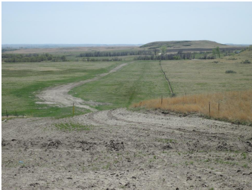
Photo 50. Direction: South. Pipeline right-of-way. Vegetated area in the right side of photo was a historic site that had been avoided.
