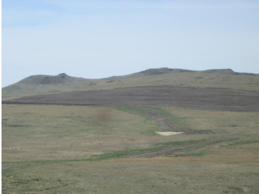
Photo 35. Direction: Southeast. Pipeline right-of-way. Grass mats had been placed for erosion control at the request of landowner.
