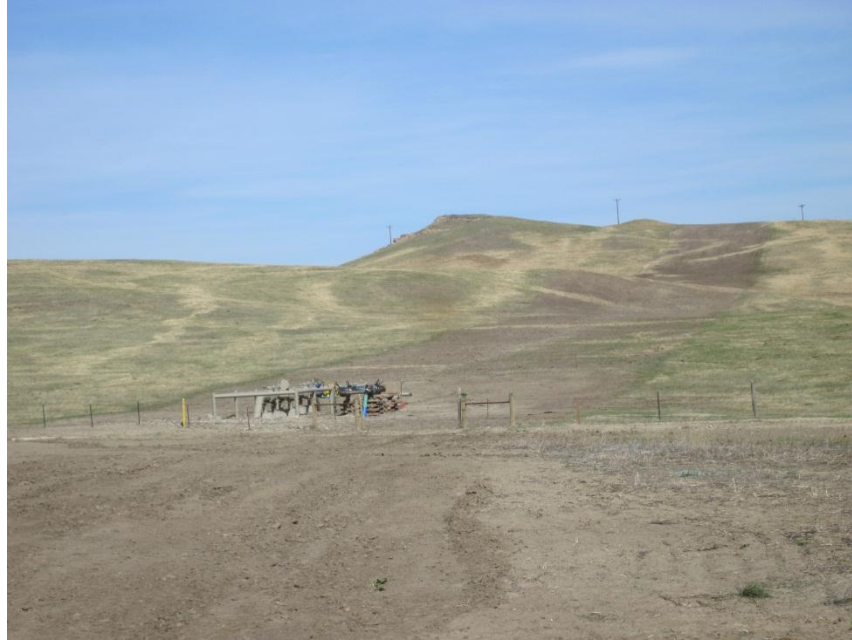
Photo 17. Direction: North. Pipeline right-of-way at the 15 th St. valve setting. Note erosion control structures on the slope.
