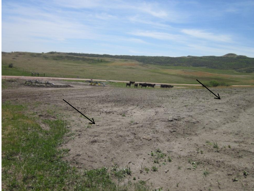
Photo 51. Direction: Southwest. Photo shows erosion control water bar (indicated by arrows) in place at Bridger's 7 th St. valve setting.
