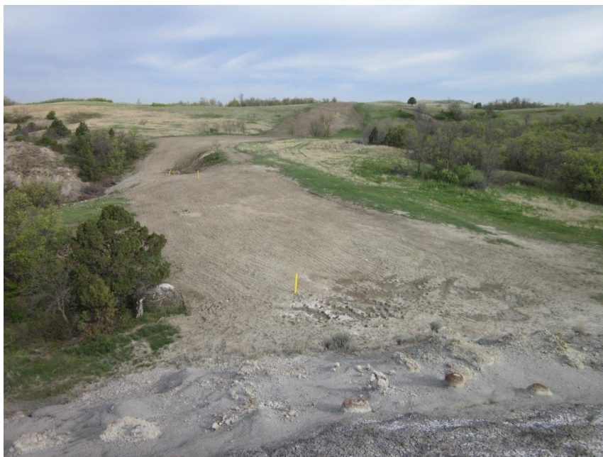
Photo 68. Direction: South. Pipeline right-of-way. Reseeding had occurred, but vegetation had yet to reclaim the area.
