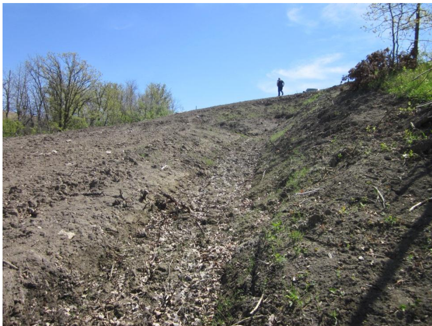
Photo 54. Direction: North. Channel created to prevent erosion. Note some vegetation growing on the slope, which should further stabilize the area. However, this area should be monitored closely to make sure vegetation fully recolonizes the area.
