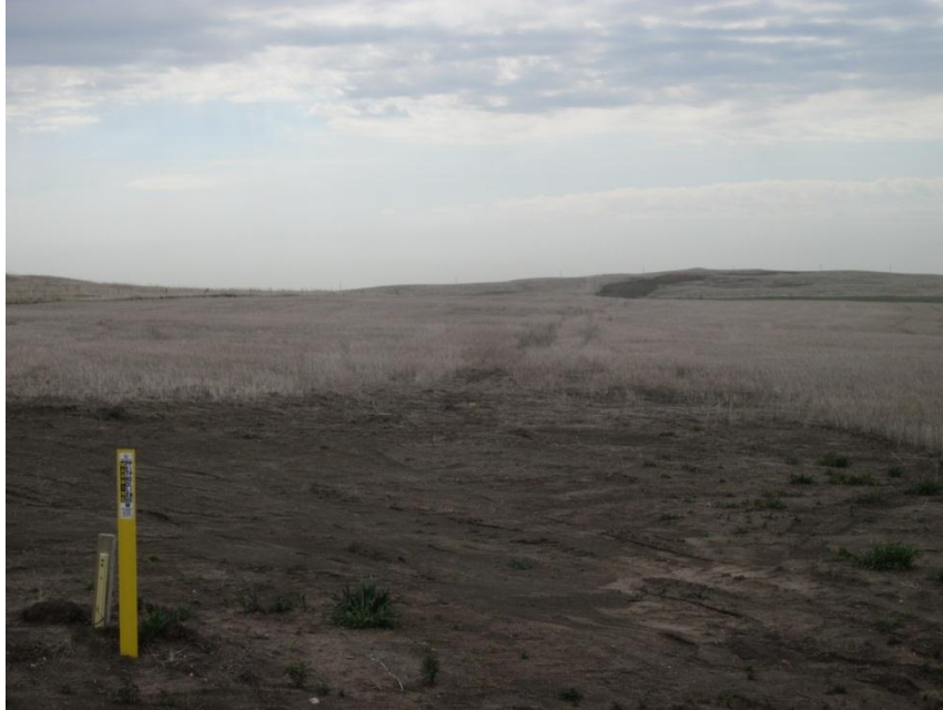
Photo 77. Direction: Southeast. Pipeline right-of-way. Note cathodic tester located in bottom left of photo.
