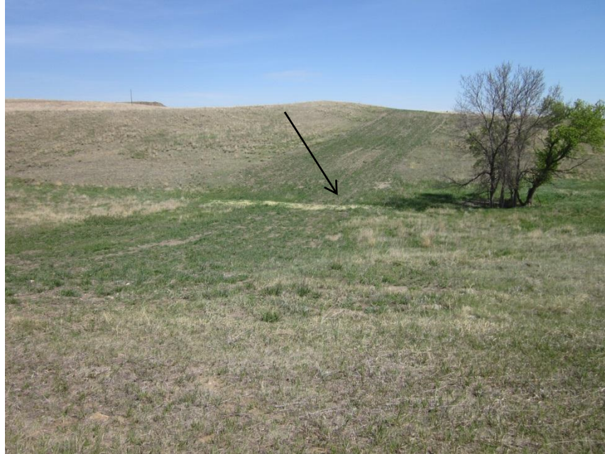
Photo 31. Direction: Northwest. Pipeline right-of-way. Grass mats (indicated by arrow) had been placed for erosion control at the request of landowner. This area was nearly completely reclaimed by vegetation.
