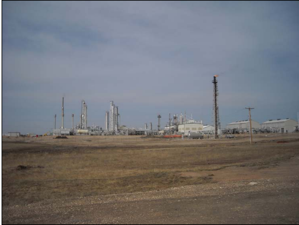
Figure 1. Overview of Hess Corporation Tioga gas plant, facing west. Photographed by J. Cooper on April 7, 2010.
