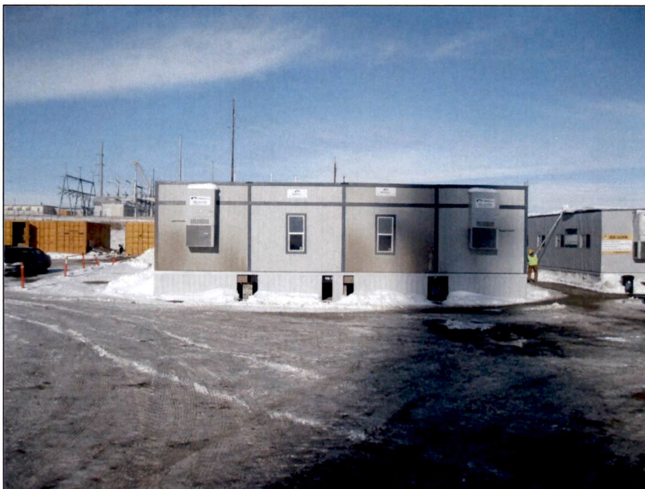
Figure 8. Photo taken facing north near the center of the TGP Expansion. Temporary office buildings set on-site.
