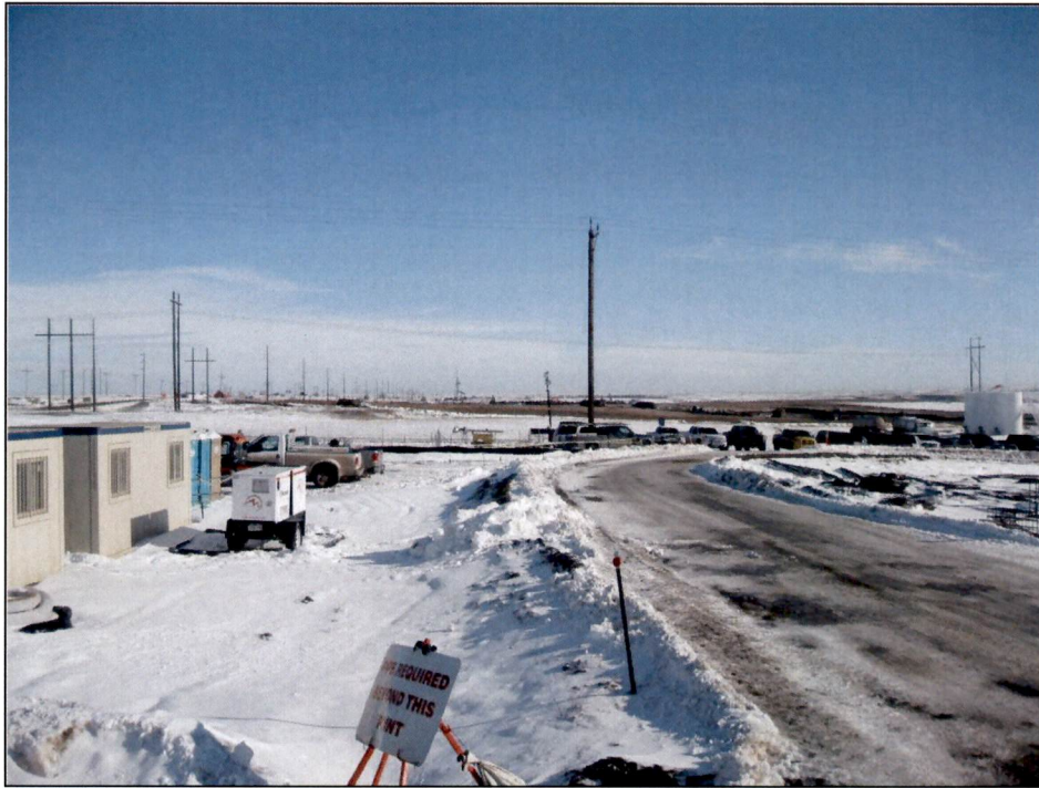
Figure 9. Photo taken facing north near the center of the TGP Expansion. Secondary containment in place under portable generator.
