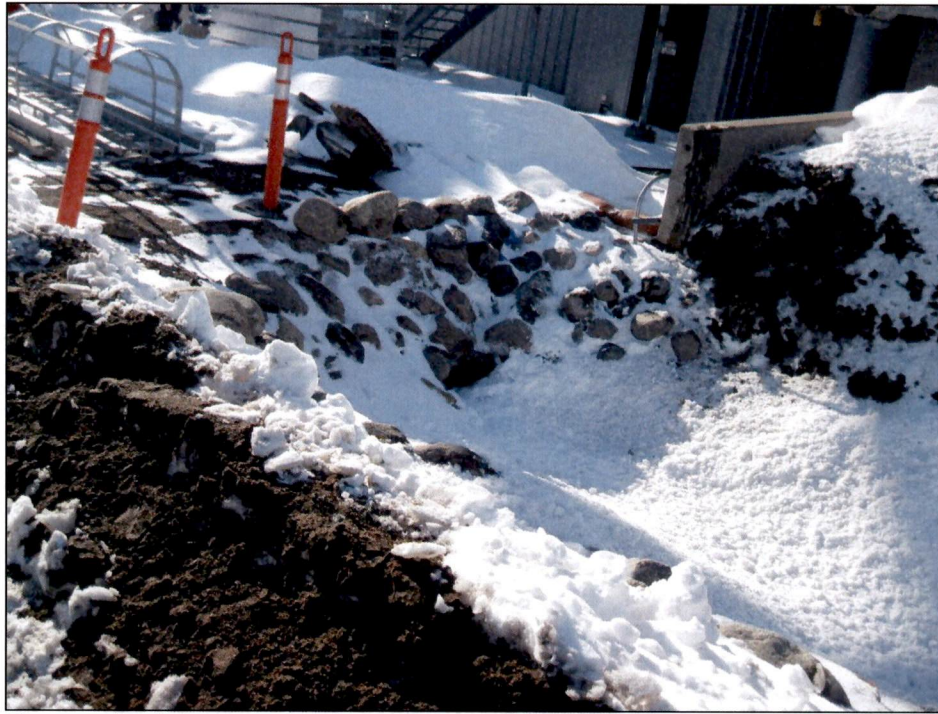
Figure 3. Rock rip-rapped culvert entrance within diversion ditch. Silt fence is also in place in bottom of ditch (currently covered by snow).
