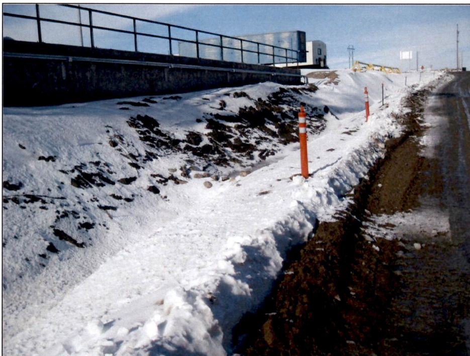
Figure 2. Diversion ditch separating existing site from construction expansion zone. Water is diverted from the existing facility grounds south to containment ponds through ditch. Silt fence and straw wattles are used occasionally in bottom and around culverts.
