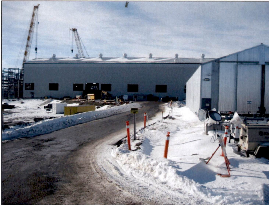
Figure 7. Photo taken facing west near the center of the TGP Expansion. Pictured is access road above tiered construction site. Water diversion ditch to culvert under road currently snow filled (marked by orange pylons).
