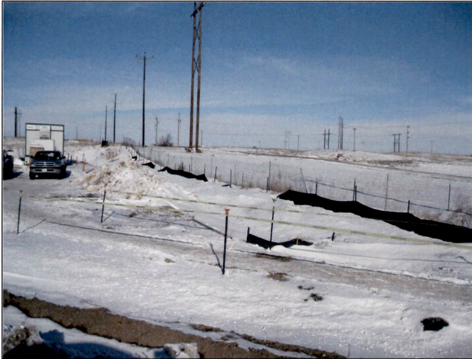
Figure 5. Water diversion ditch on east side of TGP expansion site. Silt fence in place with minor damage from heavy snow. Fencing will be repaired as conditions allow.
