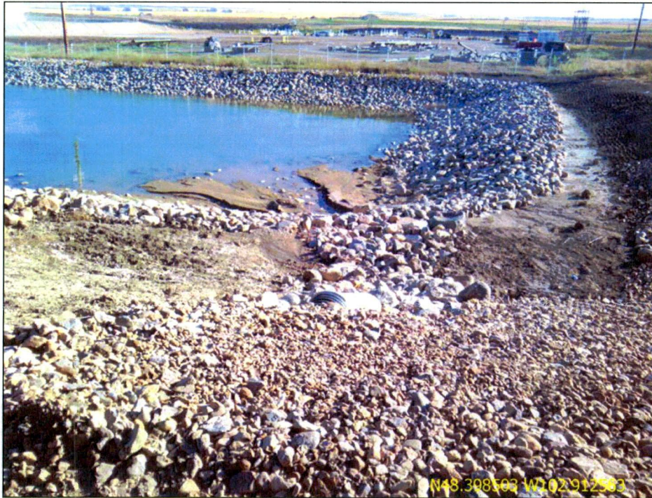
Figure 5. Storm water retention pond is rock rip-rapped with two inlet culverts from the construction site.
