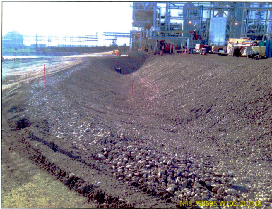
Figure 3. Recently refurbished water conveyance ditch leading directly to the storm water retention. Rock rip-rapped after pipeline (staked) was installed.
