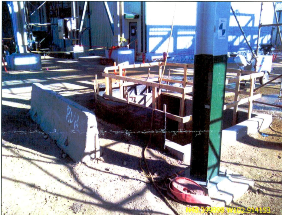
Figure 7. Concrete drain and conveyance being established to permanently direct surface water through the site to the pond.
