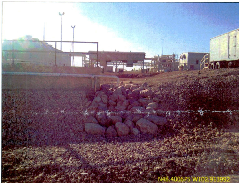
Figure 9. Photo taken facing west of drainage from original plant site. Large rocks placed to dissipate energy of flow water from overland and a downspout of adjacent building.
