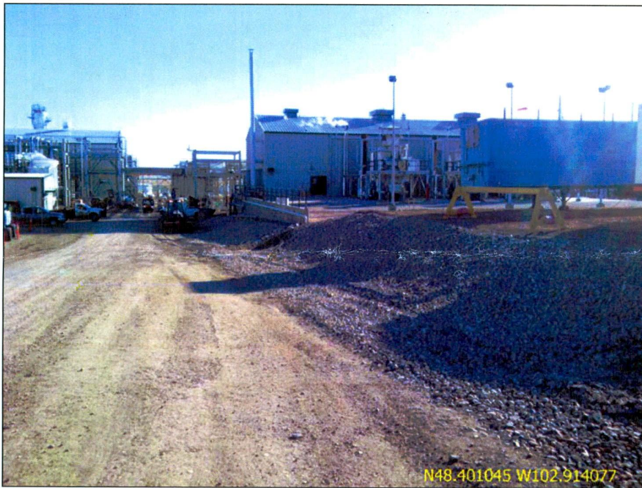
Figure 8. Diversion ditch separating existing site from construction expansion zone. Silt fencing and straw wattles were previously used, but has been stabilized with erosion control matting and rocked.
