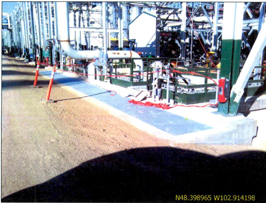
Figure 6. Concrete water collection drain in the interior of the plant site. Concrete conveyances and pipelines direct the water through the site to the pond.
